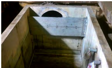
CAM 002A & B inlet structure-baffle is visible in front of CAM 002A outlet with a steel plate (temporary condition) bolted on the left hand wall on the CAM 002B outlet.
