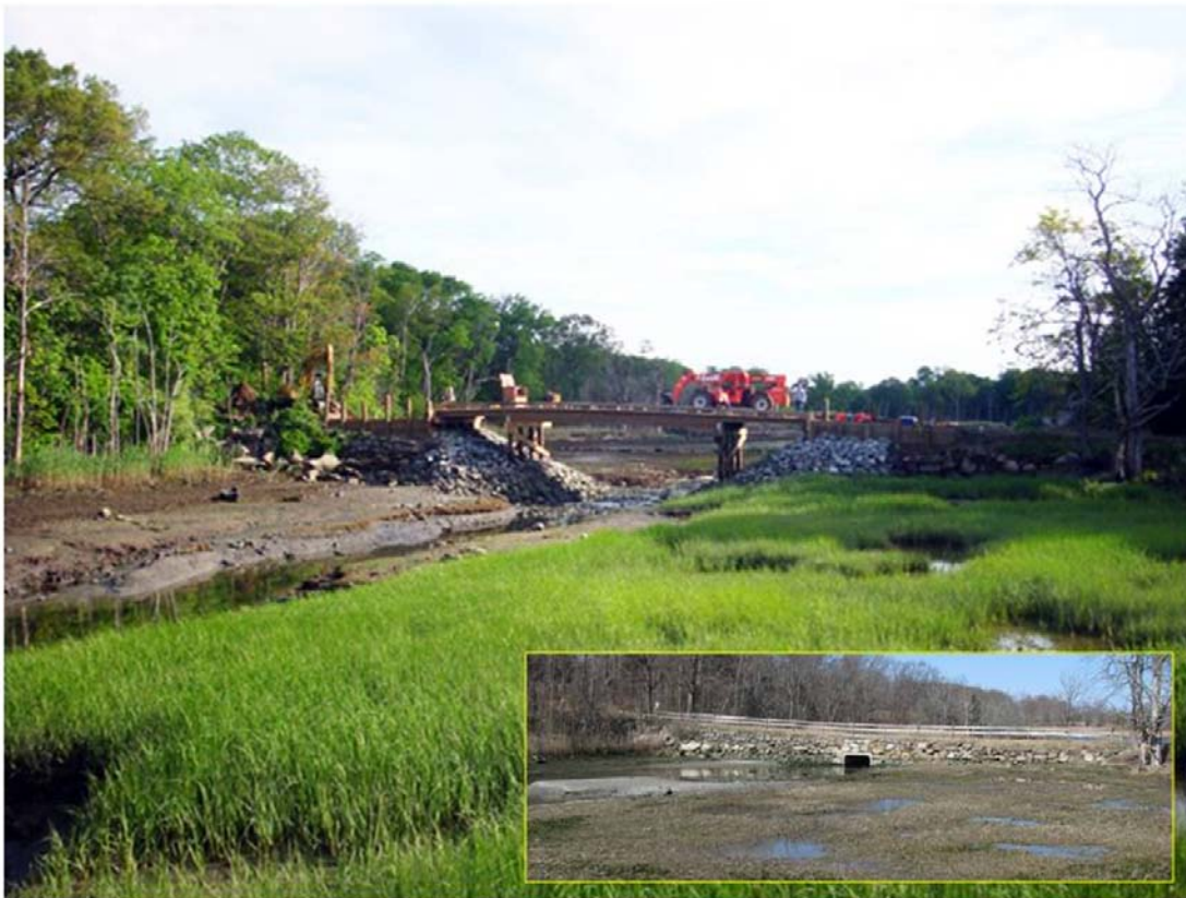
Figure 2- The New Open Span Crossing at Damde Meadows. The pre-Restoration Condition is shown in the inset.
