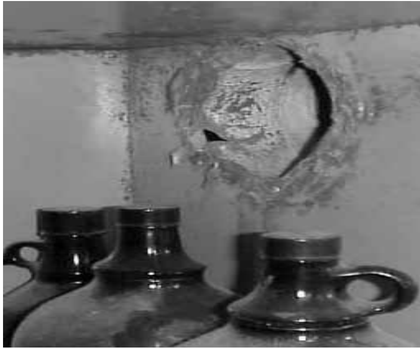
Hole Made By Exhaust Vent Ductwork in Flameproof Cabinet
