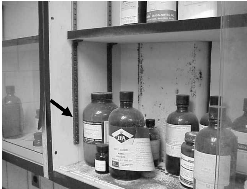
Corroded Classroom Shelves with Stored Chemicals, Note Corrosion on Shelf Supports
