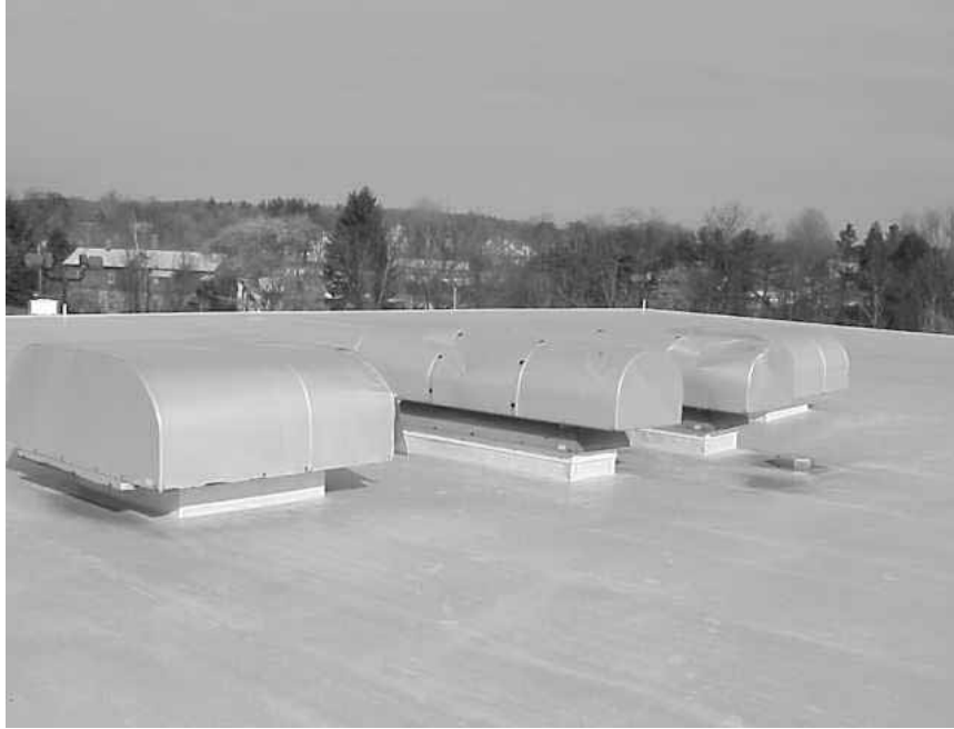
Fresh Air Intakes and Exhaust Vents for B and D Wings.
