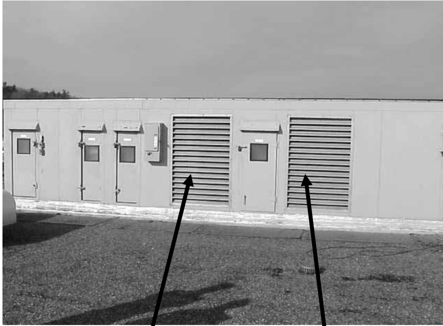
Fresh Air Intake
