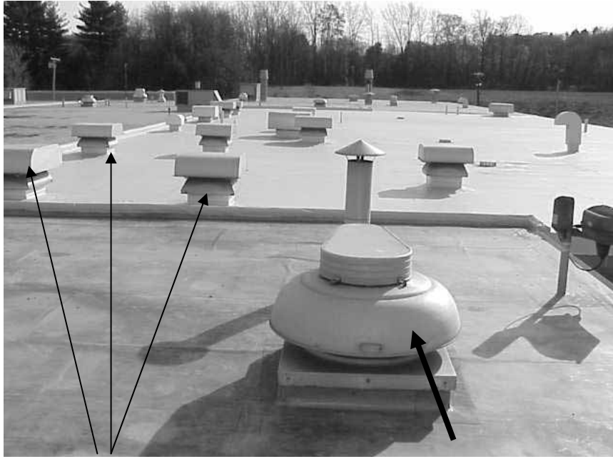
Fresh Air Intakes
