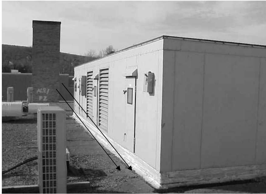
Rooftop AHU Servicing The Internal Classrooms Of The A And C Wing
