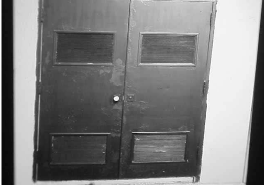
Exterior Door to Mechanical Room Containing AHU for the Art Room (Exterior View) Note Fresh-air Intake Louvers
