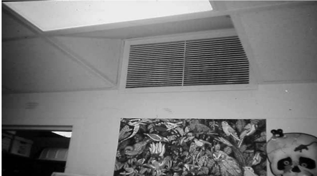
Passive Vent Providing Exhaust Ventilation to Science Classrooms
