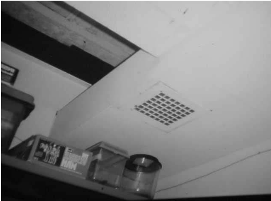
Inactive Ceiling-mounted Exhaust Vent Located in Science Classroom 8 Chemical Storeroom
