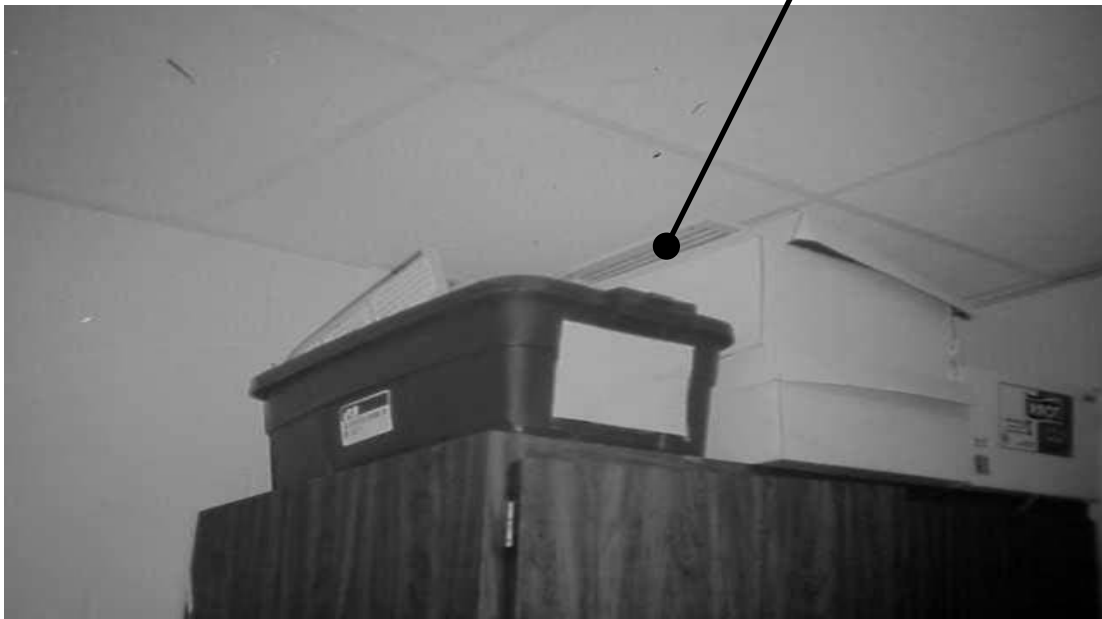
Ceiling-mounted Exhaust Vent Obstructed by Boxes
