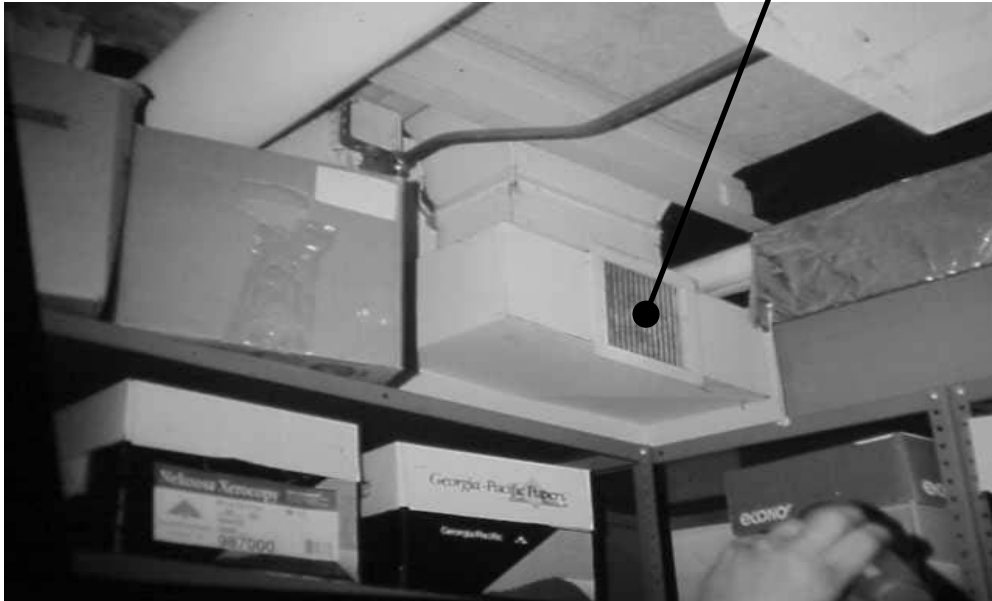
Inactive Ceiling-mounted Exhaust Vent Located in Science Classroom 10 Chemical Storeroom
