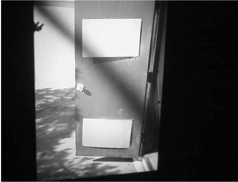
Exterior Door to Mechanical Room Containing AHU for the Art Room (Interior View) Note Fresh-air Intake Louvers are Covered with Sheet Metal
