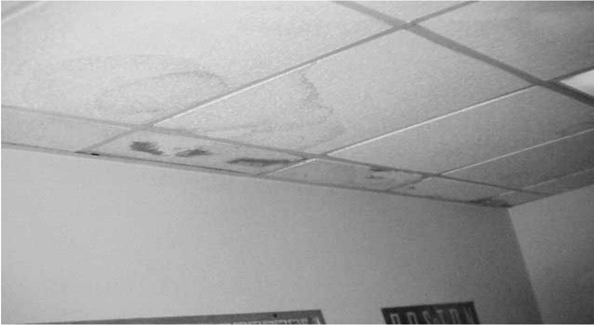
Water-Damaged Ceiling Tiles Noted in Classroom
