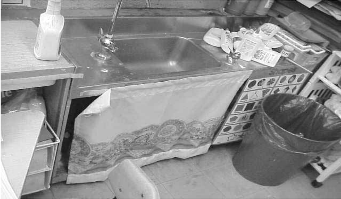
Classroom Cabinet Containing Cleaning Products and Flammable Material Note Missing Door on Cabinet
