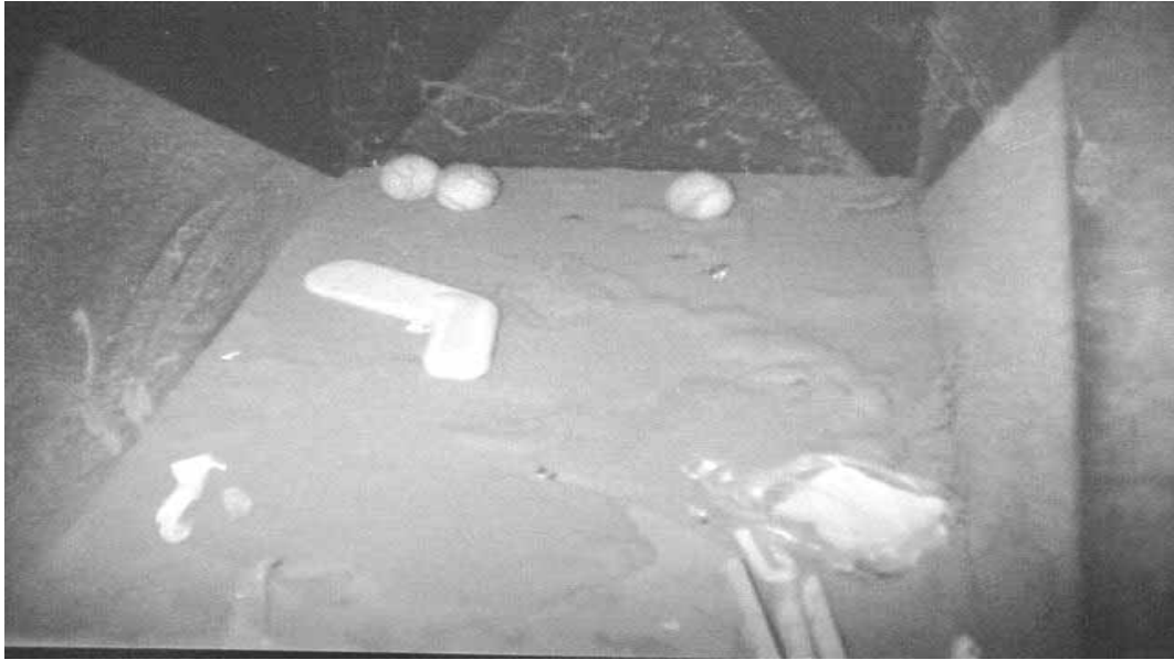
Accumulated Dirt, Dust and Debris Noted in Inactive Gymnasium Exhaust Vent Picture Taken through Damaged Exhaust Grille (see above)
