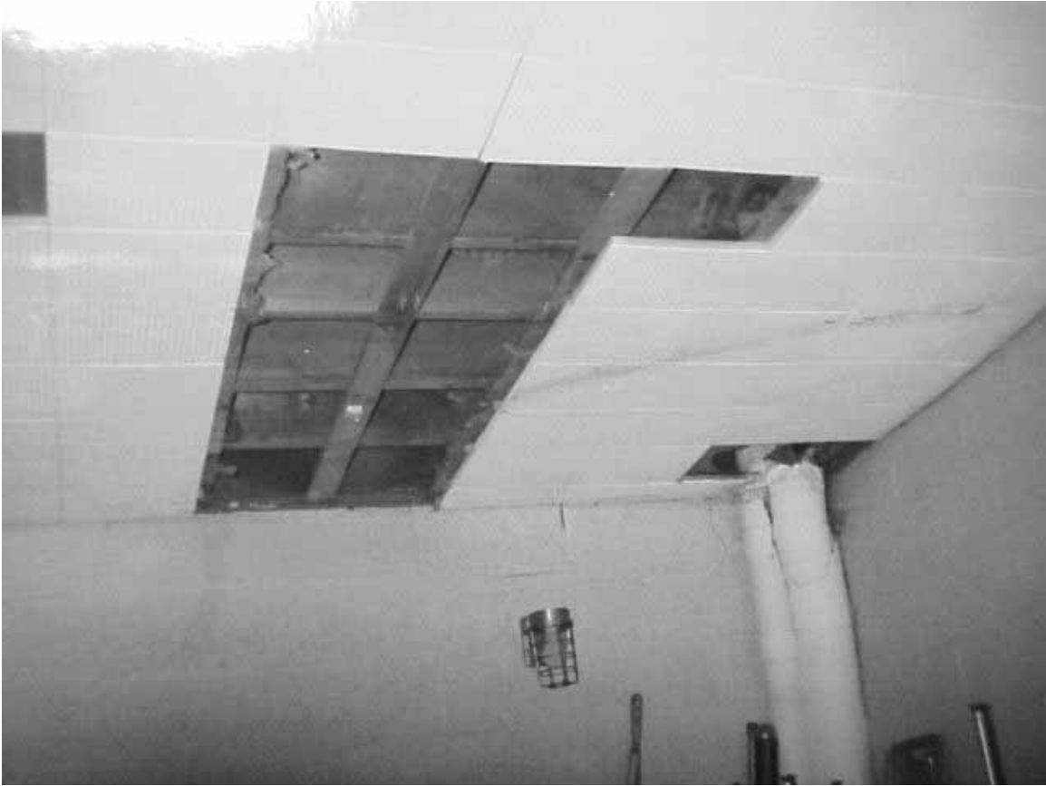
Missing Ceiling Tiles Noted behind Stage in Occupational Therapy Area
