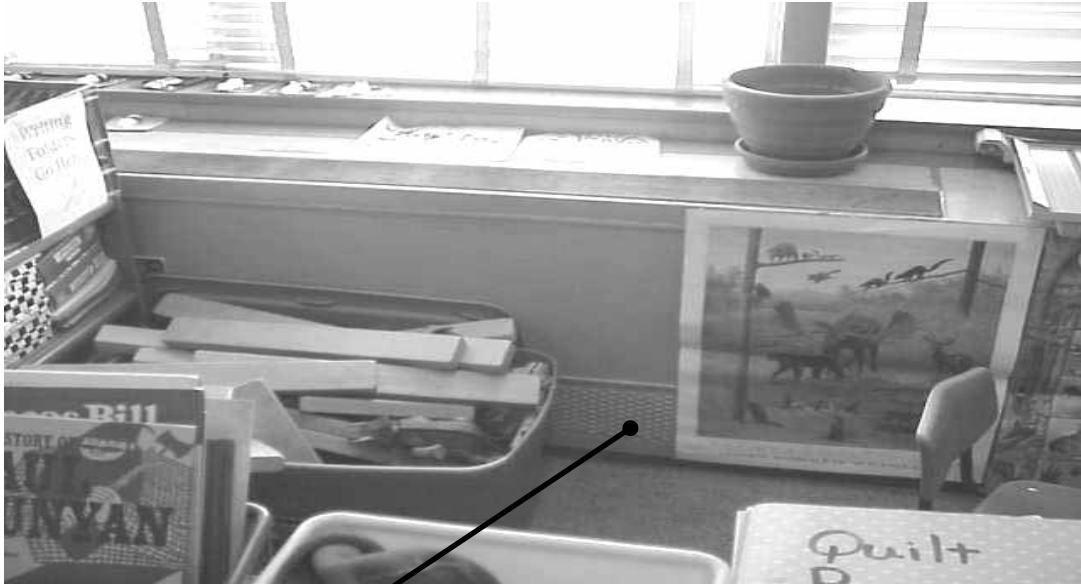
Univent Return Vent Blocked by Storage Bin and Poster
