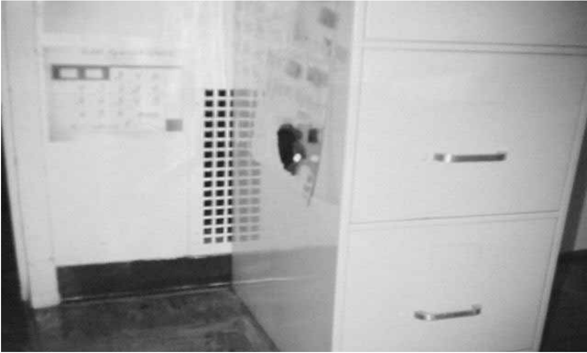
Wall-mounted Exhaust Vent Obstructed by File Cabinet
