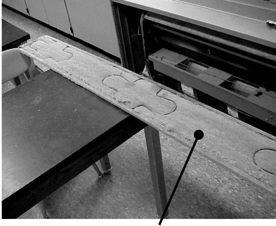
Metal Rack with Replaceable Filter Media
