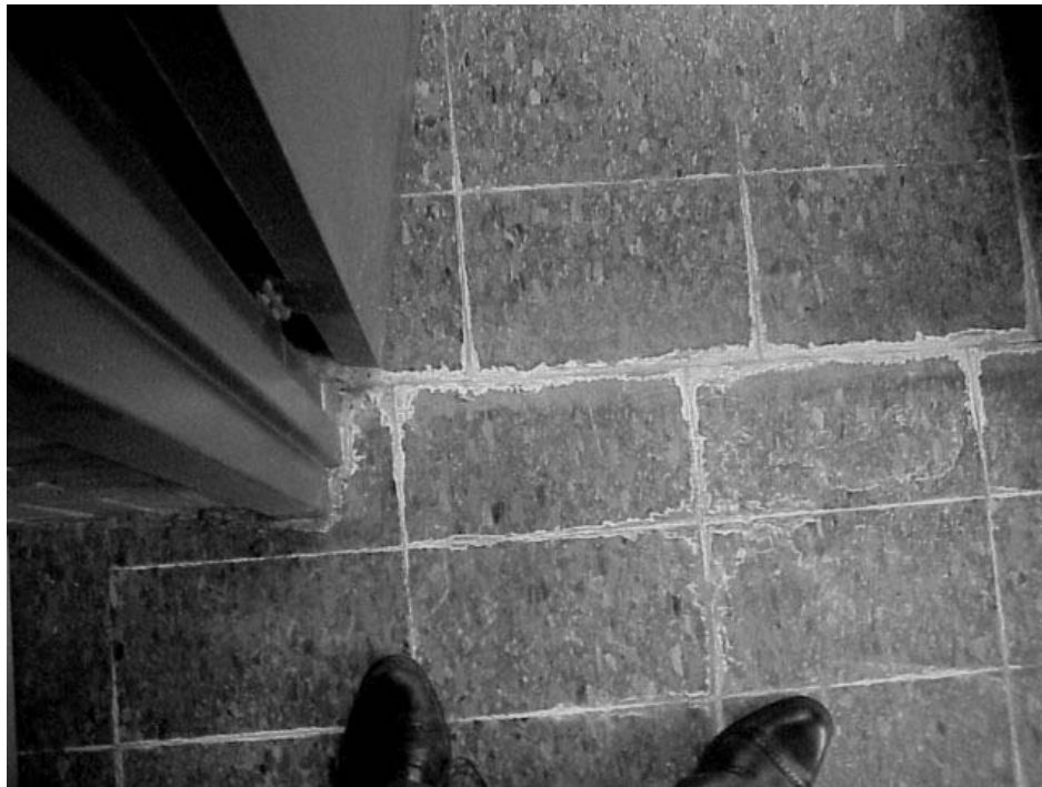
Dried Residue in Cracks of Floor Tiles in the Threshold of Rear Hallway Door of Classroom 108
