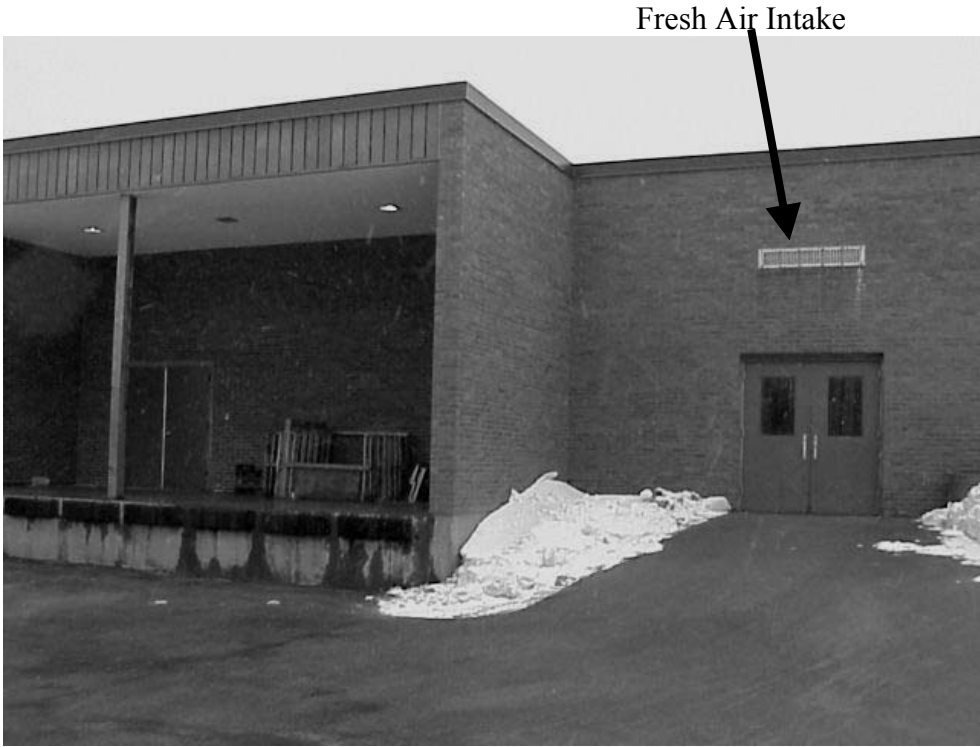
Loading Dock in Close Proximity to Fresh Air Intake
