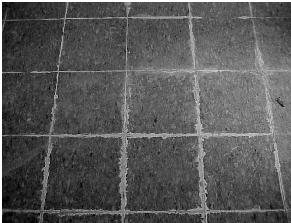
Dried Residue in Cracks of Floor Tiles in the Small Hallway between the Boy's Locker Room and Classroom 108
