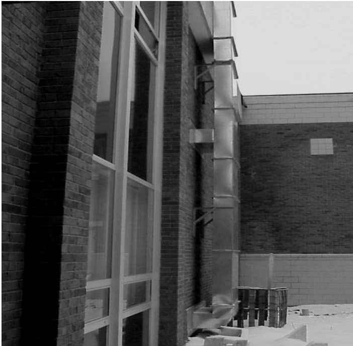
Ground View of Ductwork Installed for Fresh Air Intakes of Classrooms 106, 108, 210 and 212
