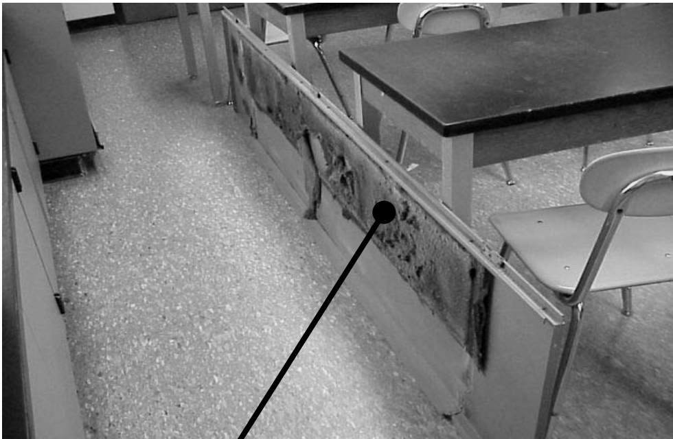
Frayed Fiberglass Insulation on Univent Cover
