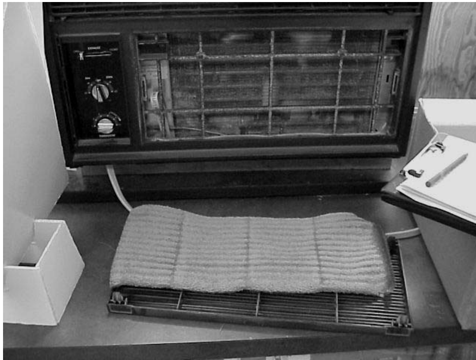
Window-Mounted Air Conditioner, Note Heavy Dust Accumulation on Filter
