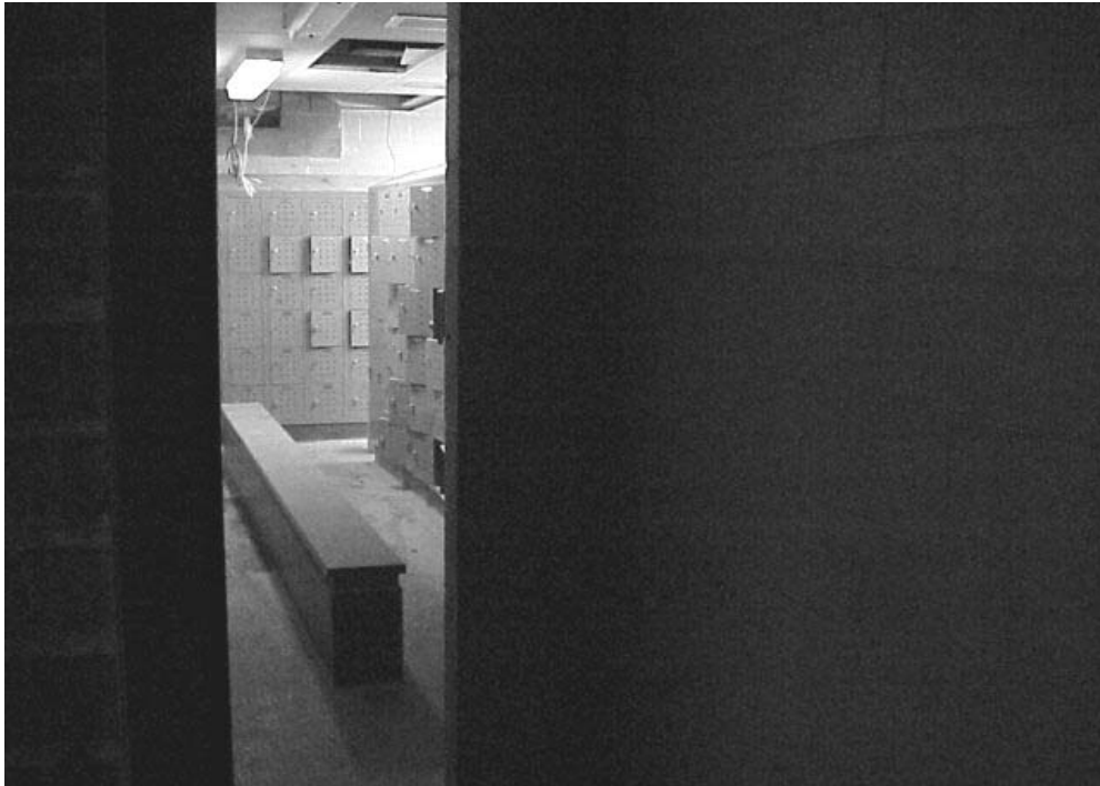
Hallway Door To Locker Room Under Renovation, Note No Containment
