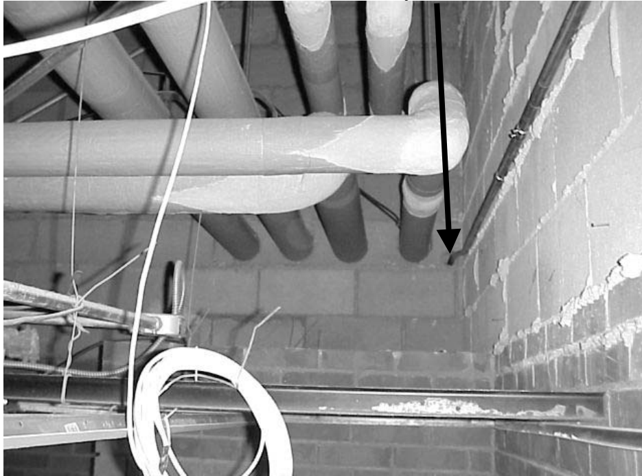
Utility Holes In Wall Through Which Odors May Pass
