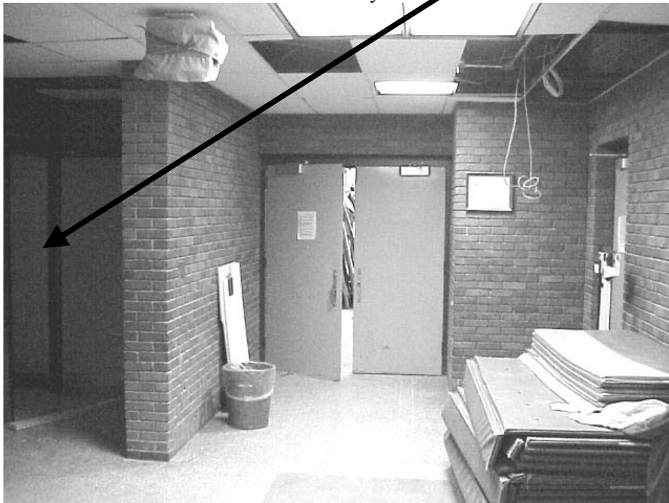
Hallway Door To Gymnasium Under Renovations Left Ajar, Note No Containment
