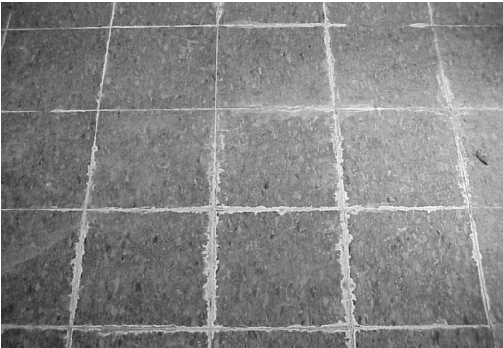
Signs of Dried Moisture in Hallway Floor Tiles near Gymnasium Locker Room
