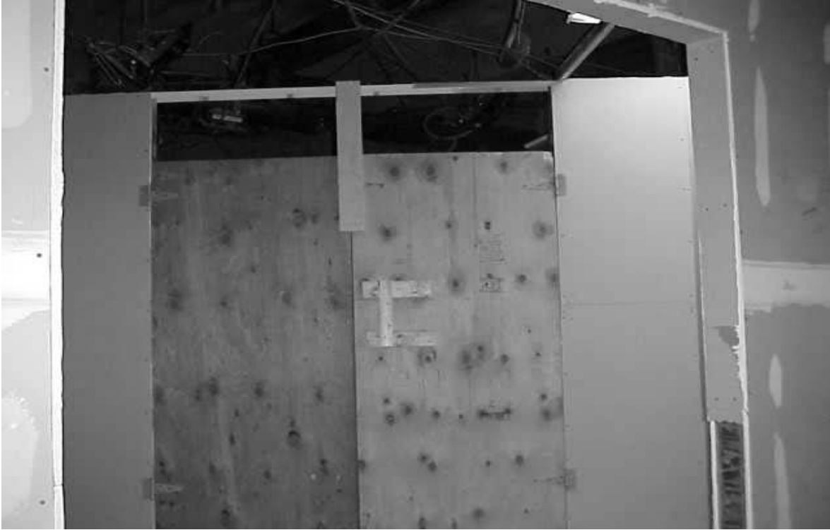
Containment Barrier Separating Construction Zone from Occupied Areas Note Removed Ceiling Tiles and Spaces above Containment Wall
