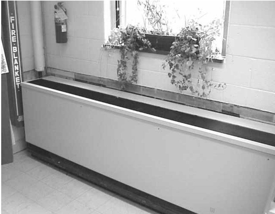
Plants Over Univent Air Diffuser
