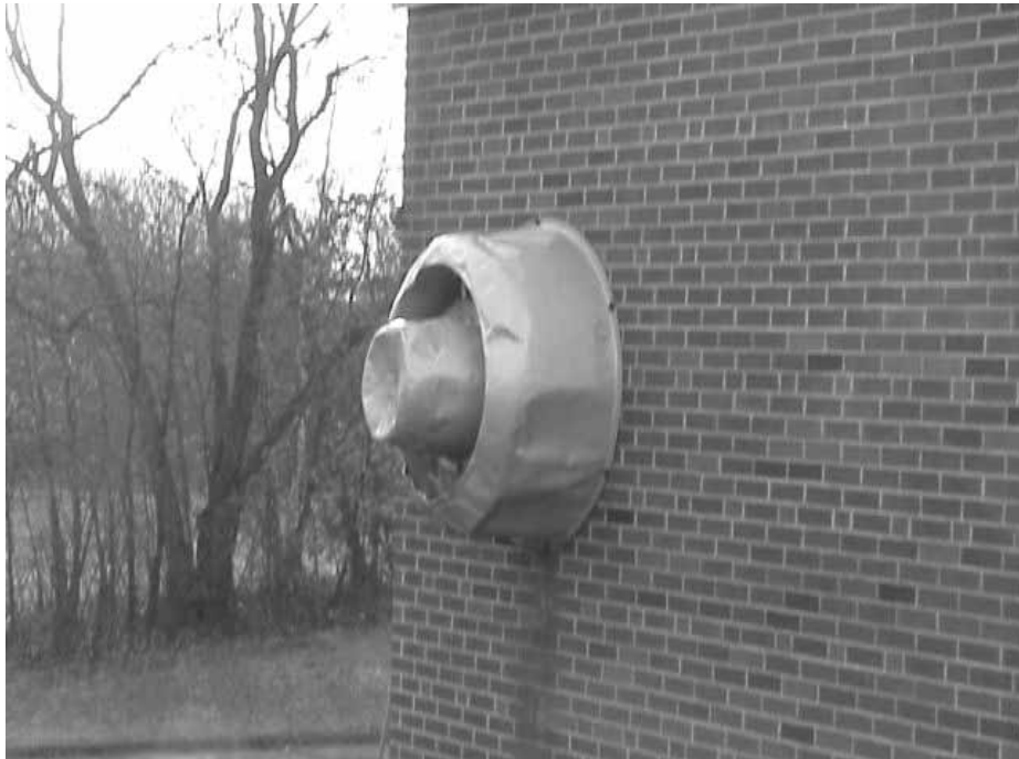
Vandalized Gymnasium Exhaust Vent Cover
