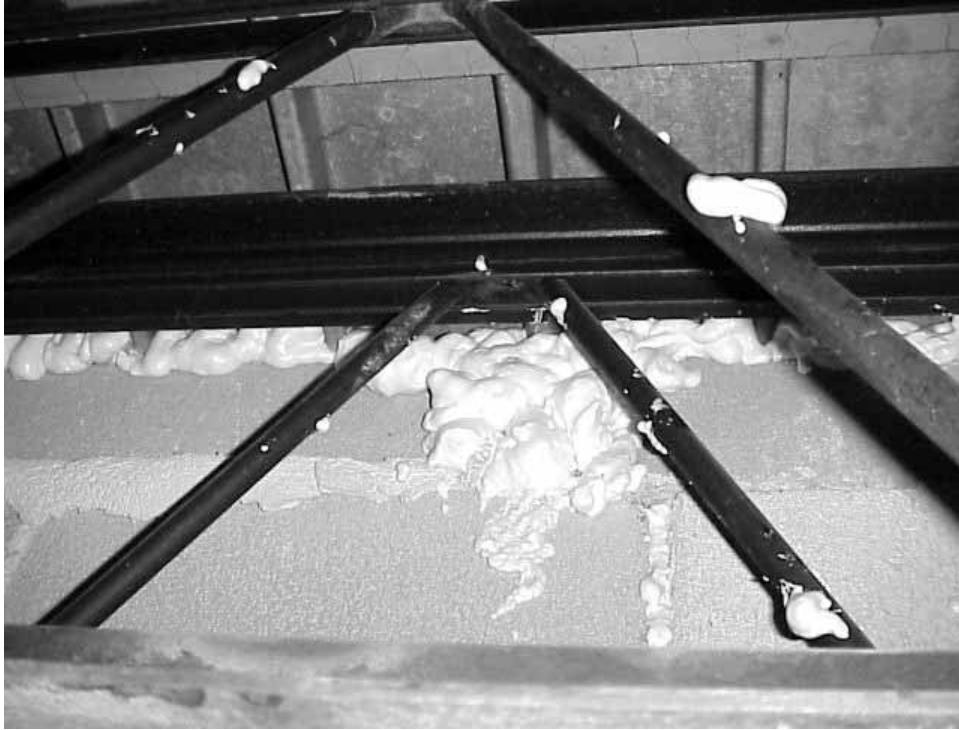
Foam Sealant Applied to Roof Decking/Wall Junction of Shared Wall of Art Room and Boiler Room
