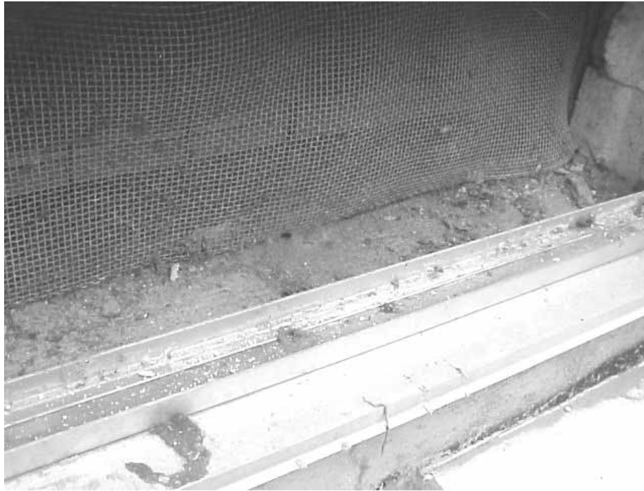
Leaves, Dirt and Other Normal Outdoor Debris behind Fresh Air Intake Louver Of Classroom 6 (Formerly Classroom 15)
