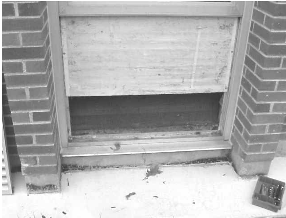
The Fresh Air Intake Grille (See Picture 14) Was Removed From Exterior Of Classroom 6 (Formerly Classroom 15)
