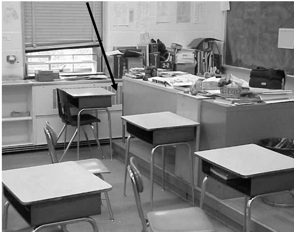
Return Vent of Unit Exhaust Ventilator Blocked with Student Desk
