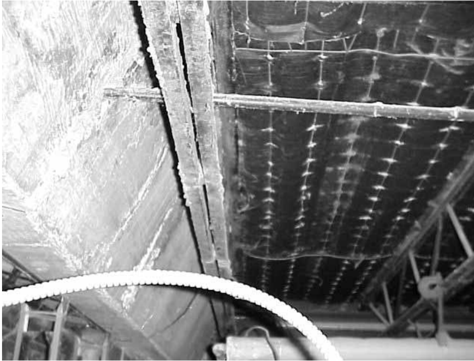
Corrosion of Steel Beams from Water Penetration through Seams around Concrete Platforms
