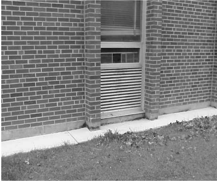
Shrubbery Was Removed From The Fresh Air Intake For Classroom 6 (Formerly Classroom 15)
