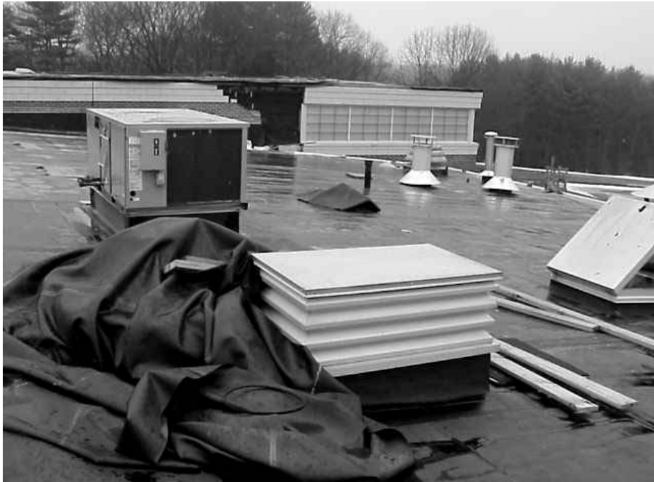
Fresh Air Intake above Kitchen
