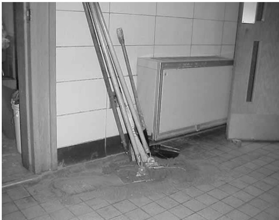
Floor Mops beneath Fan Coil Unit in West Wing
