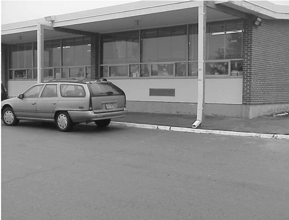
East Wing Fresh Air Intake near Parked Cars
