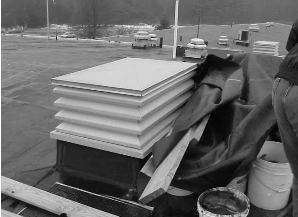
Open Containers of Roofing Materials beneath Tarpaulin next to Rooftop Fresh Air Intake
