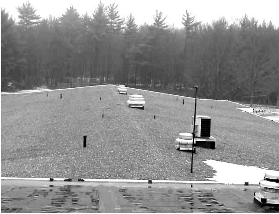
Exhaust Vents Above The West Wing, Note Wet Roof Rock Ballast Around Vents
