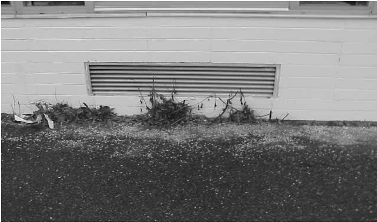
Plants Growing in the Exterior Wall/Tarmac Junction outside Classrooms 7-10
