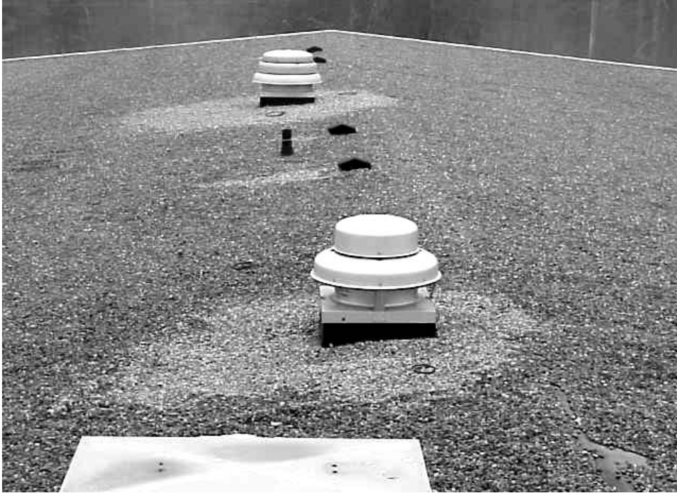
Exhaust Vents above the Eastern Wing, Note Dry Roof Rock Ballast Dried By Exhaust Air from These Vents
