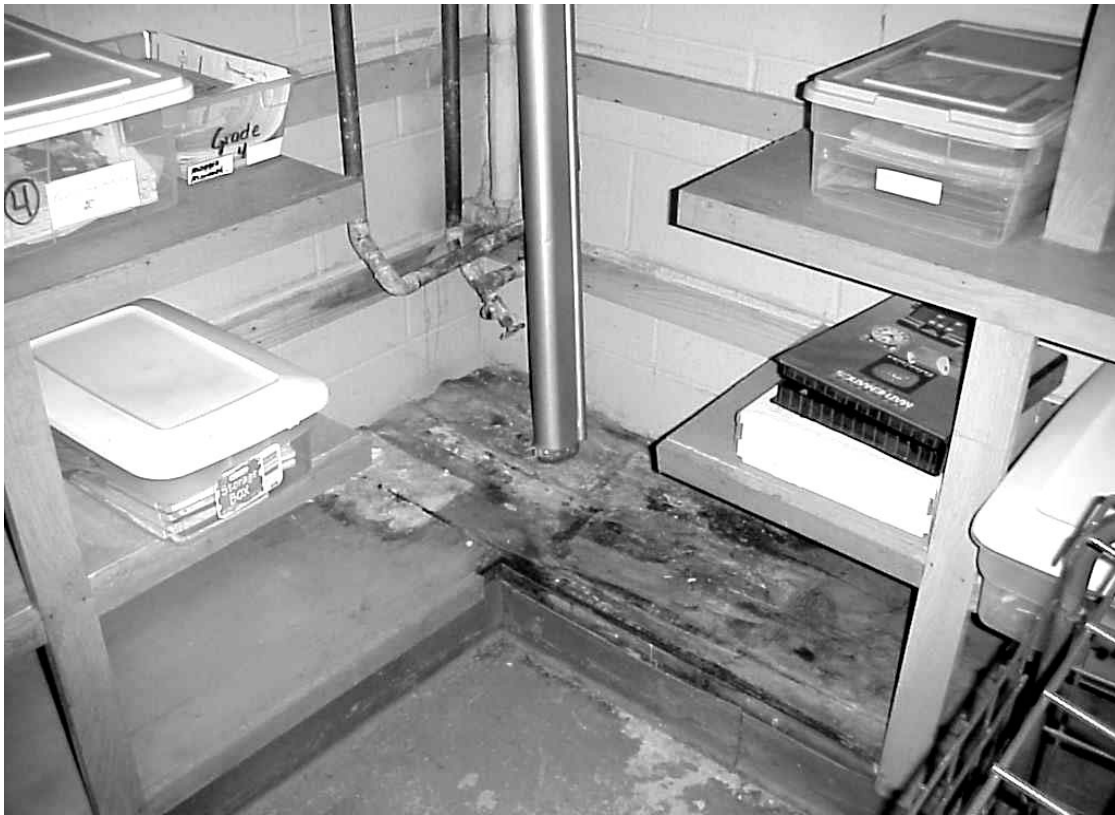
Mold Colonized Wood Shelves in Book Storeroom near Boy's Restroom in West Wing
