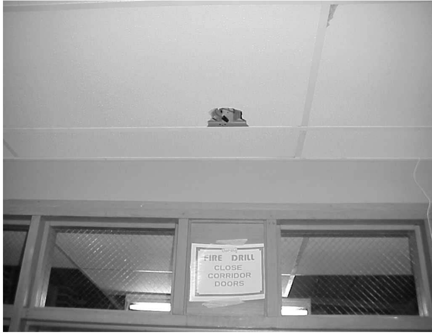
Close-up of Hole In Ceiling System in Picture 1
