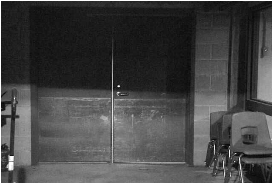
Double Doors Leading to Dumpster Room Note Spaces between and beneath Doors
