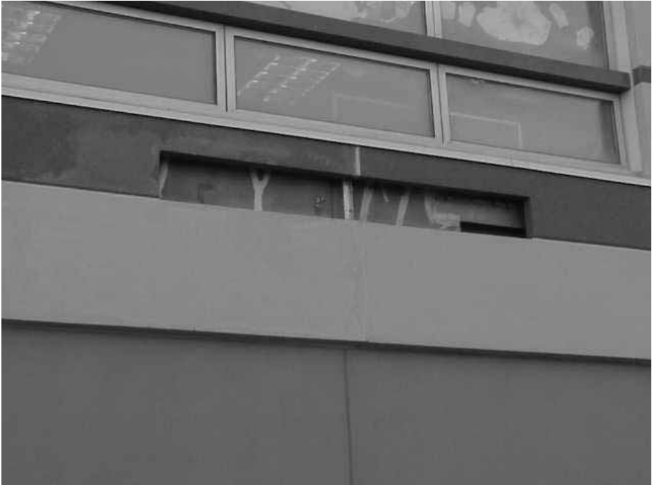
Exterior Wall Sealing over Fifty Percent of a Classroom Univent Fresh Air Intake Vents
