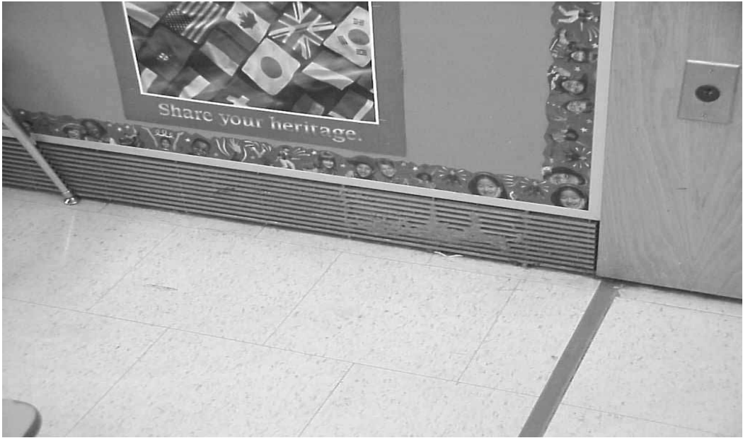
Exhaust Vent Located at Floor Level in Classroom
