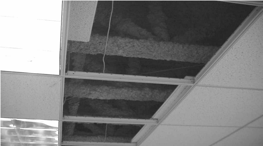
Missing Ceiling Tiles
