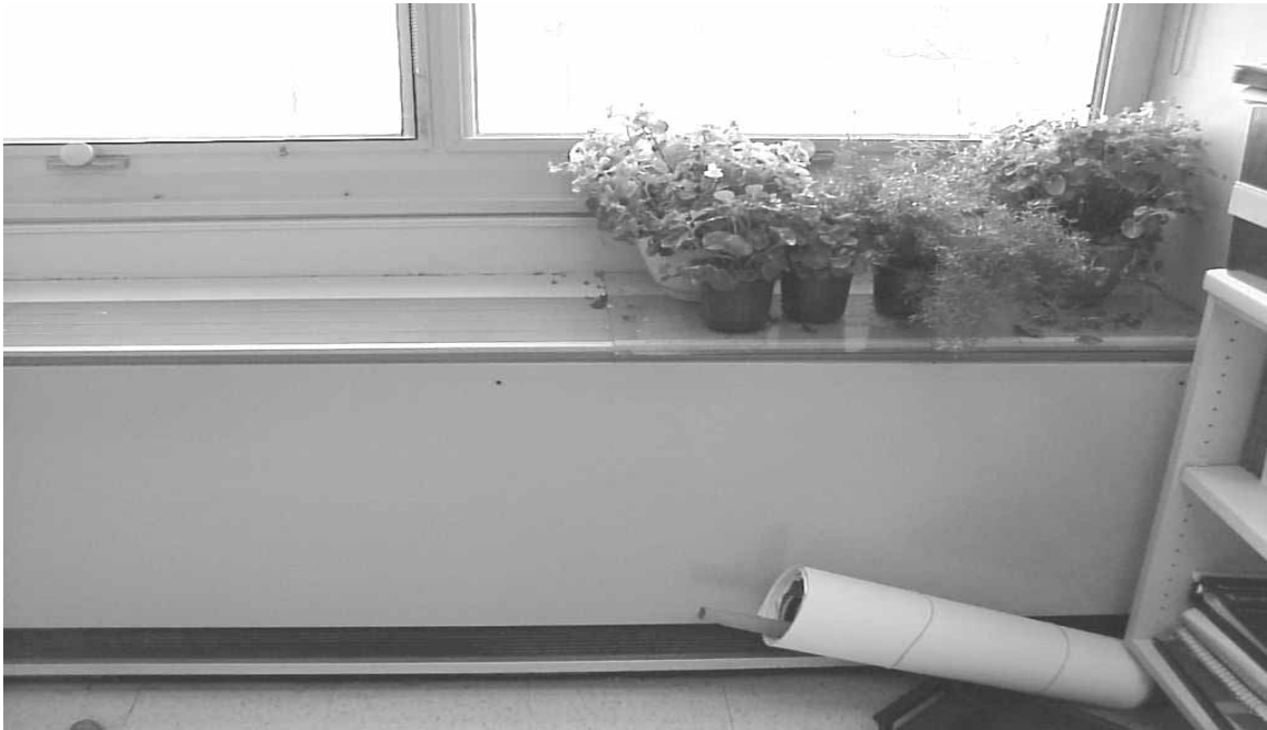
Plants Noted on Classroom Univent Air Diffuser
