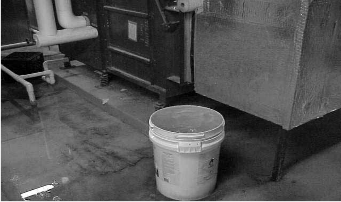
Bucket Stationed below Leak in HVAC Penthouse Note Overflow on Floor
