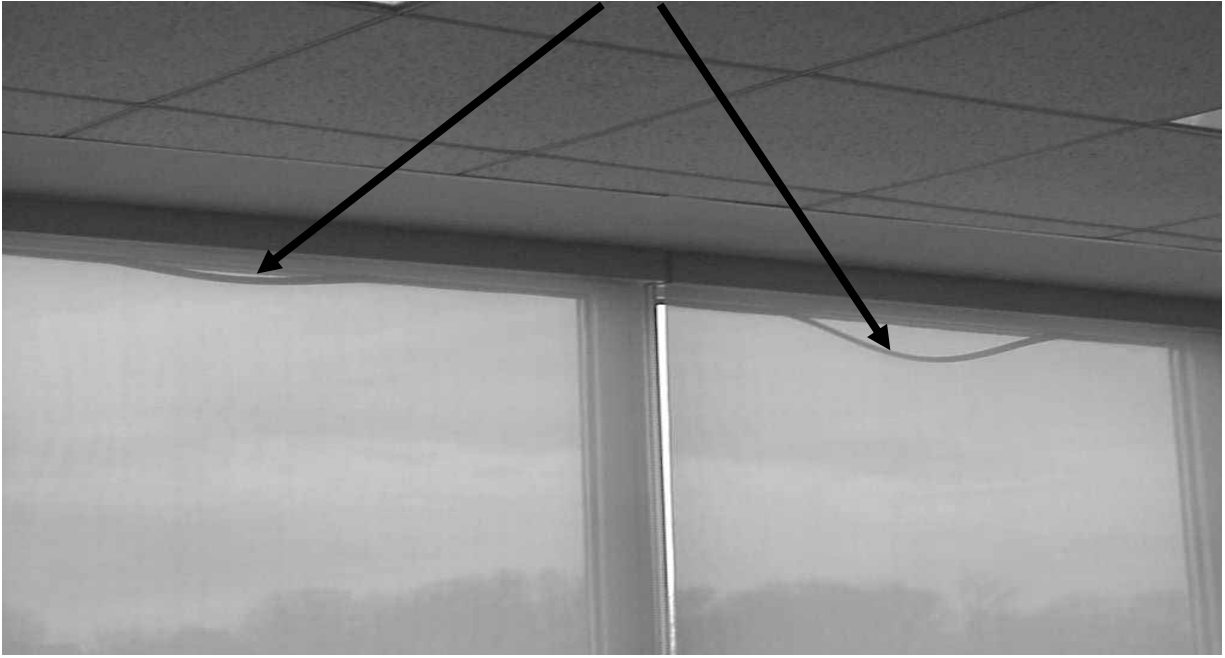
Failing Caulking Noted around Classroom Window
