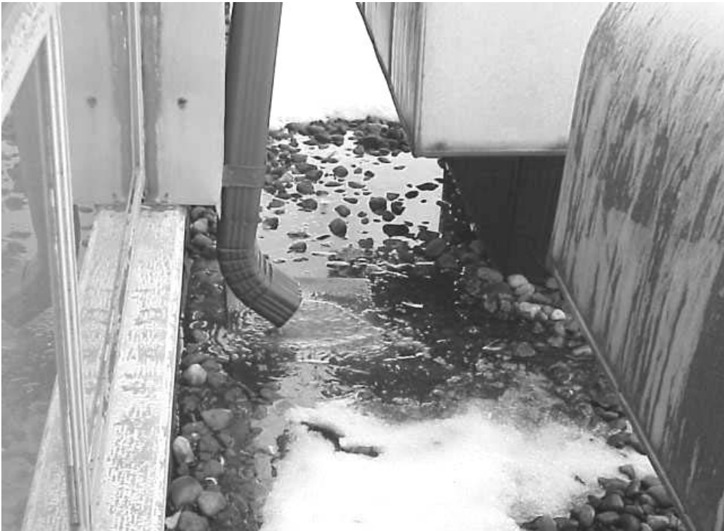
Water Accumulation on Roof
