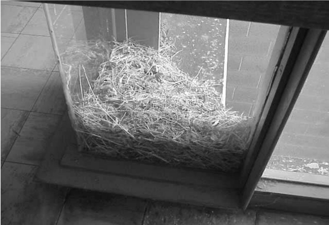
Bird Nest (taken from inside building) On Front Ledge of Second Floor
