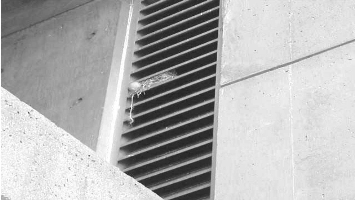
Bird Nest in Air Intake Vent
