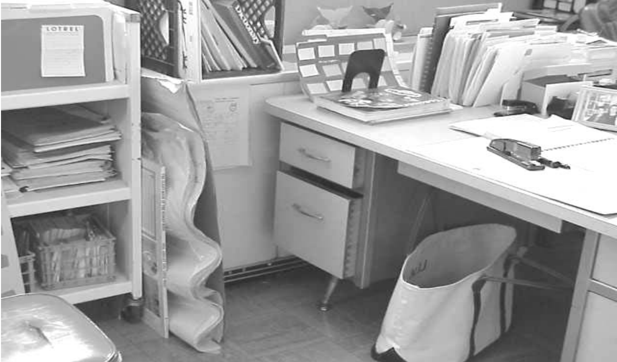
Univent Return Vent Obstructed by Desk
