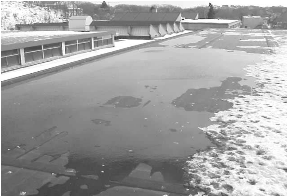
Water Pooling on Roof
