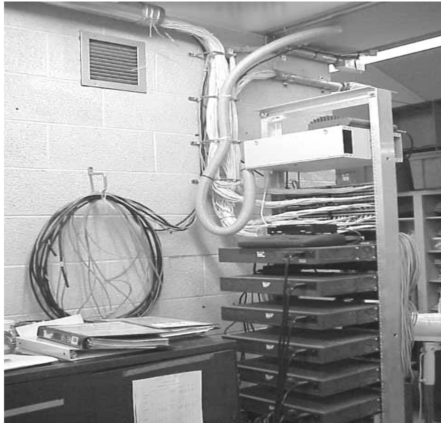
Computer Main Frame Located beneath Inactive Exhaust Vent in Reading Room 233
