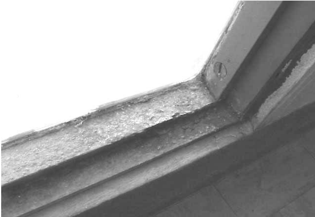
Water Damaged Window Frame
