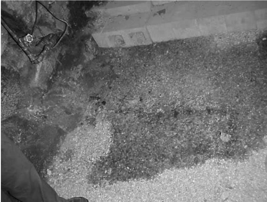
Standing Water in Basement
