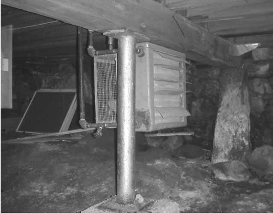
Fan Heating Unit in Basement
