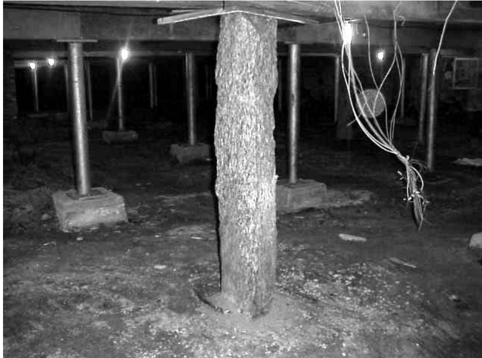
Granite Floor Support Pillar, Note Steel Tube Floor Supports in Background That Indicate Renovations
