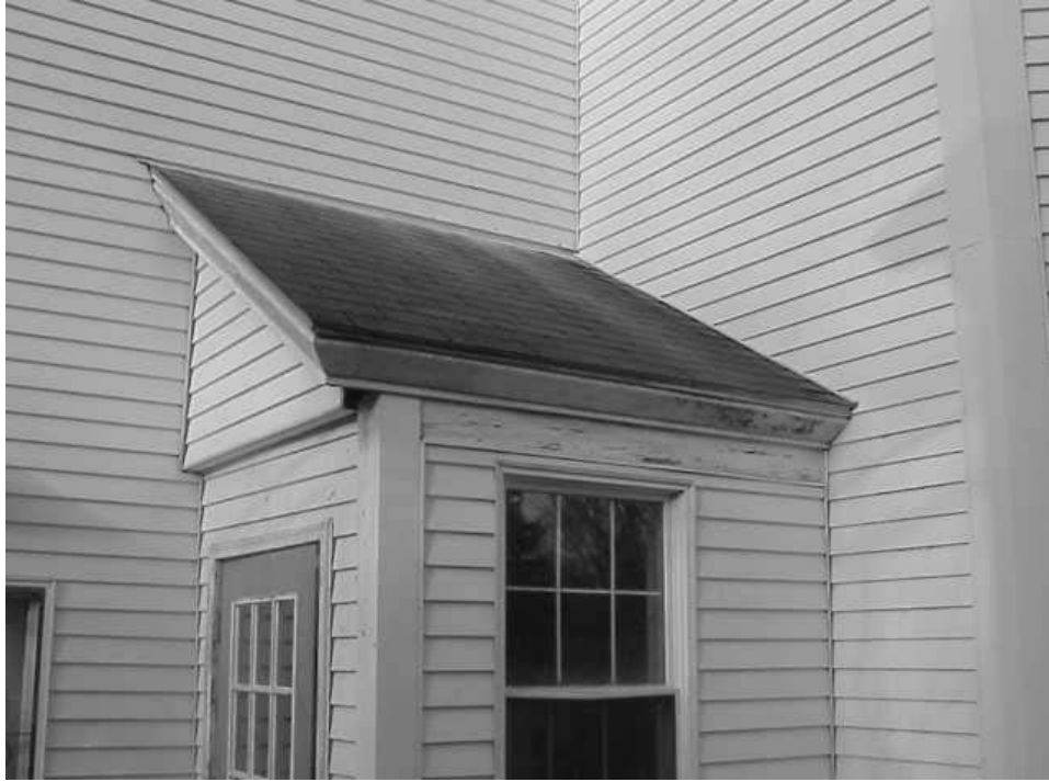
Wall/Roof Junction above Stairwell Water Damaged Plaster
