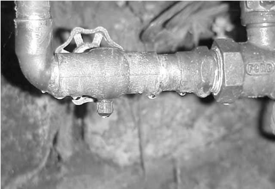
Condensation on Water Pipes
