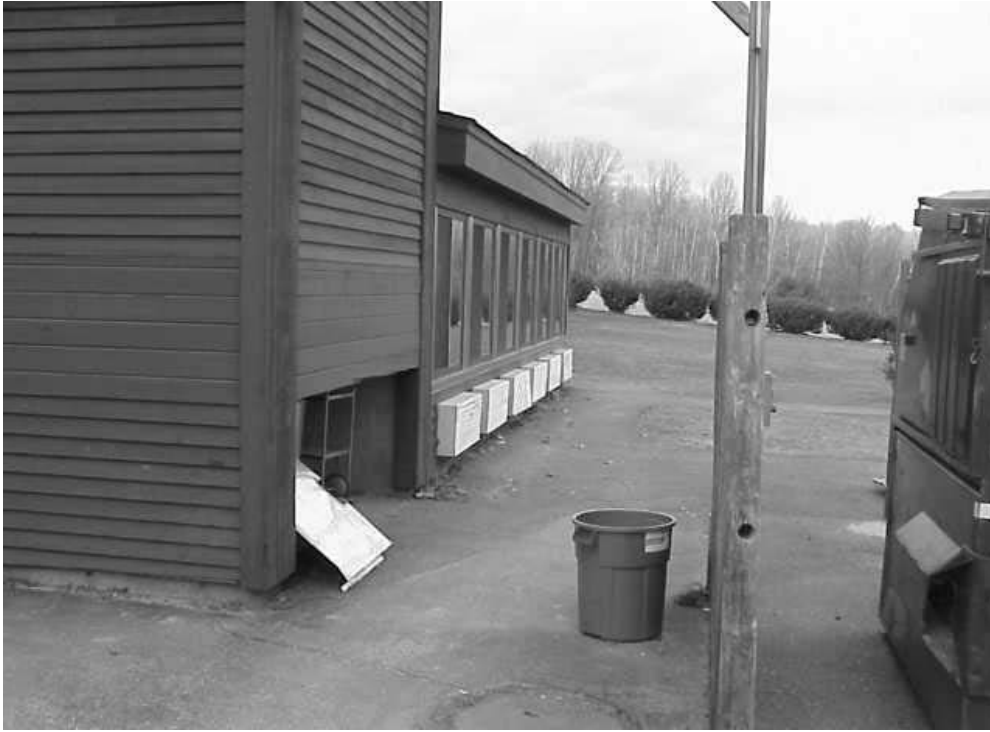
Outer Cafeteria Fresh Air Intakes
