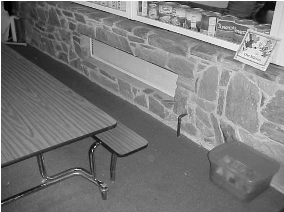
Kitchen/Cafeteria Univent Fresh Air Supply Vent Sealed Indoor by Outer Cafeteria, Note Stone of Former Exterior Wall
