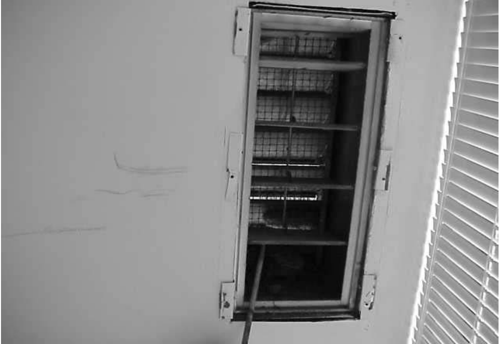
Exhaust Vent with Louvers Fully Opened
