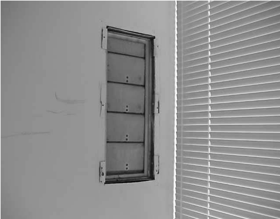
Louvered Exhaust Vent with Grille Cover Removed
