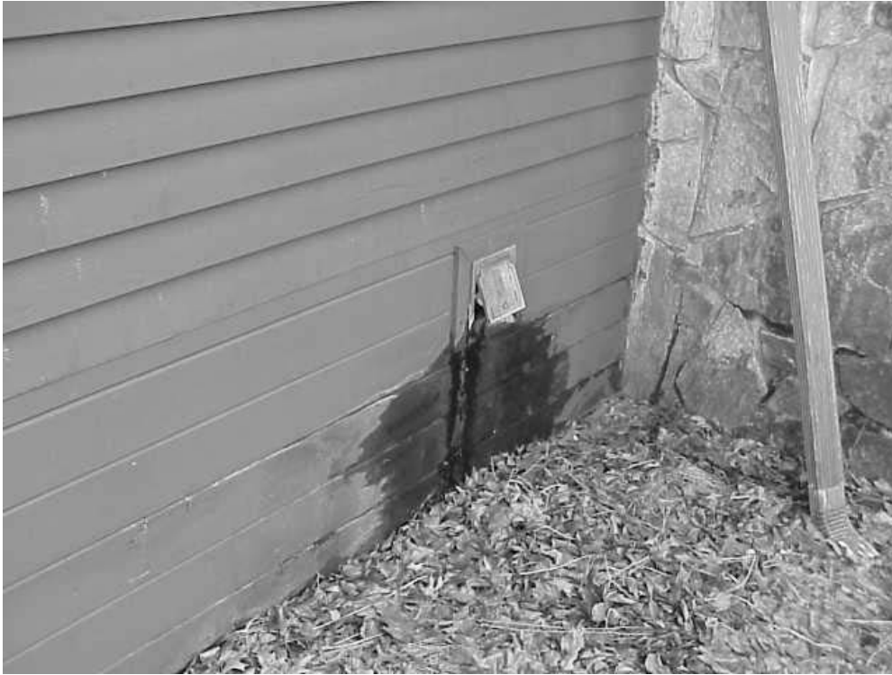
Exterior Wall Water Damaged by Dripping Spigot
