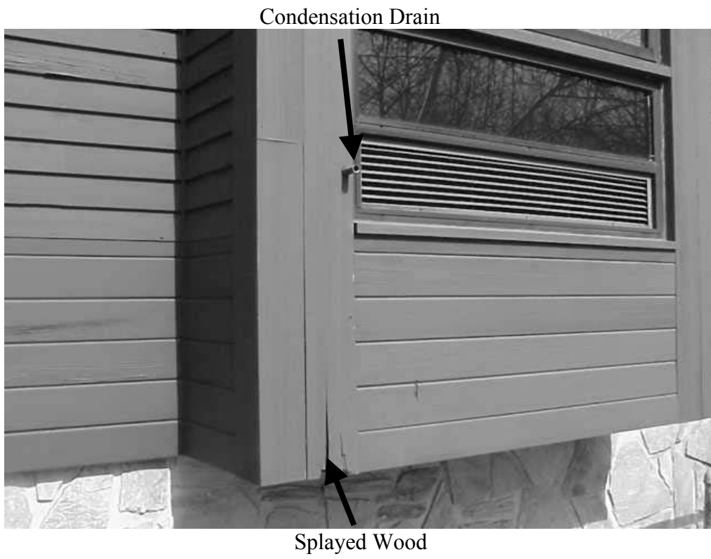
Condensation Drain, Note Splayed Wood Immediately below Drain
