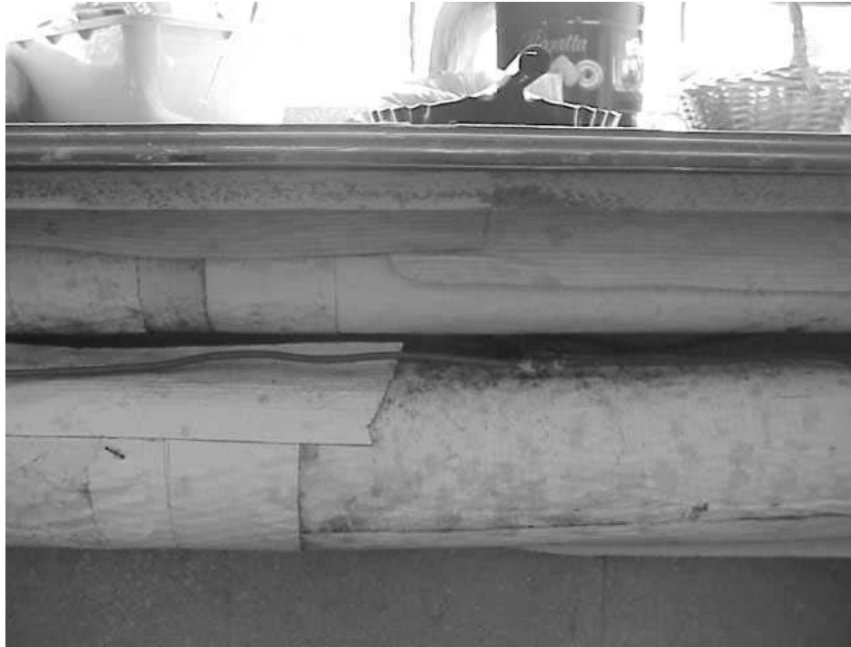
Insulated pipes in Wooden Univent Cabinet, Note Stains/Possible Mold Growth
