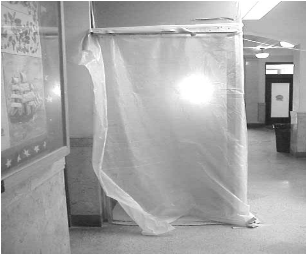
Unsecured Containment Barrier around Restroom Renovations Note the Only Means of Egress is through This Barrier
