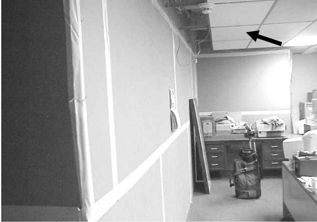
Missing Ceiling Tiles Noted in Office Area Adjacent to the Construction Zone
