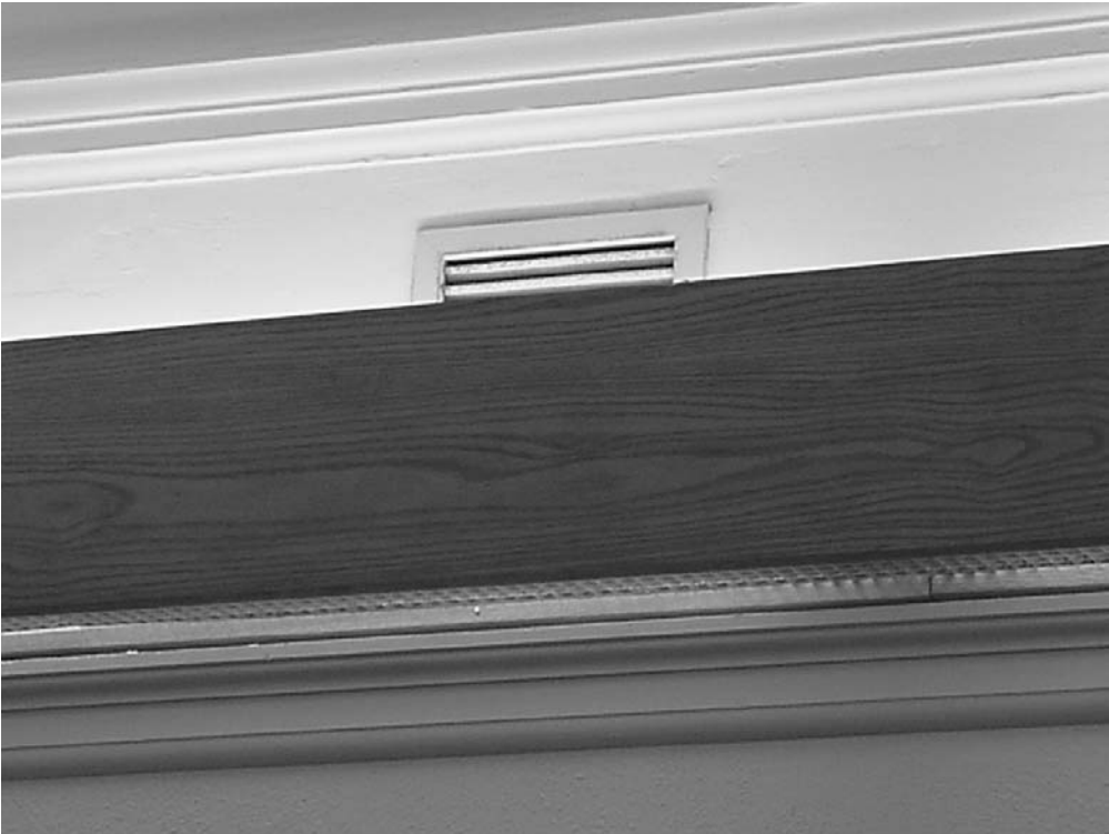
Exhaust Vent behind Wood Molding
