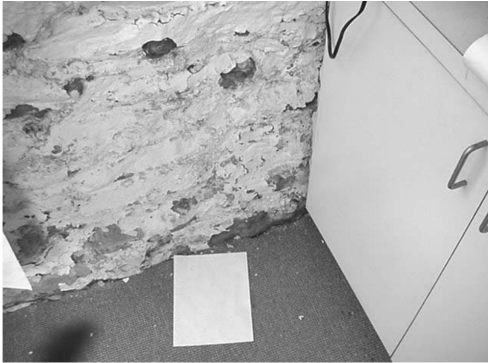
Water Intrusion and Powdered Brick on Carpeting, Note the Proximity of Carpet to Wall
