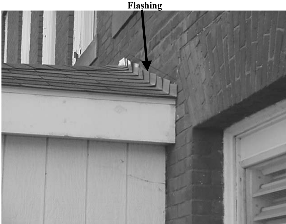
Roof Flashing Laying Flush on Exterior Brick of North Wall
