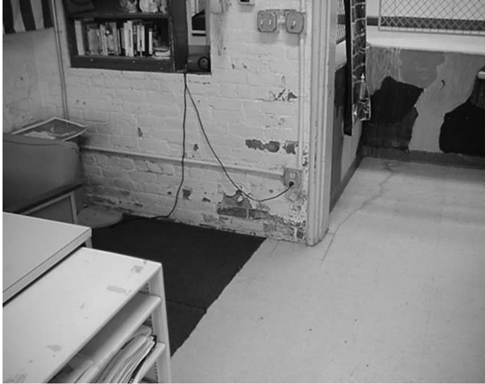
Carpet in Close Proximity to Interior Wall with Signs of Water Intrusion in Art Room
