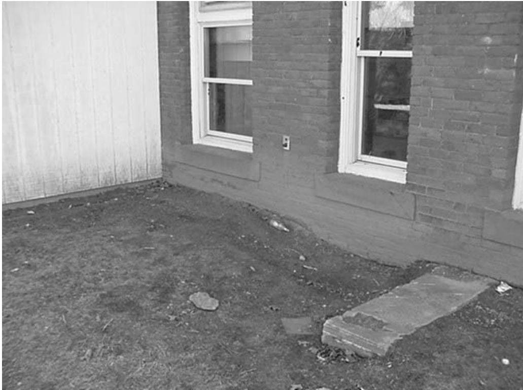
North Wall of North Wing with Mud Spattering and Discoloration, Note the Trough in Soil against the Wall
