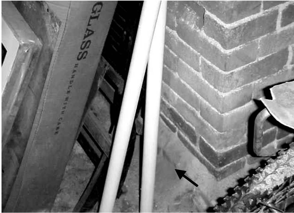
Crumbled Brick and Dust on the Outside of an Exhaust Vent Shaft
