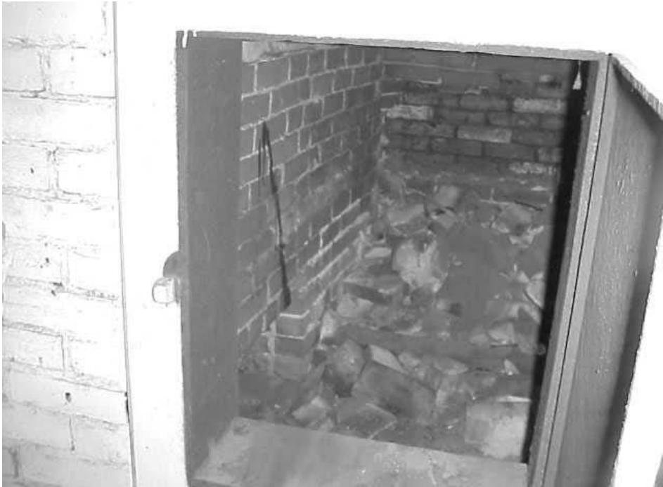
Exhaust Vent in Basement Sealed by Steel Door
