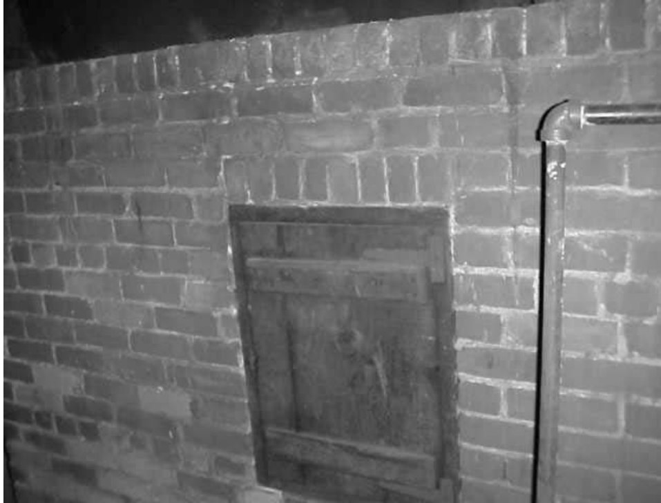
Exhaust Vent in Basement Sealed by Wooden Door in the 1848 Section
