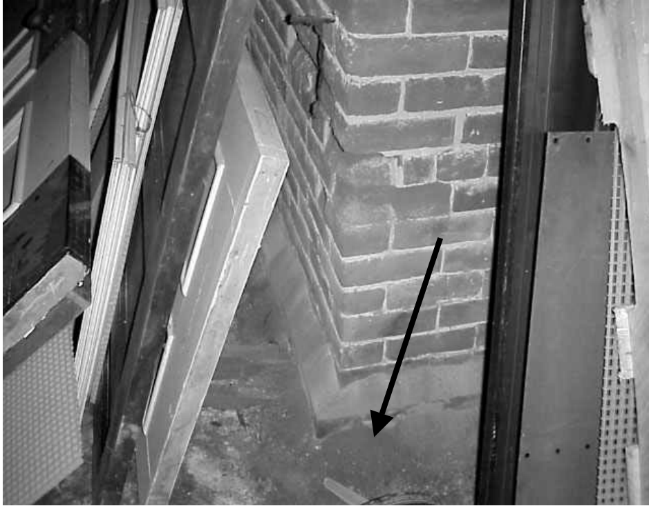
Crumbled Brick and Dust on the Outside of an Exhaust Vent Shaft
