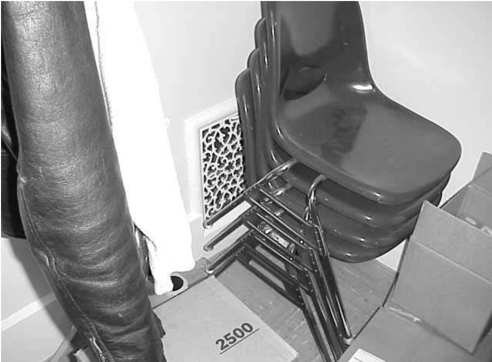
Wall Mounted Exhaust Vent
