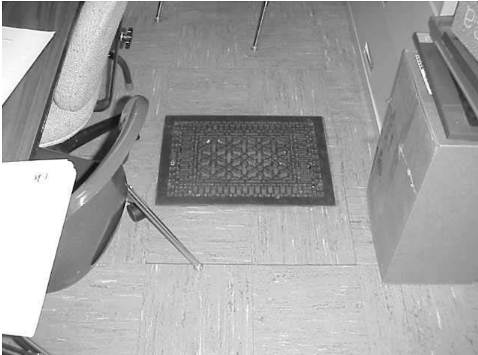
Supply Vent in Floor
