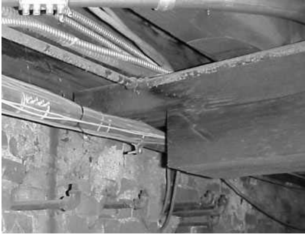
Floor Support Beam with a Cut Removing 2/3 of Wood
