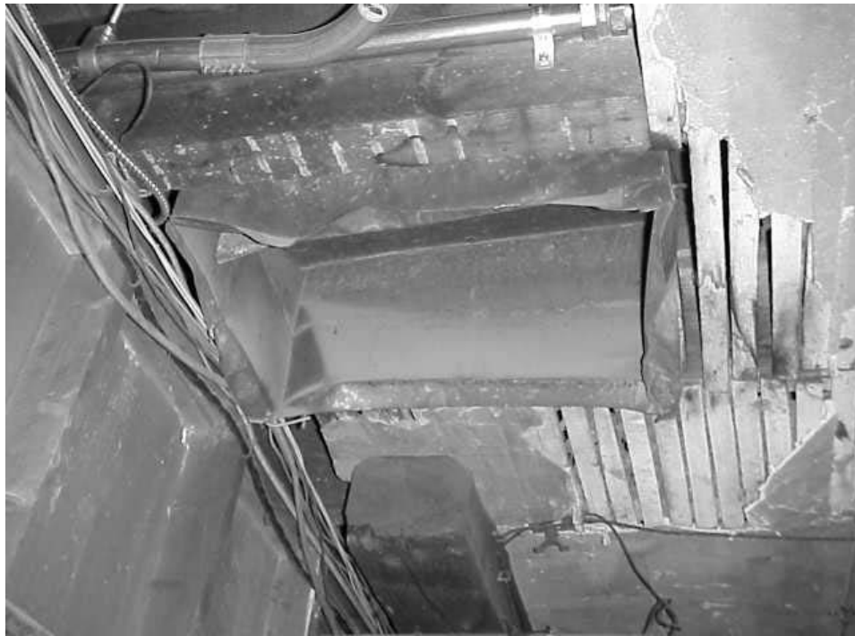
Abandoned Ductwork in Basement Ceiling below Board of Health Office, No Corresponding Vent in the first floor Was Located
