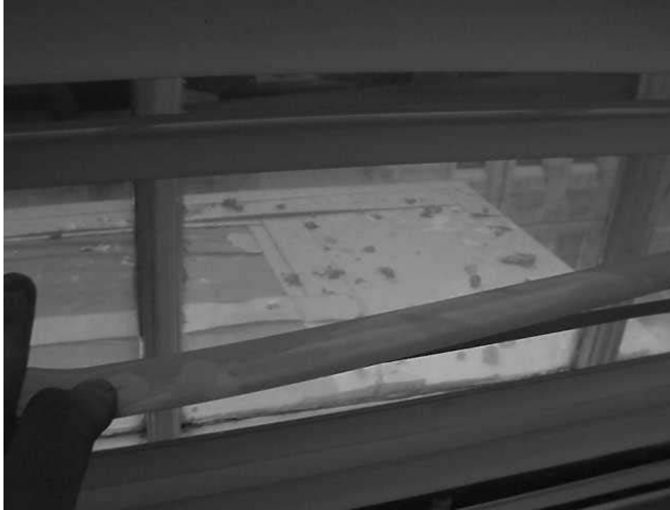
Pigeon Waste on the DPW Engineer's Office Window-Mounted Air Conditioner Casings
