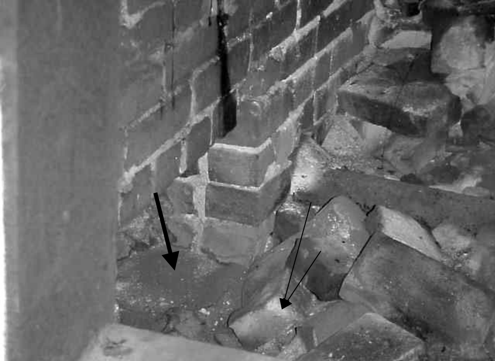
Crumbled Brick inside Exhaust Vent Shaft
