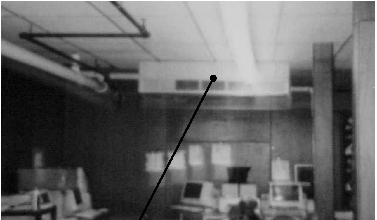
Ceiling-Mounted Univent Noted in Classroom 13
