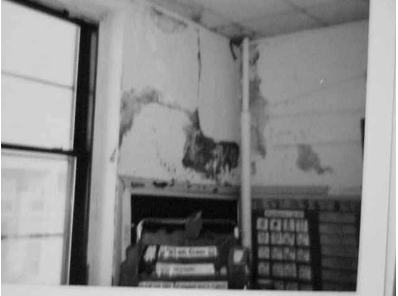
Water-Damaged Ceiling Tiles and Wall Plaster Noted in Northeast Classroom
