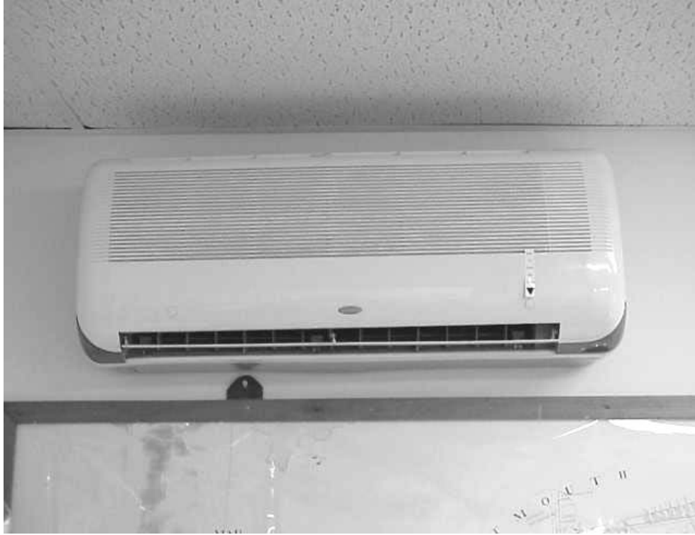
Example of Wall-Mounted Air-Conditioning (A/C) Unit Note A/C Units do not Provide Fresh Air but Recirculate Only
