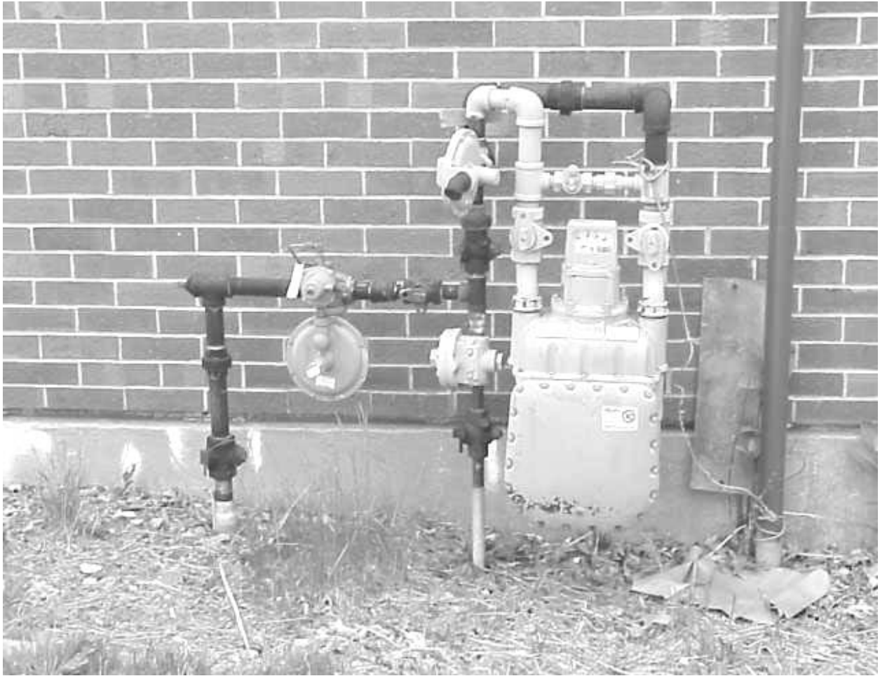
Gas Regulator Noted Leaking on Exterior Eastside Wall
