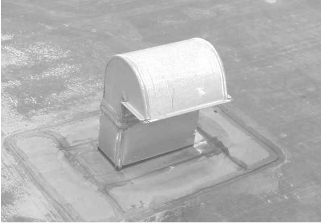
Rooftop Exhaust Ductwork for Main Office Area
