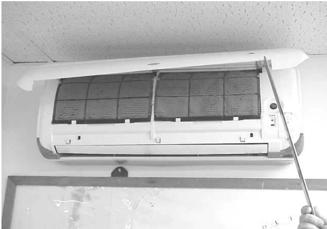
Wall-Mounted A/C Unit Opened to Expose Filter
