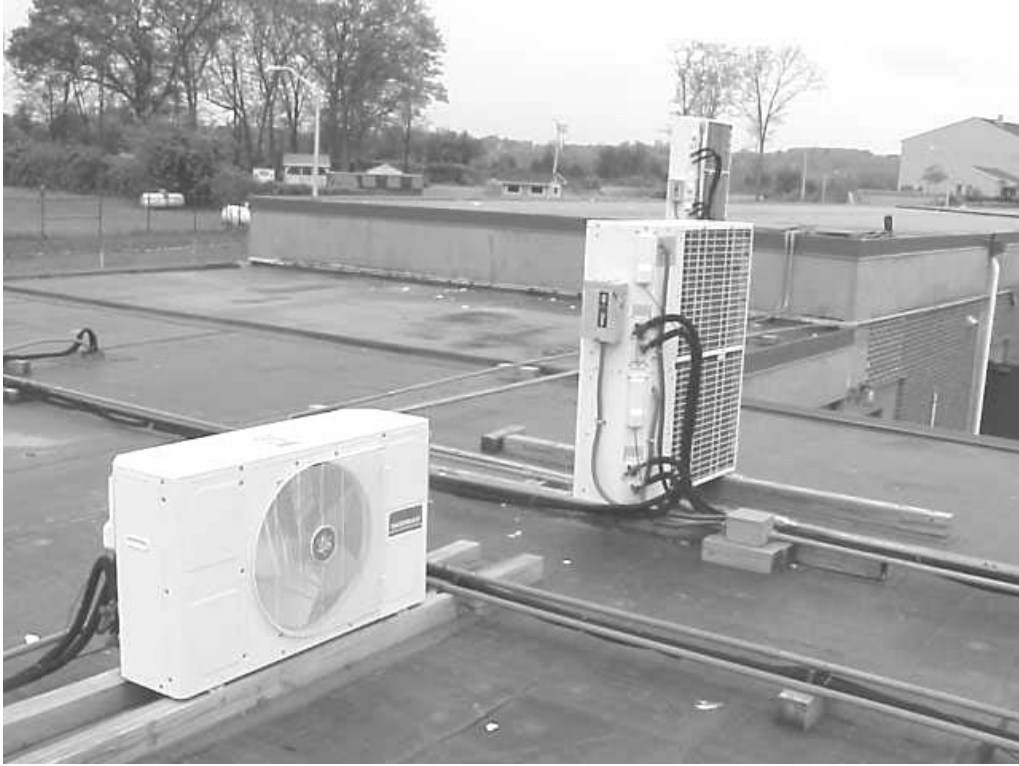
Rooftop Units Providing Chilled Water for A/C Units
