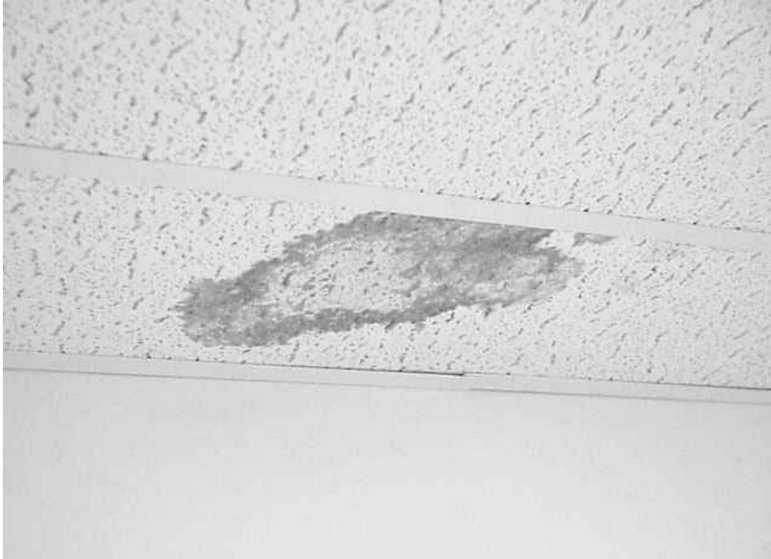
Water-Stained Ceiling Tile
