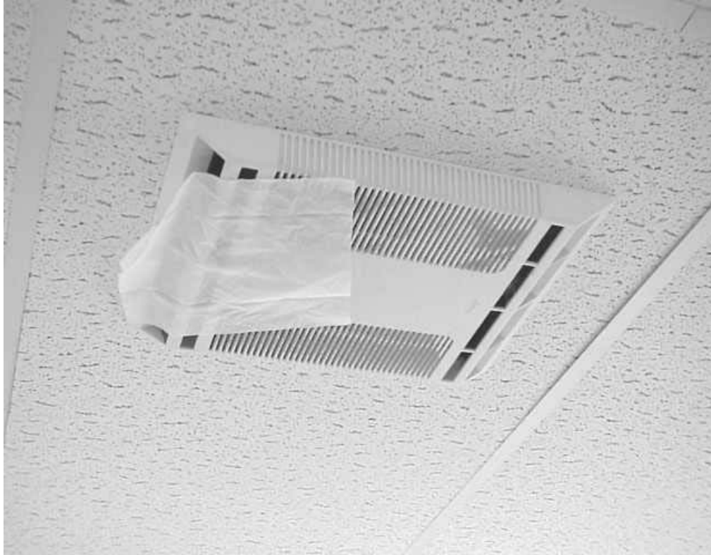
Ceiling-Mounted Exhaust Vent Noted in Billing Office Area Note Tissue Indicating Draw of Air
