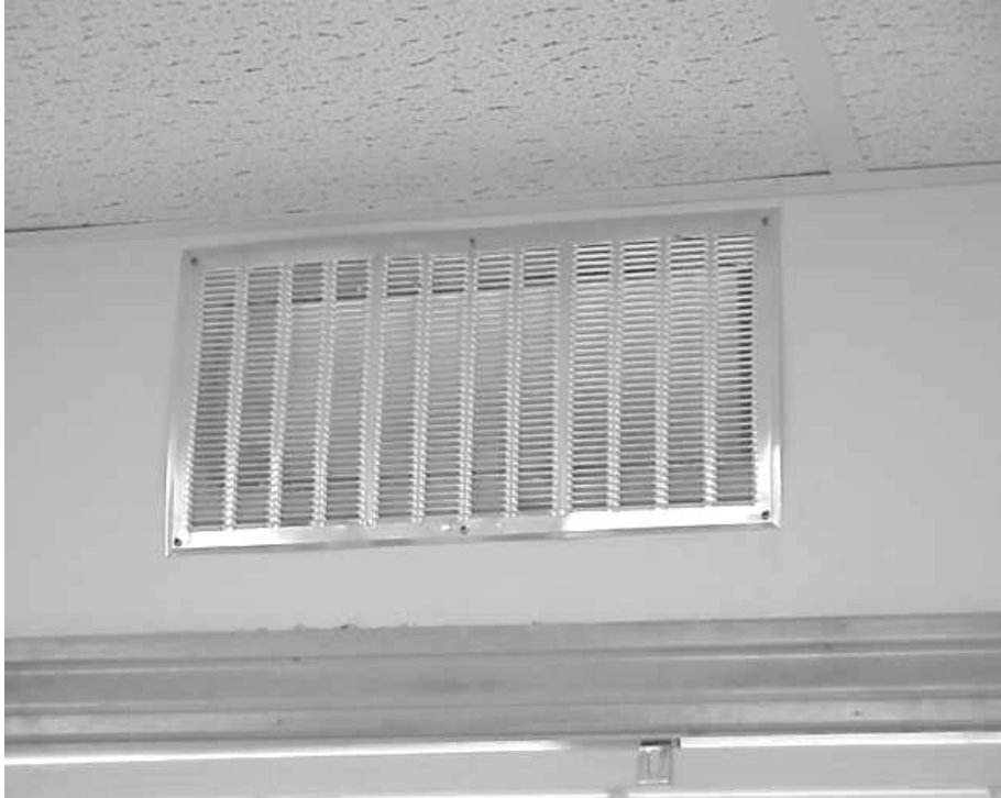
Example of Passive Wall Vent Installed in Main Office Area to Facilitate Airflow
