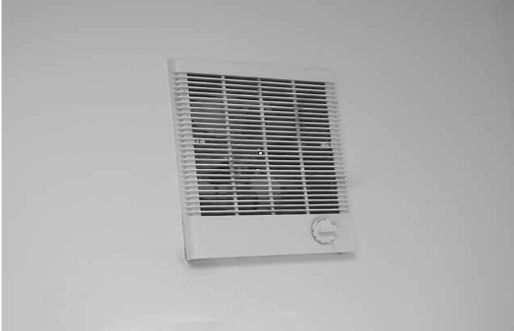
Example of Wall-Mounted Fan Installed in Main Office Area to Facilitate Airflow
