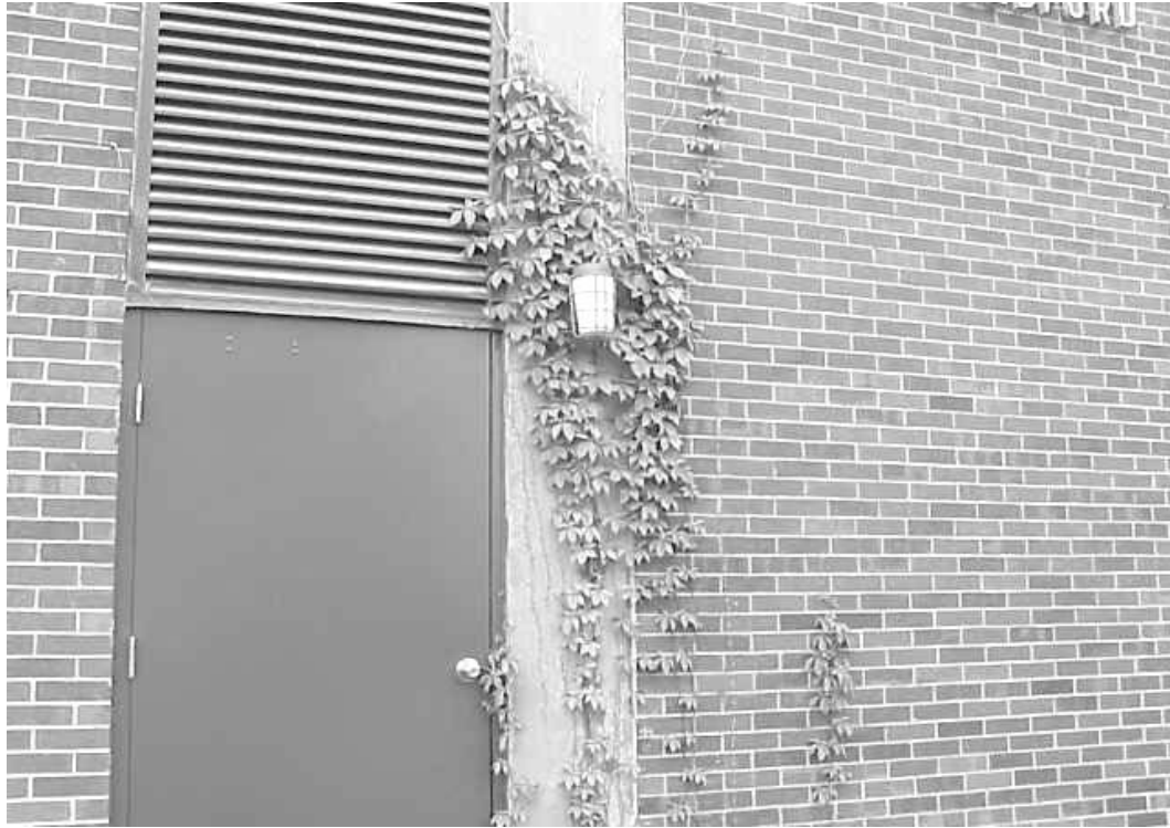
Vine Growth Noted on Exterior Brick
