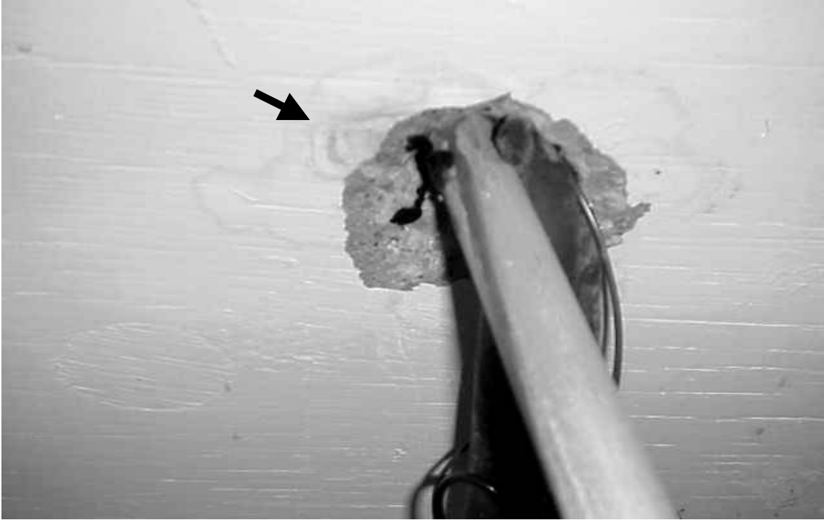
Utility Hole for Pipe Penetration through Roof Noted above Ceiling Tiles Note Water Stained Pipes and Ceiling Plaster Indicating Water Penetration
