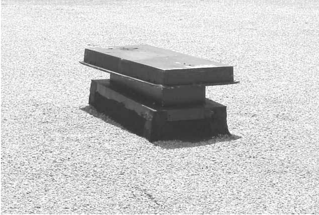
Rooftop Univent Fresh Air Intake for Interior Classrooms
