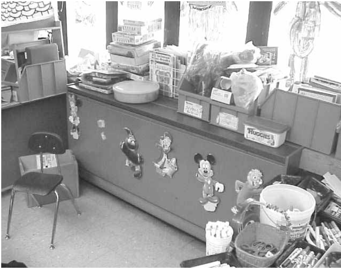
Classroom Univent: Note Materials Obstructing Air Diffuser (Top of Unit)
