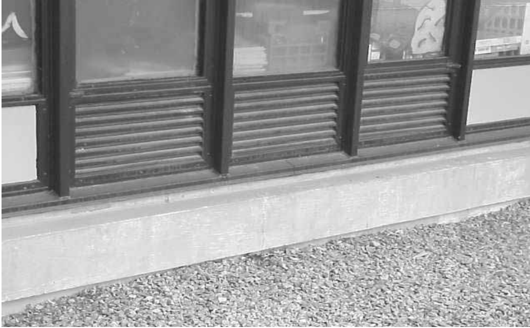
Univent Fresh Air Intakes on Exterior of Building
