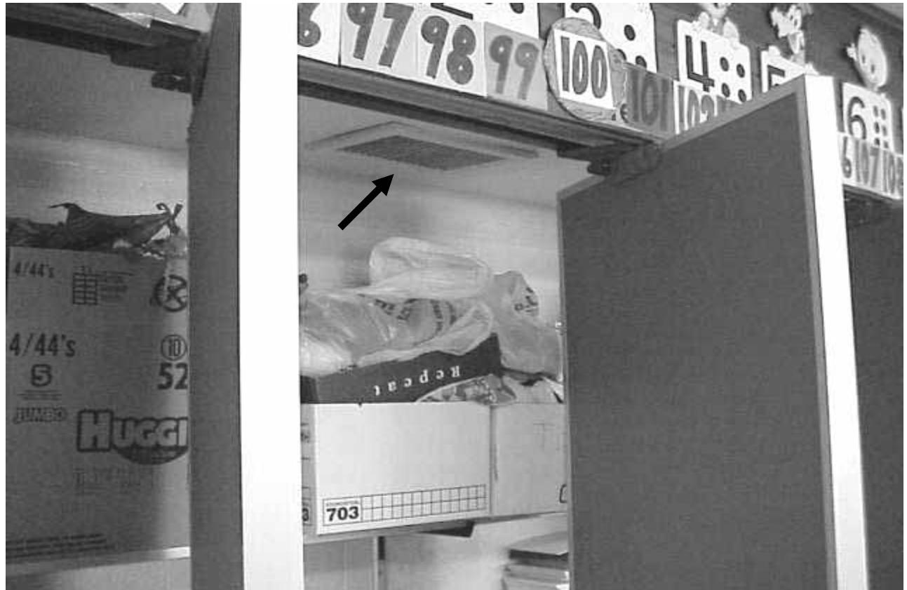
Ceiling-Mounted Exhaust Vent Noted in Classroom Coat Closets
