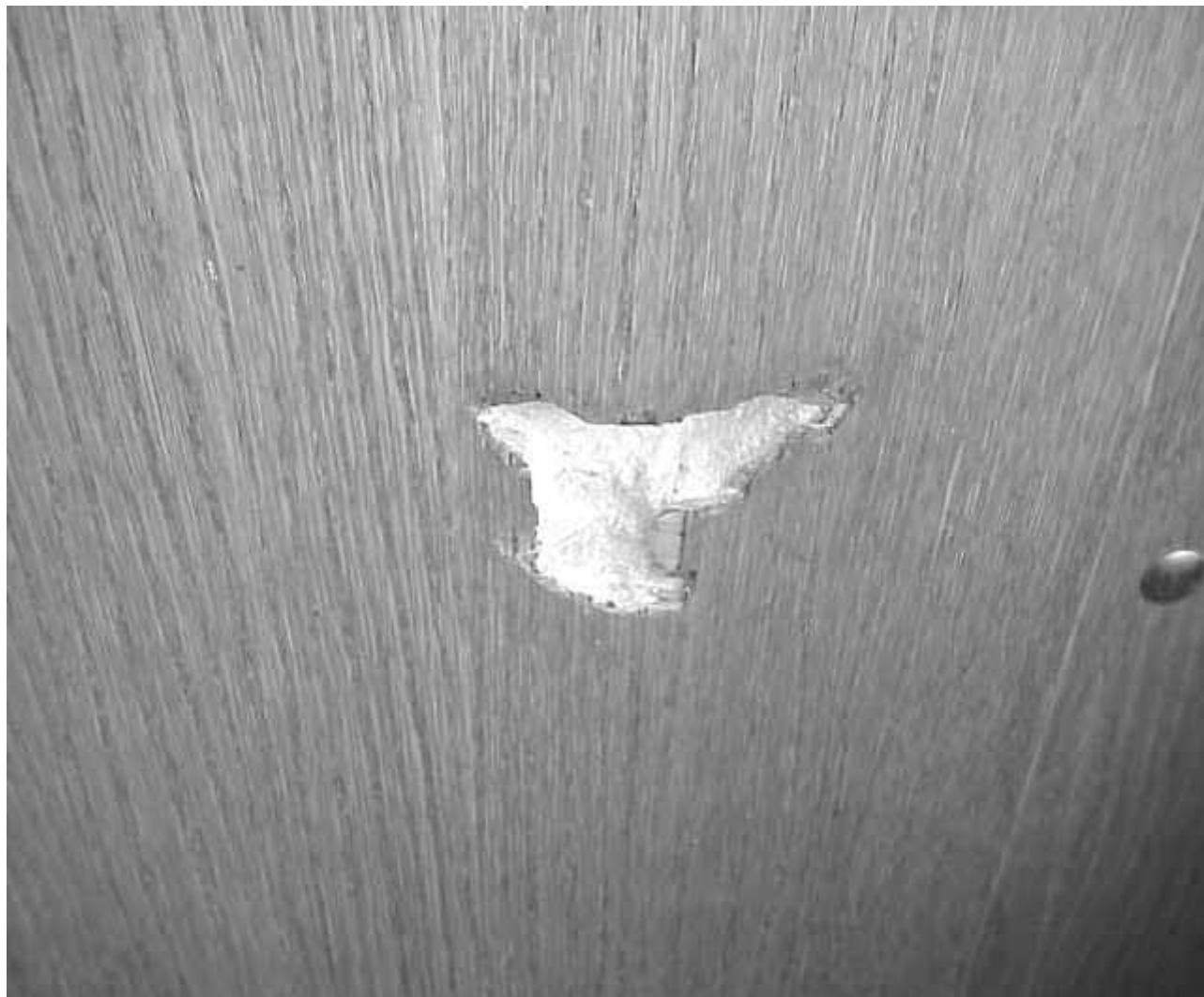
Possible Asbestos-Containing Material in Damaged Door
