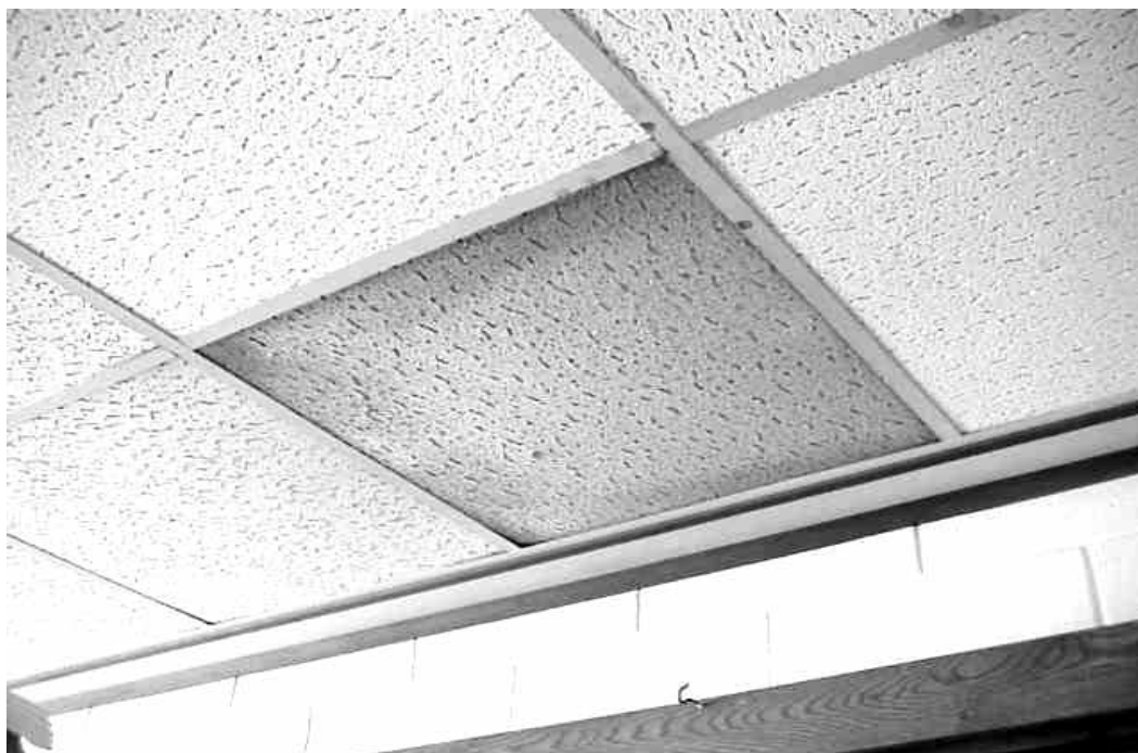
Water-Stained Ceiling Tile in Classroom
