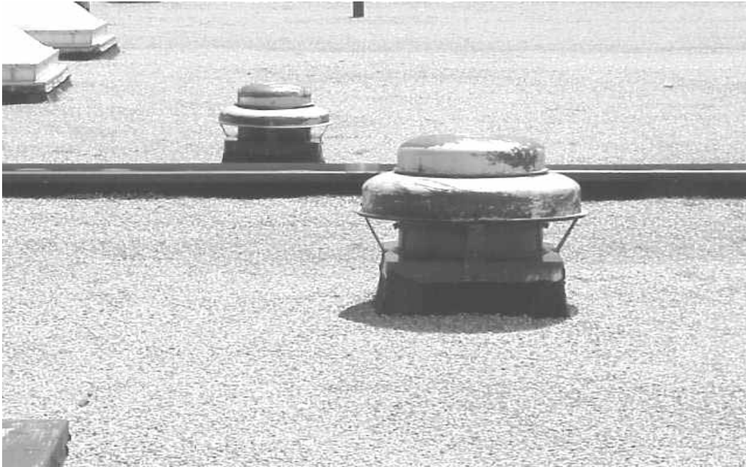
Rooftop Exhaust Motors: Note that 17 of 22 of These Motors Were Operating During the Assessment
