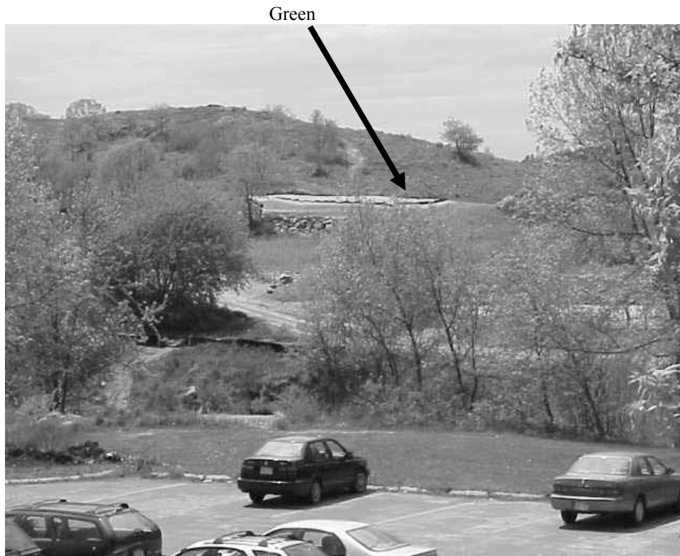
View from the Top of the Welch Elementary School Roof of Green under Construction on the Golf Course
