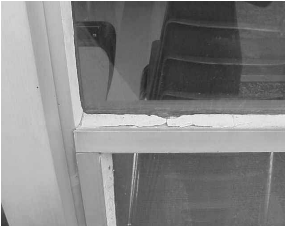
Eroded Window Caulking
