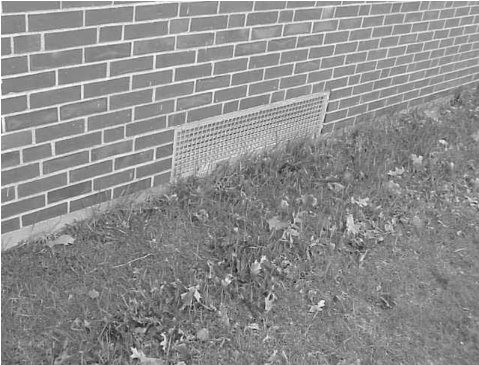
Univent Fresh Air Intake Note Lawn Growth against Air Intake
