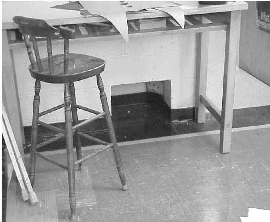
Exhaust Vent in the Original Building
