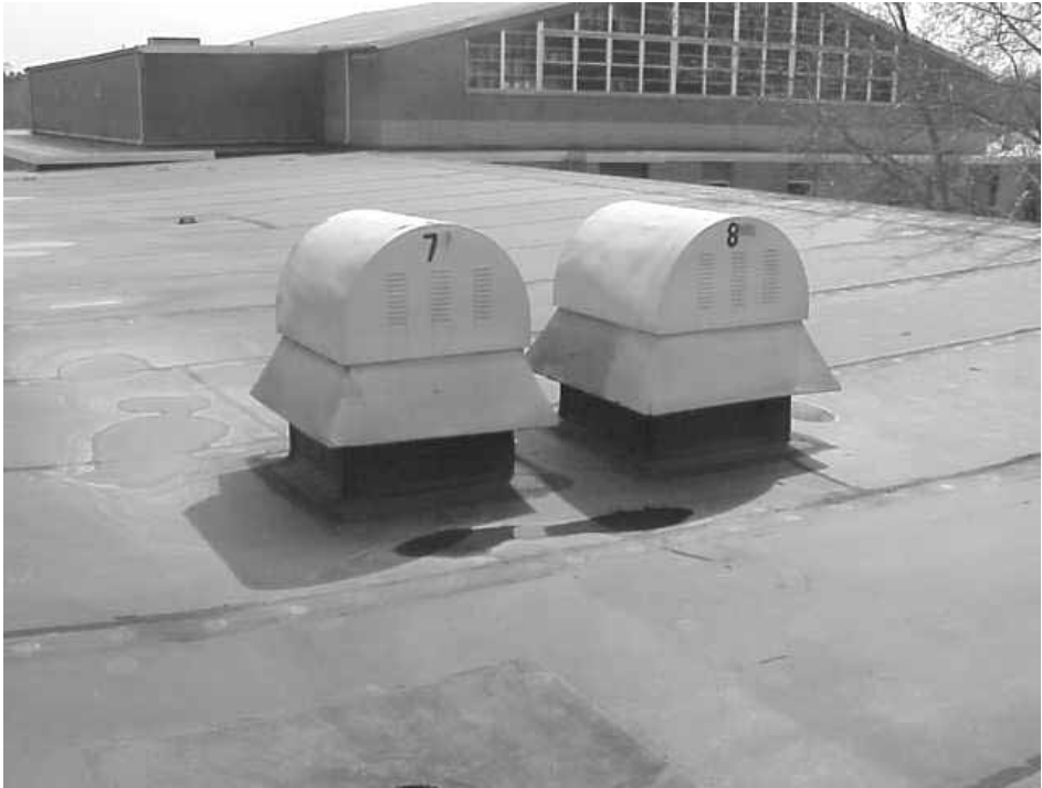
Rooftop Exhaust Vents
