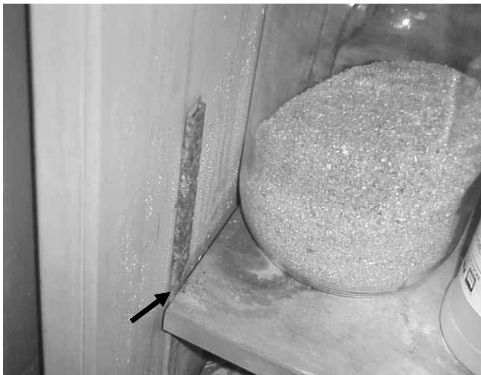
Corrosion of Shelf Support from Exposure to Stored Acids
