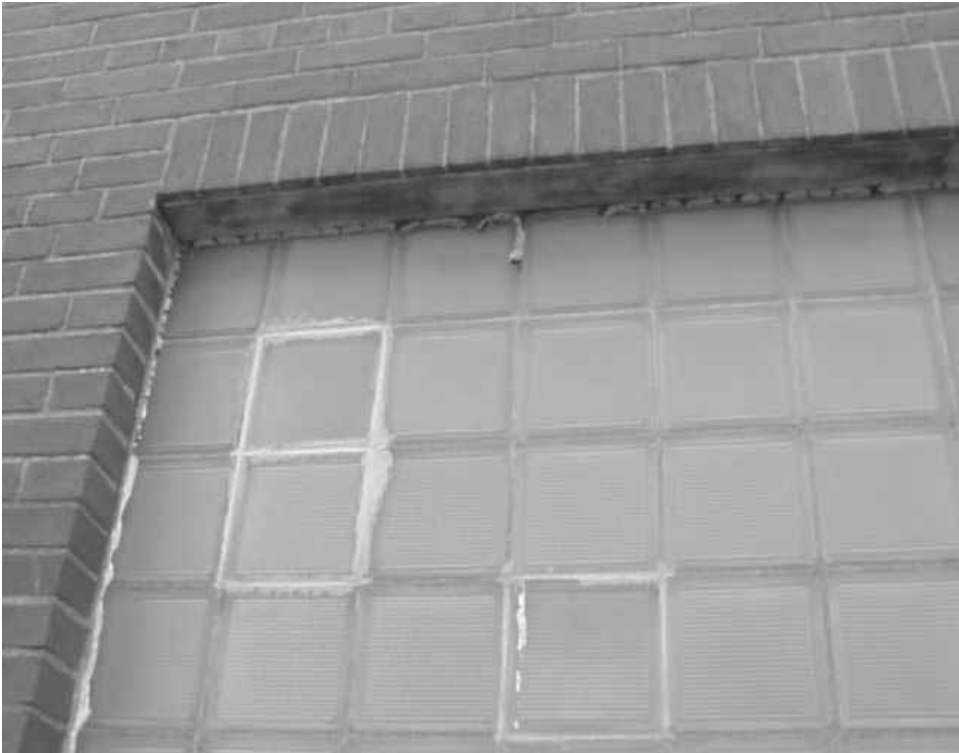
Missing and Damaged Window Caulking
