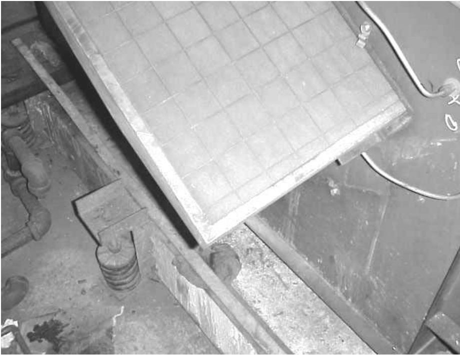
Metal Rack Filter in AHU
