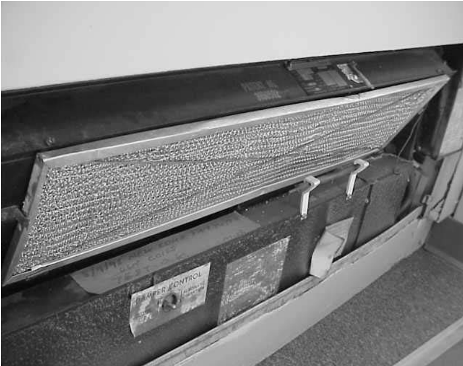
Univent with Metal Filter Installed in Univent
