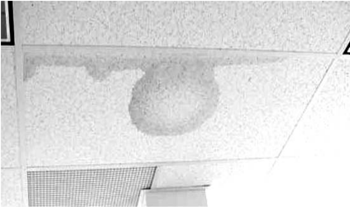
Water-Damaged Ceiling Tile
