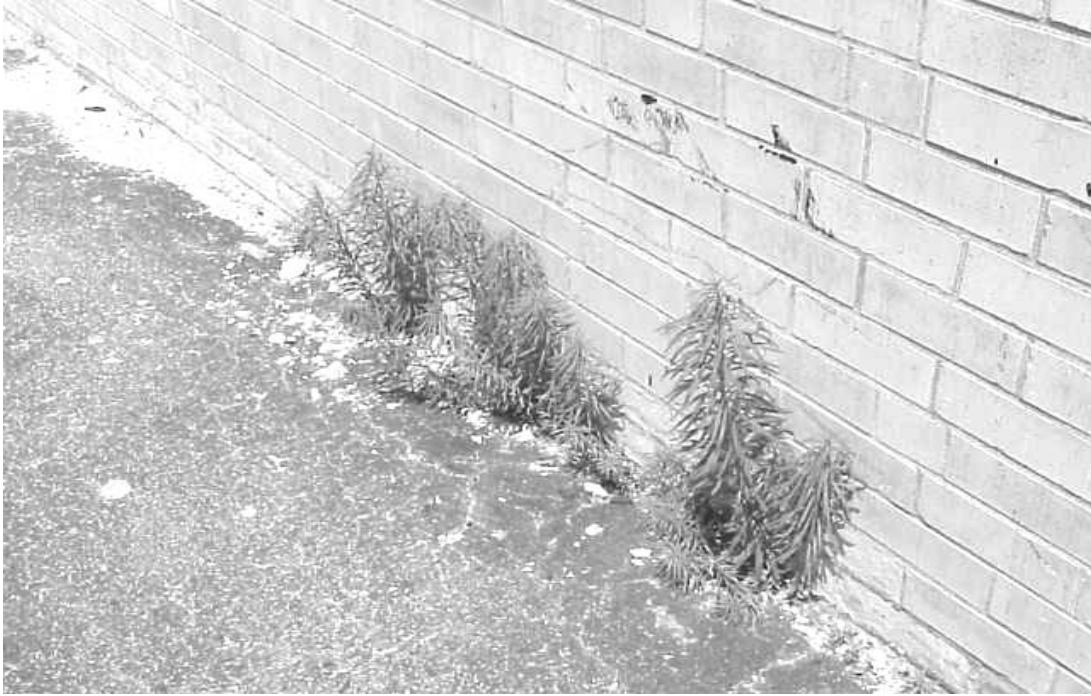
Plants Growing between the Tarmac and Exterior Brick/Foundation of Building
