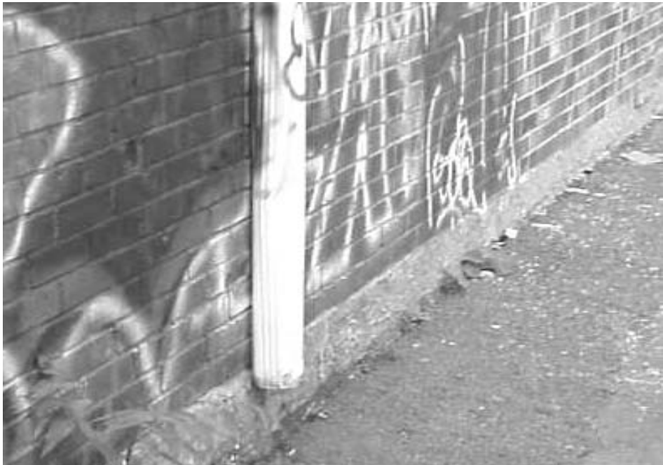
Downspout Missing Elbow Extension
