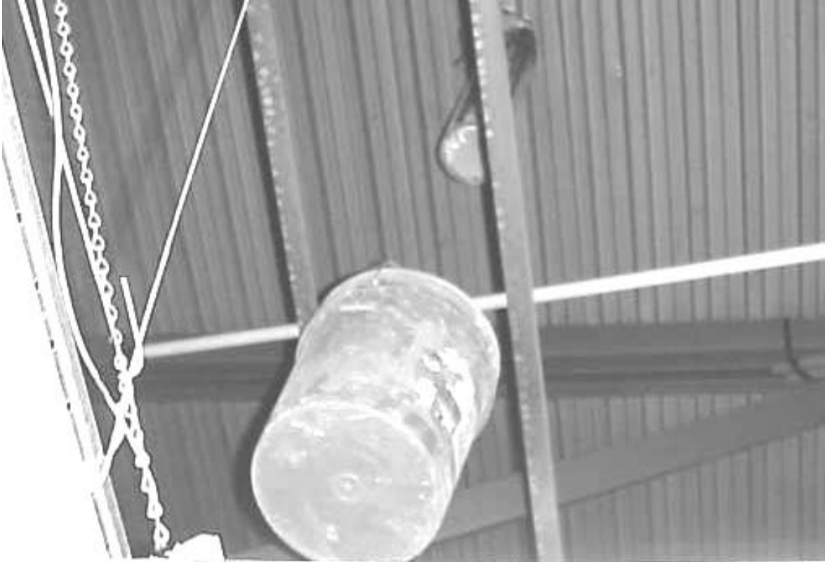
Plastic Bucket Stationed above Tiles in Ceiling Plenum
