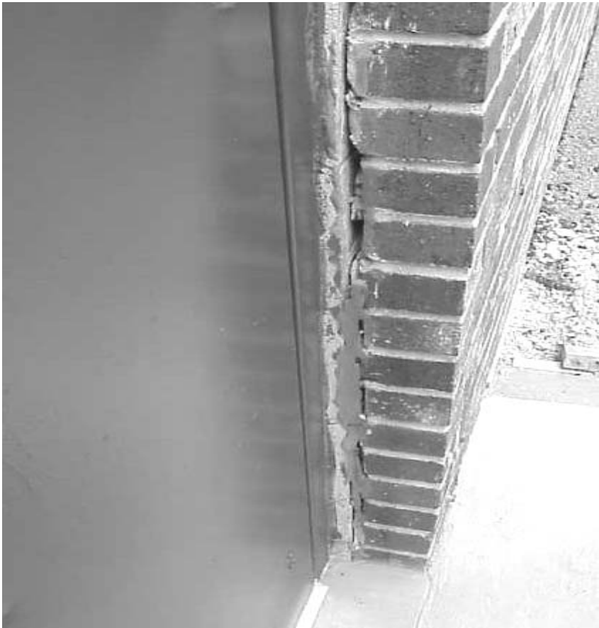
Spaces Noted between the Interior and Exterior Brick of Building
