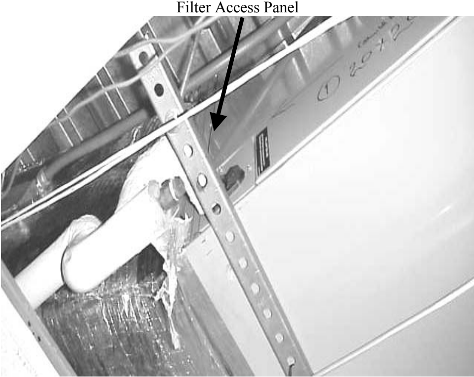
Filter Access Panel behind AHU Pipes
