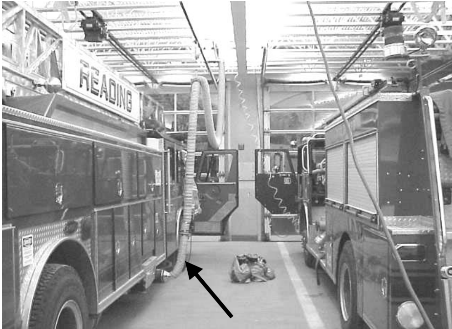
Tail Pipe Exhaust Vent System
