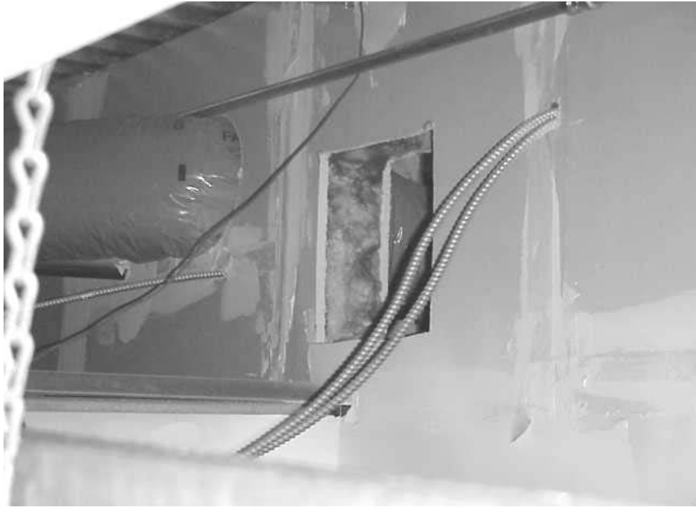
Holes Cut Into the Gypsum Wallboard to Create Pathway from Bunkroom Ceiling Plenum into The Hallway Ceiling Plenum, Note Exposed Fiberglass Insulation
