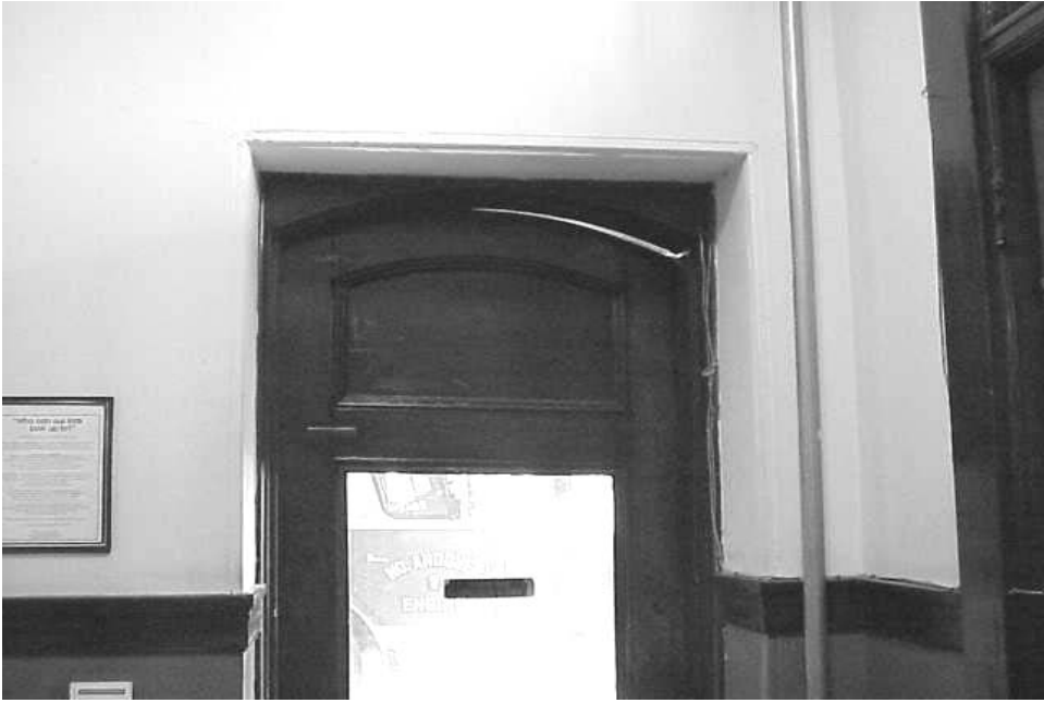
Space in Doorframe Adjacent to Engine Bays
