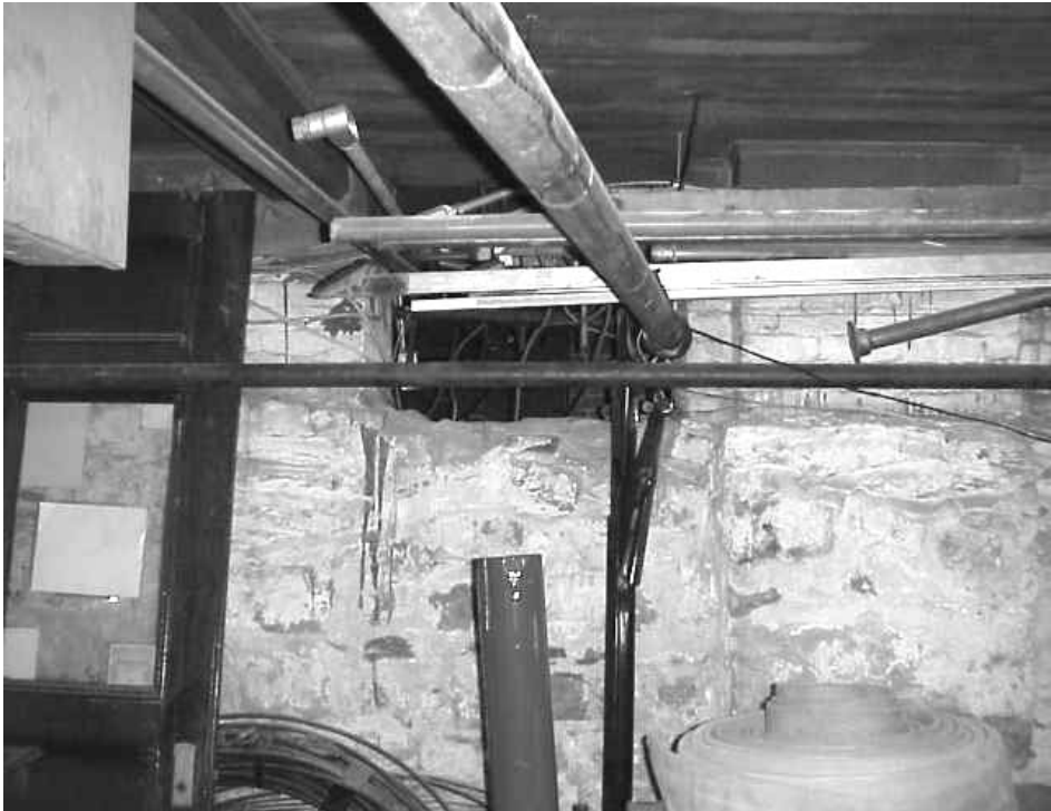
Hole in Fire Station/Town Hall Shared Wall
