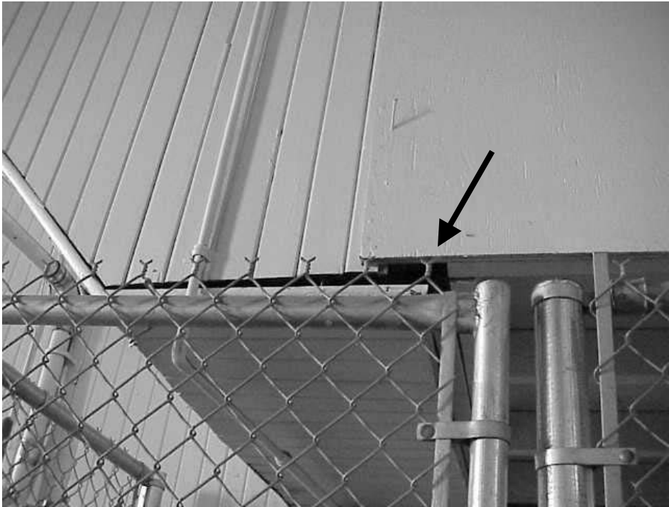
Spaces in Wall around Back Stairwell Wall
