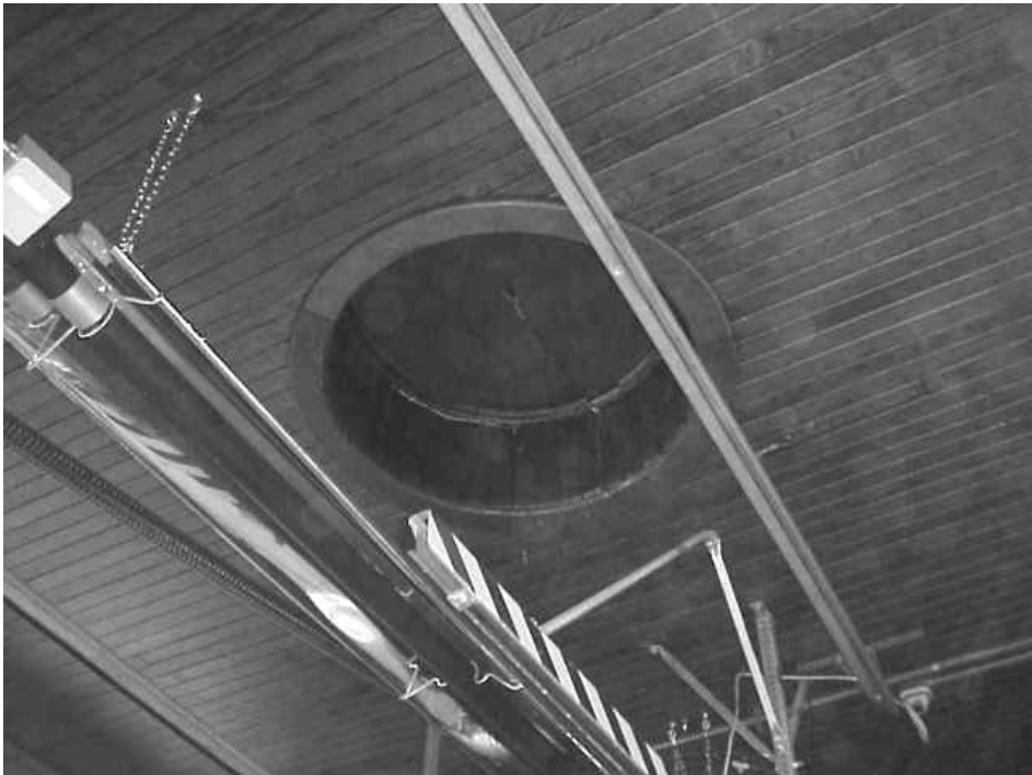
Fire Pole Hole in Ceiling
