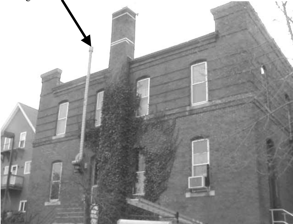
Exhaust Vent for Fire Engines
