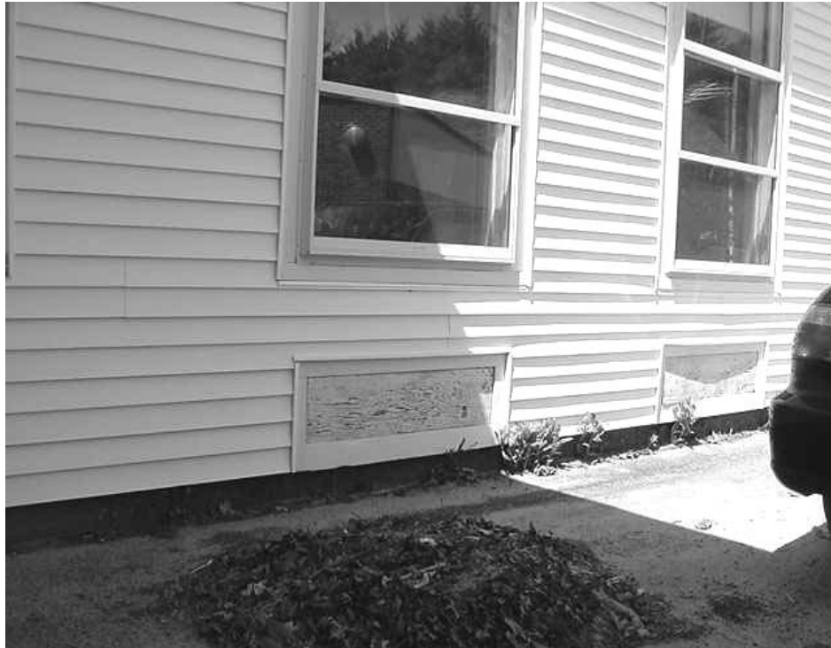
Sealed Univent Fresh Air Intakes for Library and Room 106
