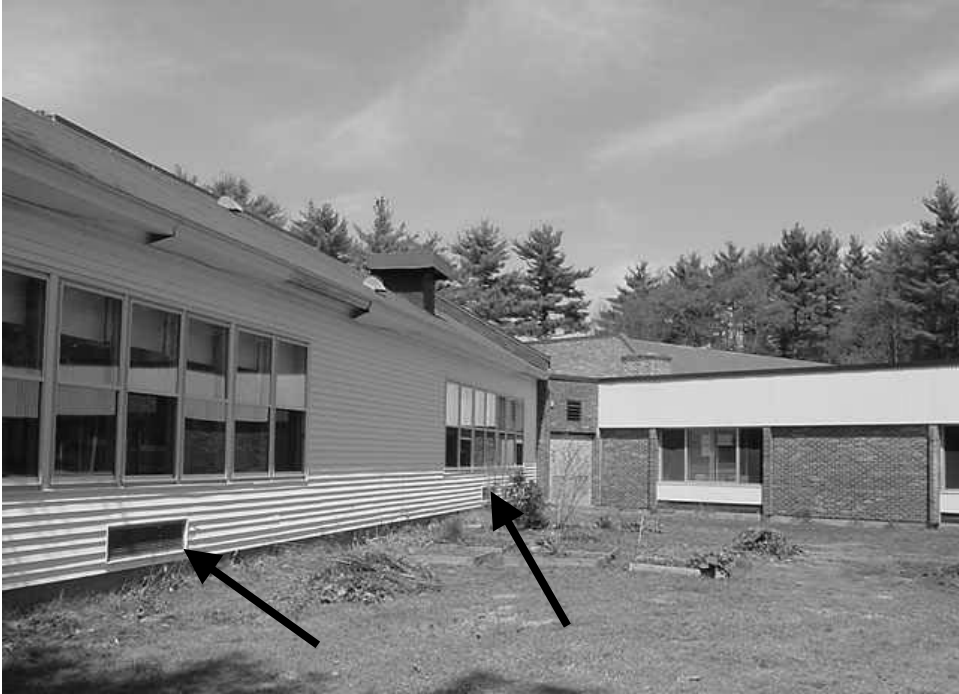
1960s Wing Univent Fresh Air Intake
