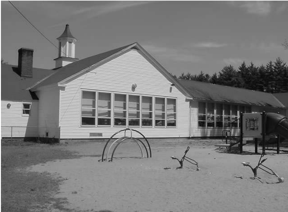
Edge Of Roof Missing Gutters
