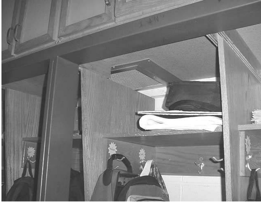
Exhaust Vent Grilles Located in Ceiling of Closet in 1975 Wing
