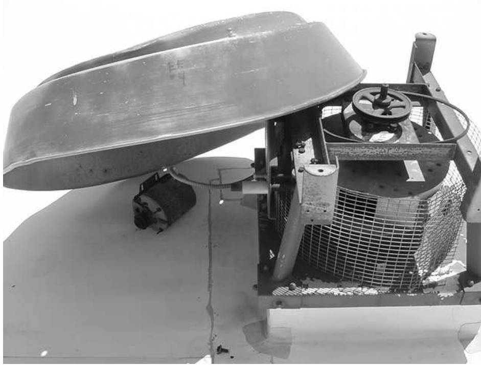
Disassembled Exhaust Vent Motor On 1975 Wing Roof
