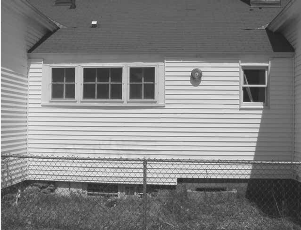
Edge Of Roof Missing Gutters over Crawlspace Vents
