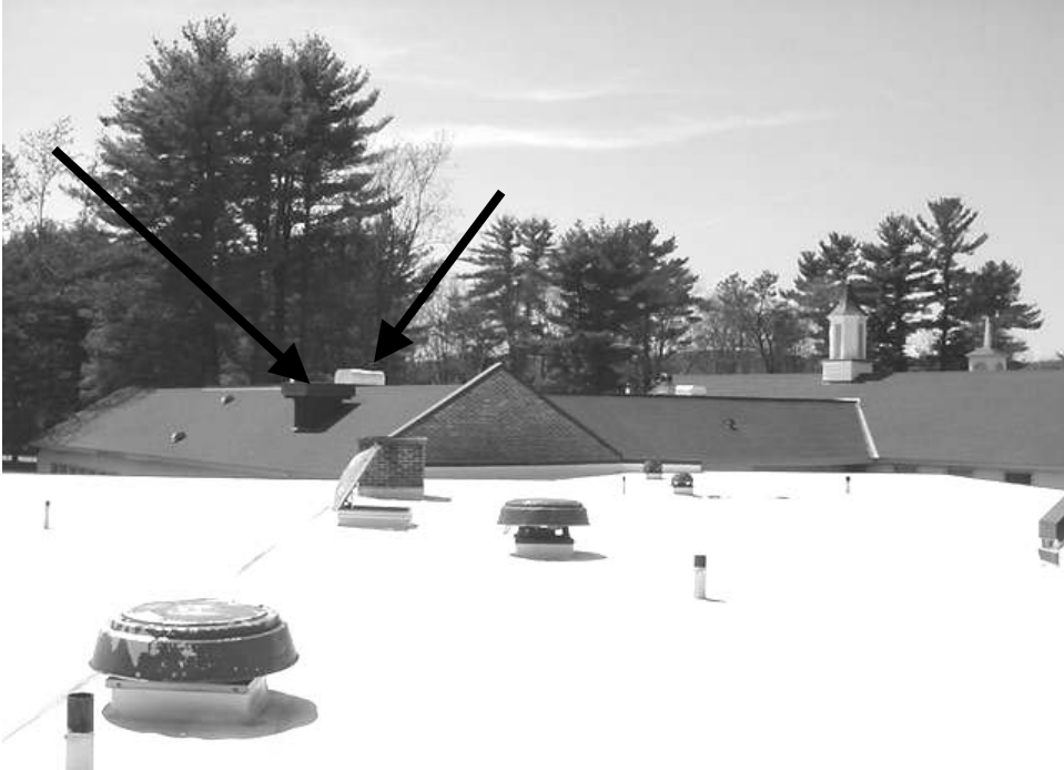
1960's Wing Rooftop Exhaust Vent Termini
