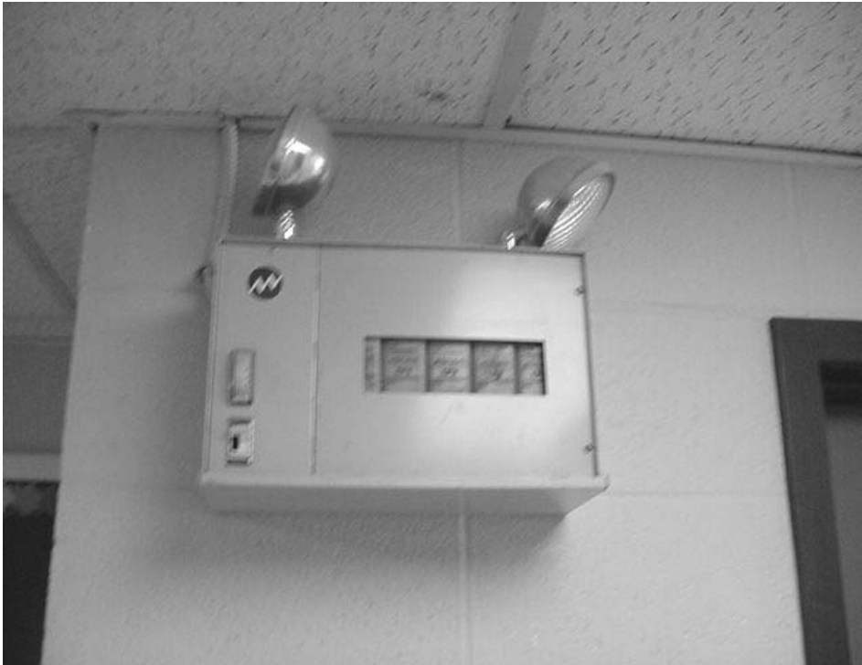
Emergency Light Powered By Acid Battery
