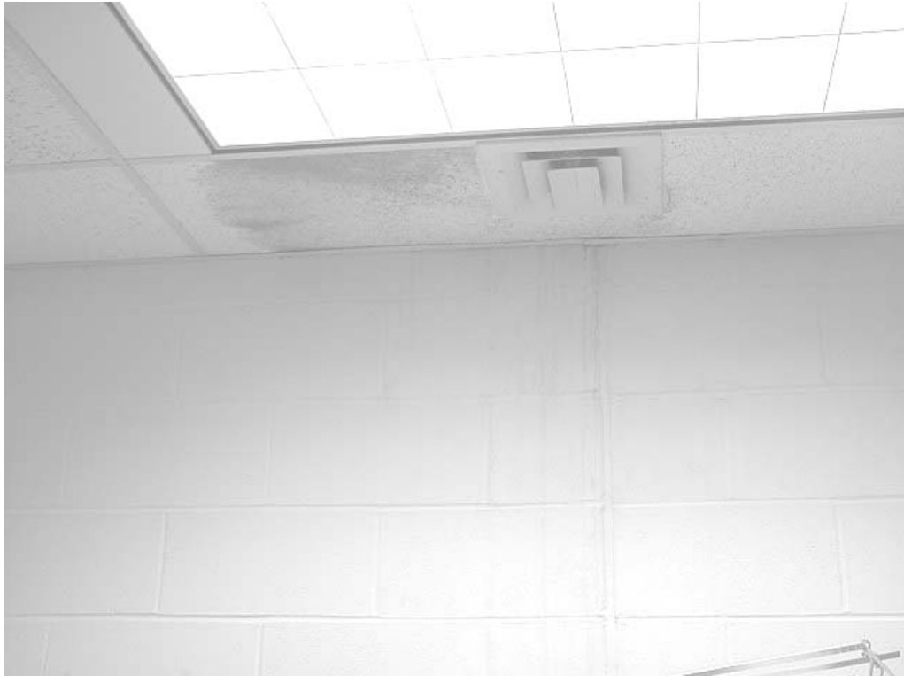
Water Damage Ceiling Tiles in area 128-I Dean's Office File Room, Note Water Stains on Wall
