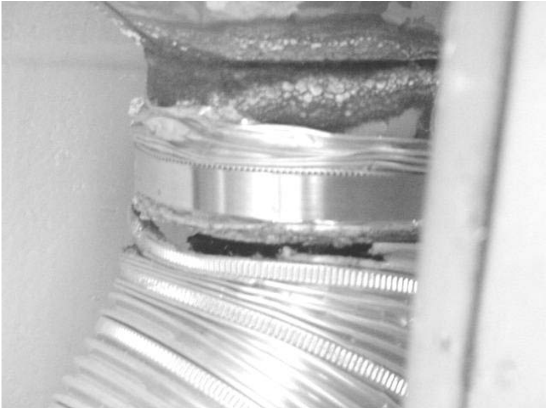
Damaged Ductwork to Kiln
