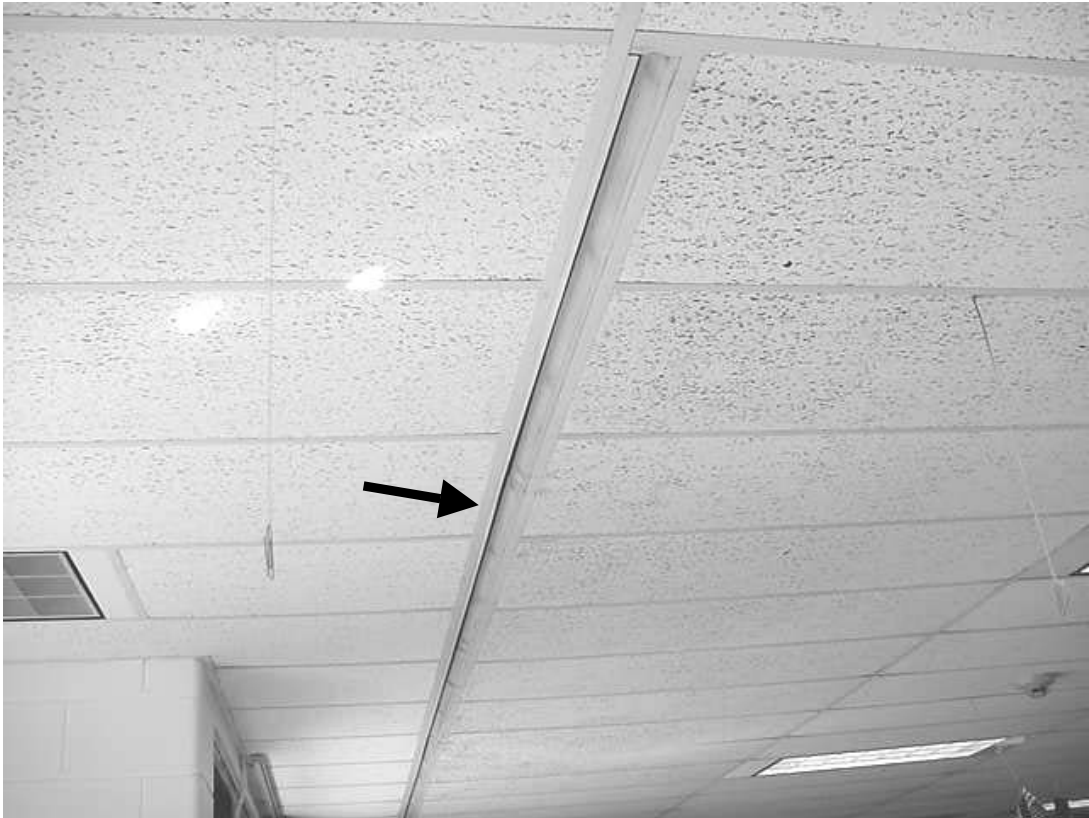
Slotted Air Diffuser in Classroom
