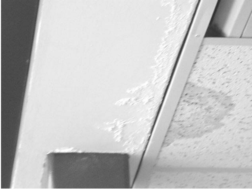
Efflorescence (e.g., mineral deposits) and Stained Ceiling Tile in Library
