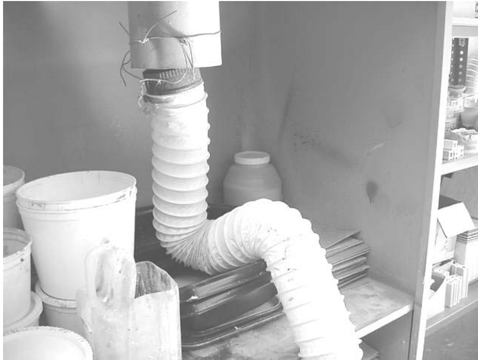
“Pinched” Flexible Ductwork Venting Kiln out of Laboratory Vent Hood
