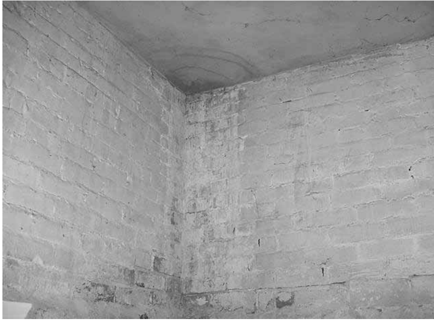
Damaged Brickwork in Storeroom at Southeastern Corner of Building
