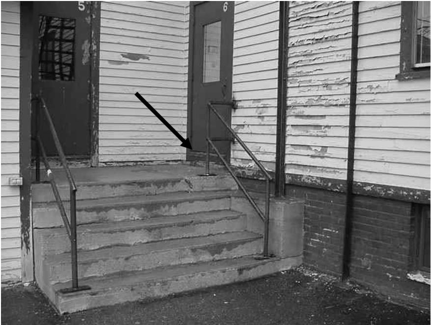
Water Damaged Wood Threshold
