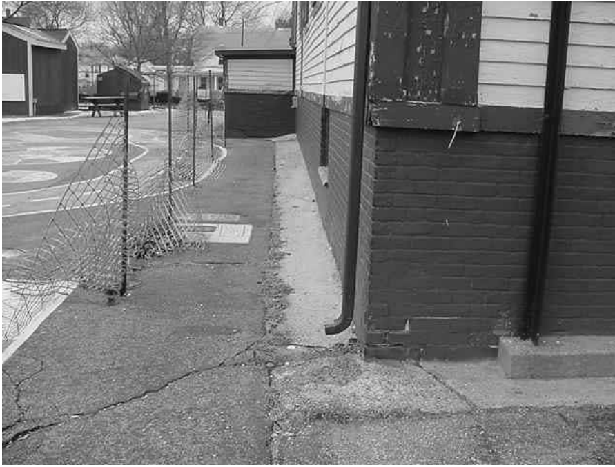
Downspout on the Southeastern Corner of Building, Note Cracks in Concrete and Tarmac
