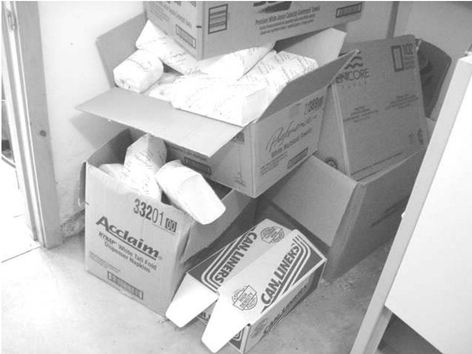
Porous Materials Stored in Mechanical Room
