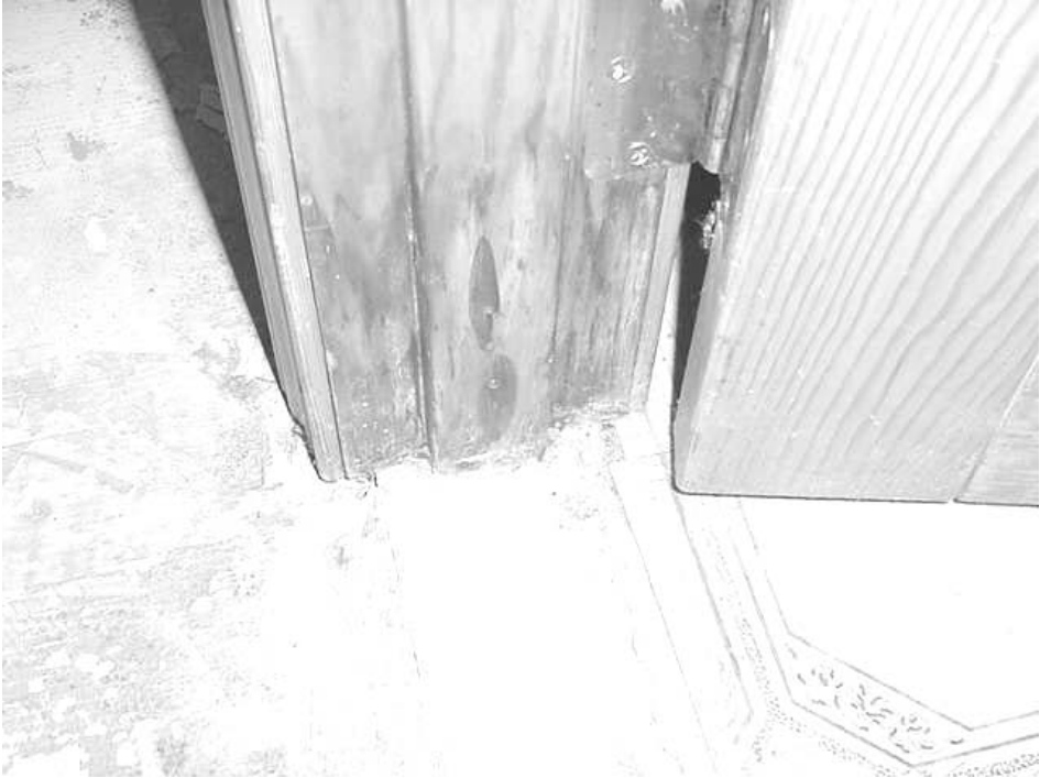
Water Damaged Wood Trim
