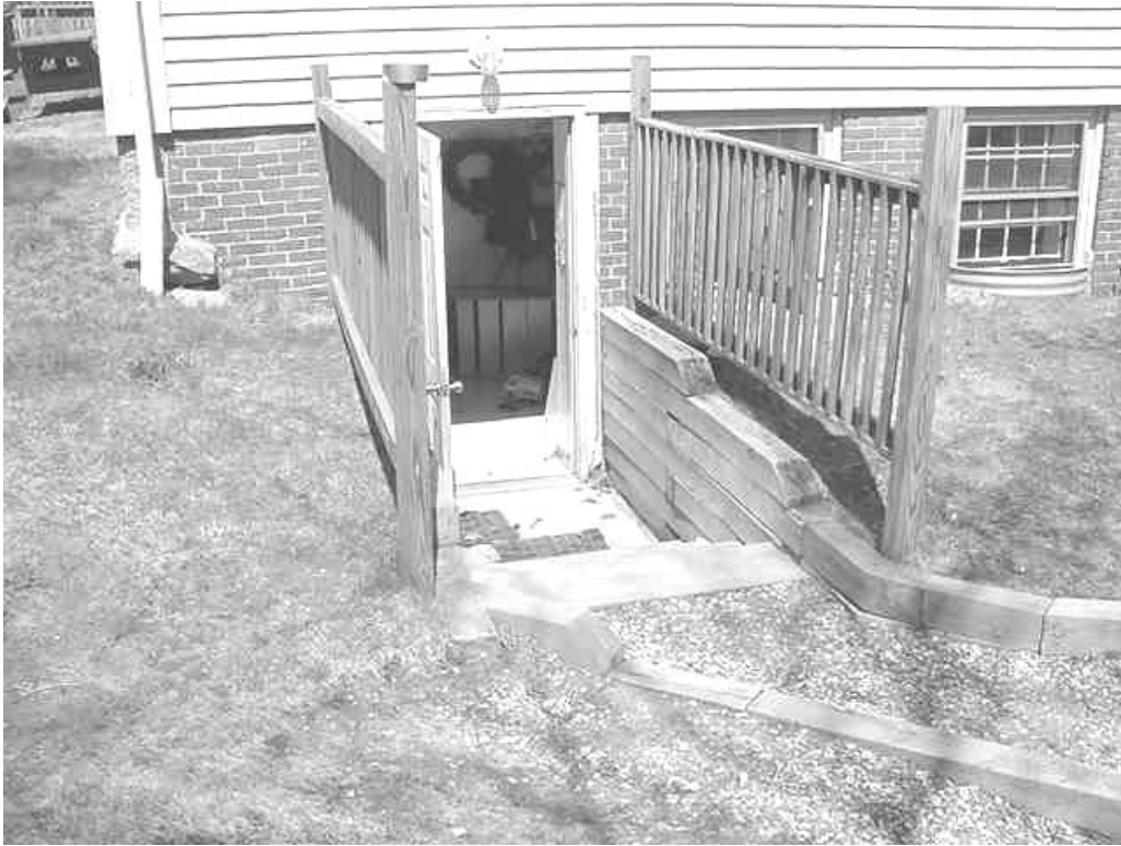
Entrance to Basement Head Start, Where Flooding Occurred
