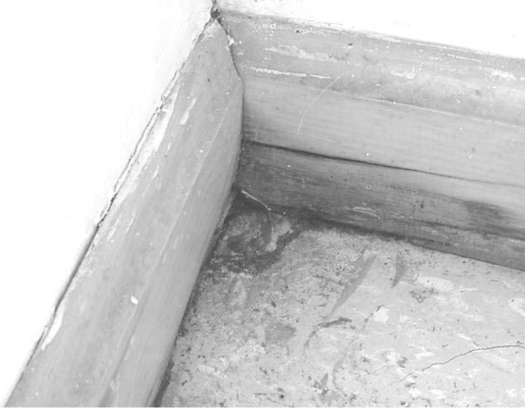
Water Damaged Wood Trim
