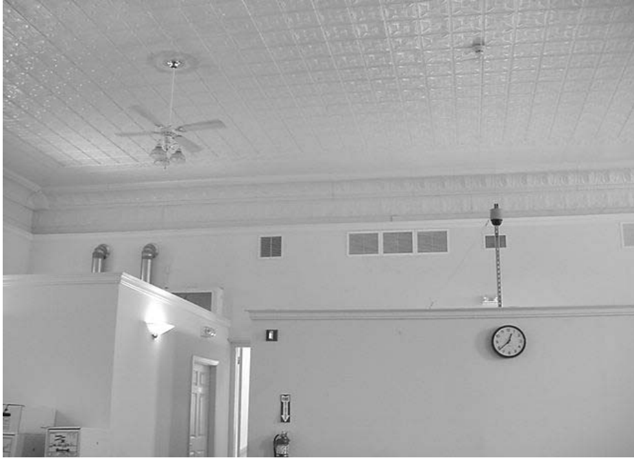
Second Floor Fresh Air Supply Vents
