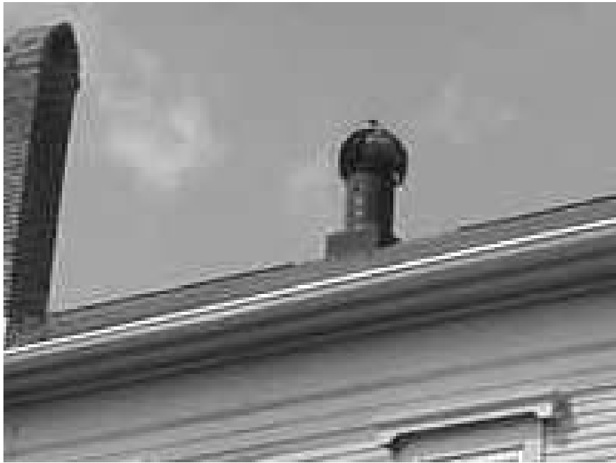
Turbine Exhaust Vent On Roof
