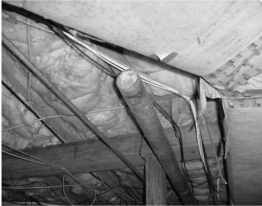
Another Open Pipe in the Basement
