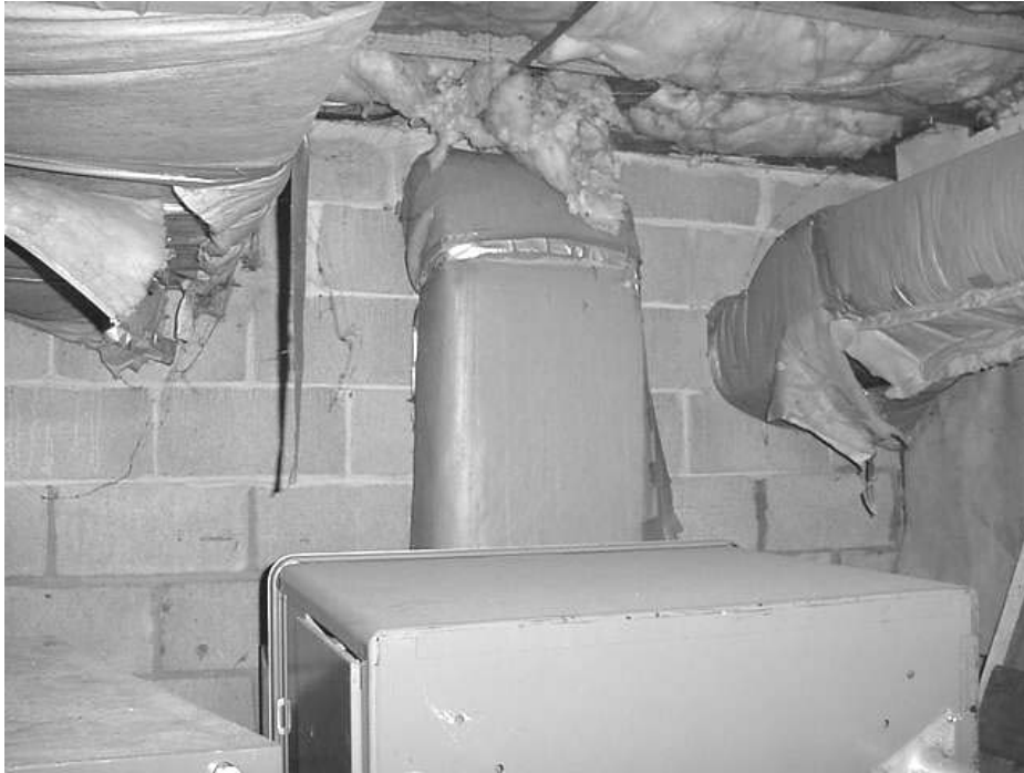
Air Intake for Basement AHU Located behind File Cabinet in Basement
