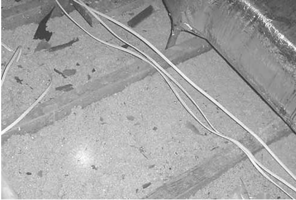
Bird Waste on Insulation in Attic
