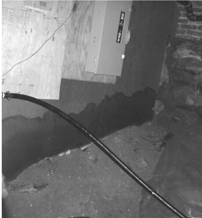
Wall Material Enclosing Fiberglass Insulation on Foundation, Note Size of Water Stain
