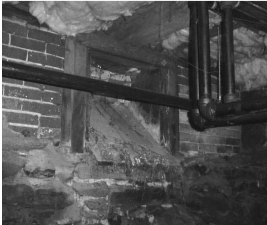
Interior View of Former Coal Chute, Note Heavy Water Damage
