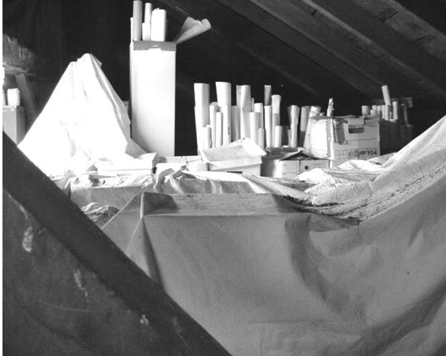
Bird Waste on Sheets in Attic
