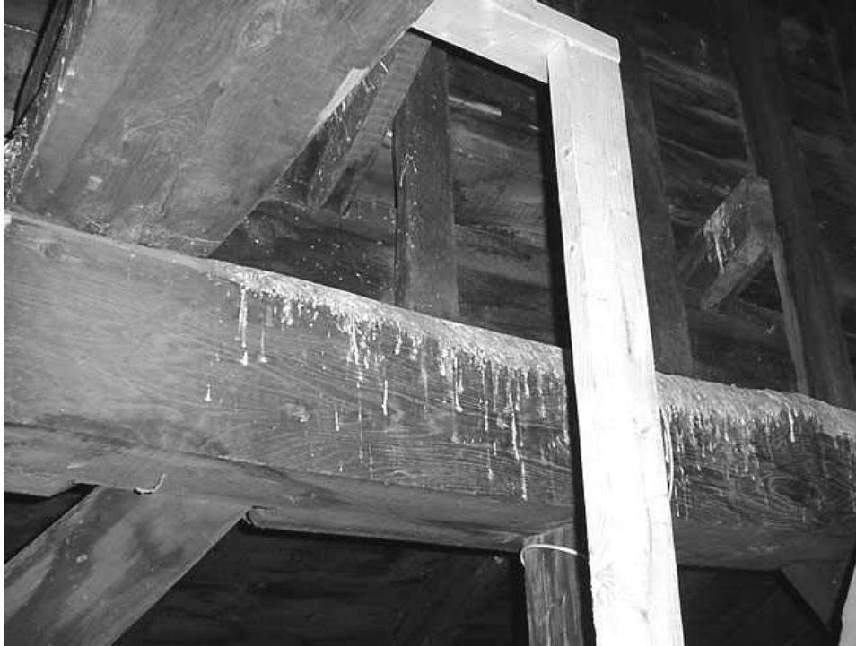
Bird Waste on Beams in Attic
