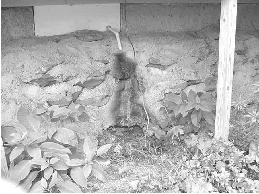
Condensation Drain That Empties onto Foundation
