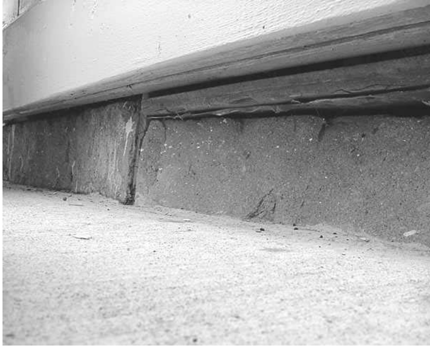
Opening In Foundation along Sidewalk
