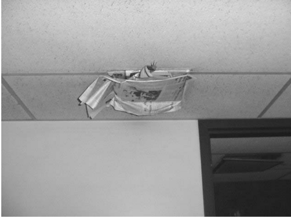
Fresh Air Diffusers in Bunkhouse Sealed with Cardboard or Newspaper
