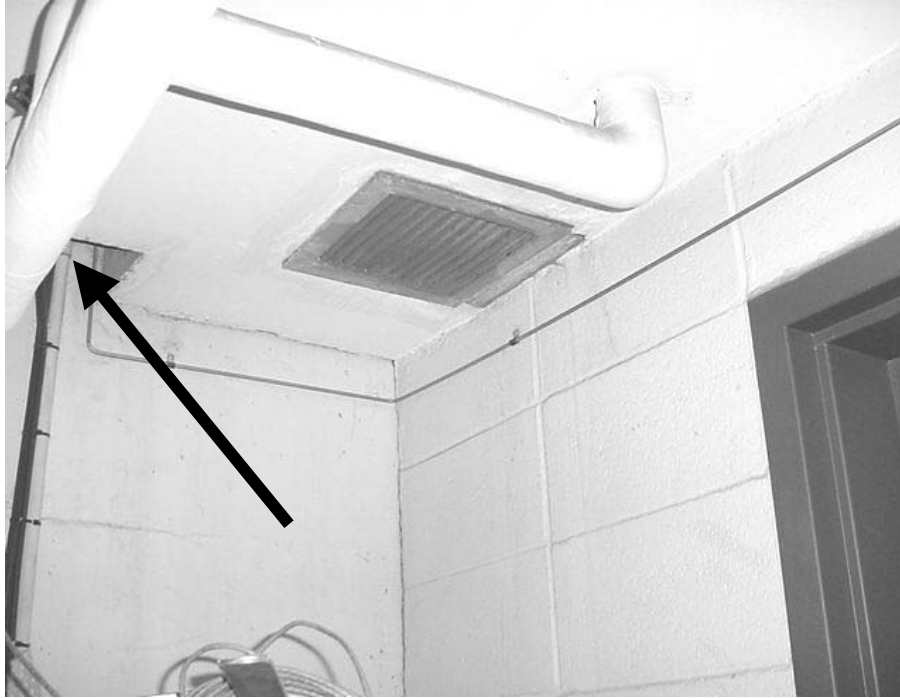
Hole in the Ceiling of the Former Oxygen Cylinder Filling Room on Garage Level
