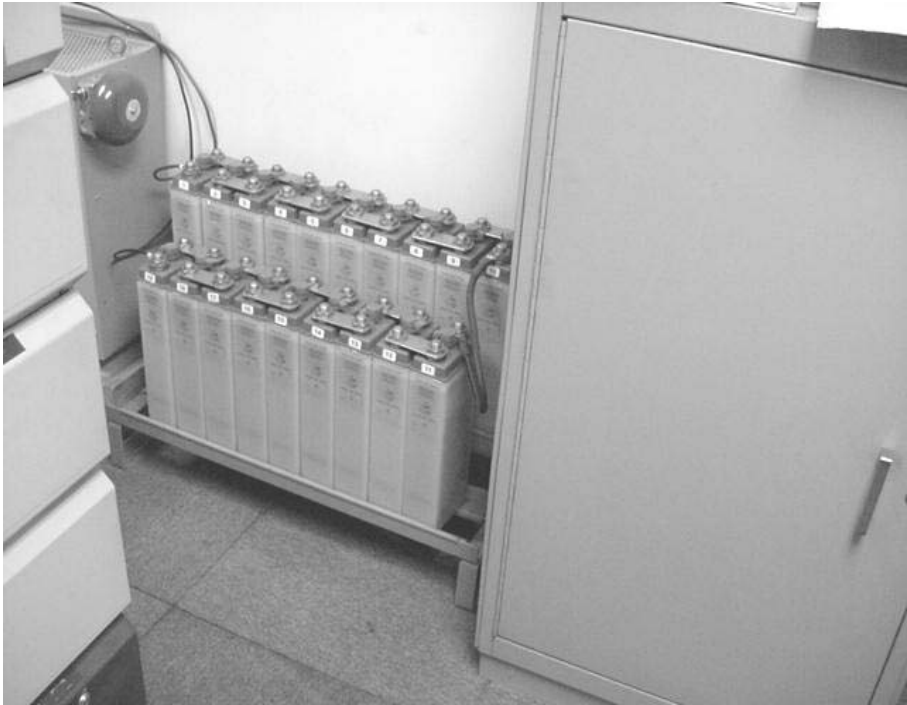
Acid Batteries in Alarm Storeroom
