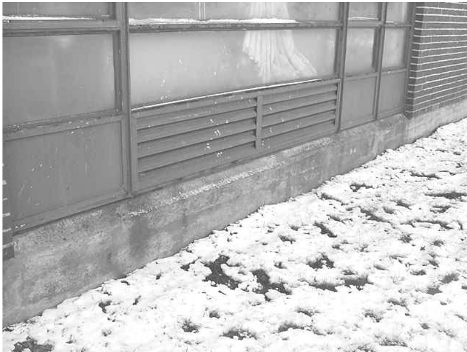
Univent Air Intake
