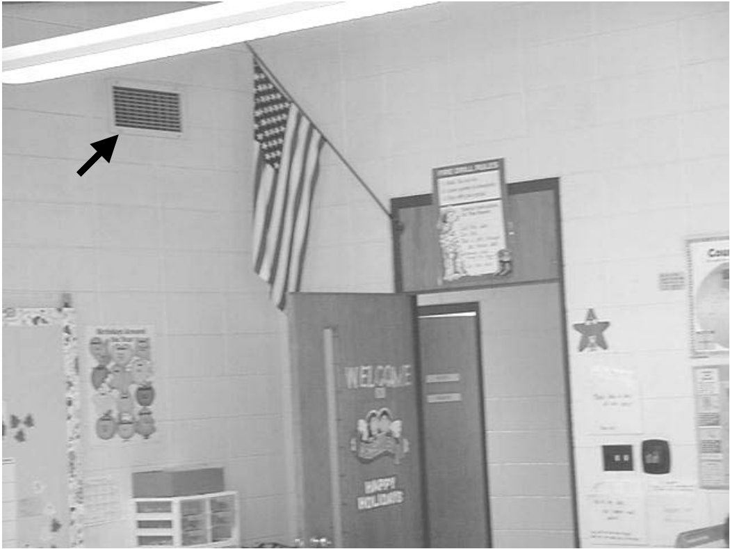
Classroom Exhaust Vent Note Open Door
