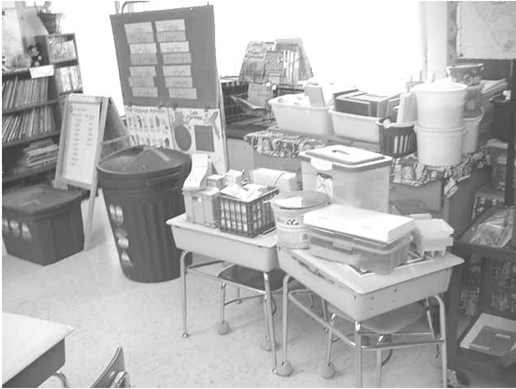
Classroom Items on and around Univent Obstructing Airflow
