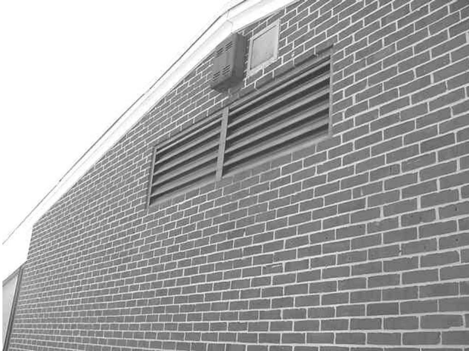
Exhaust Terminus Exterior of Building
