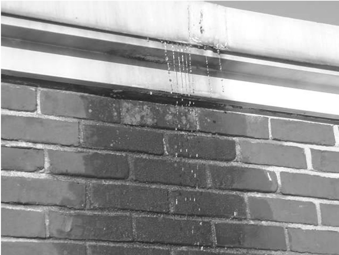
Water Staining and Moss Growth on Exterior Brick
