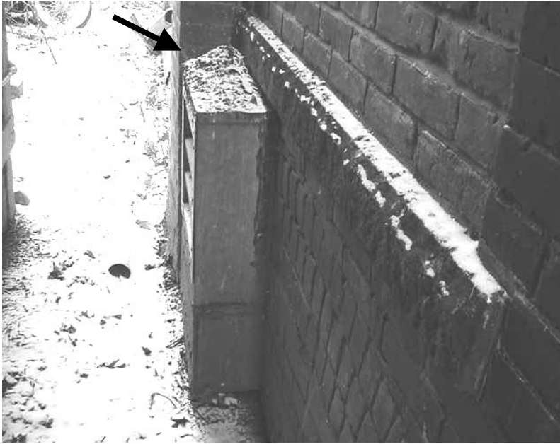
Accumulated Bird Waste in Alleyway
