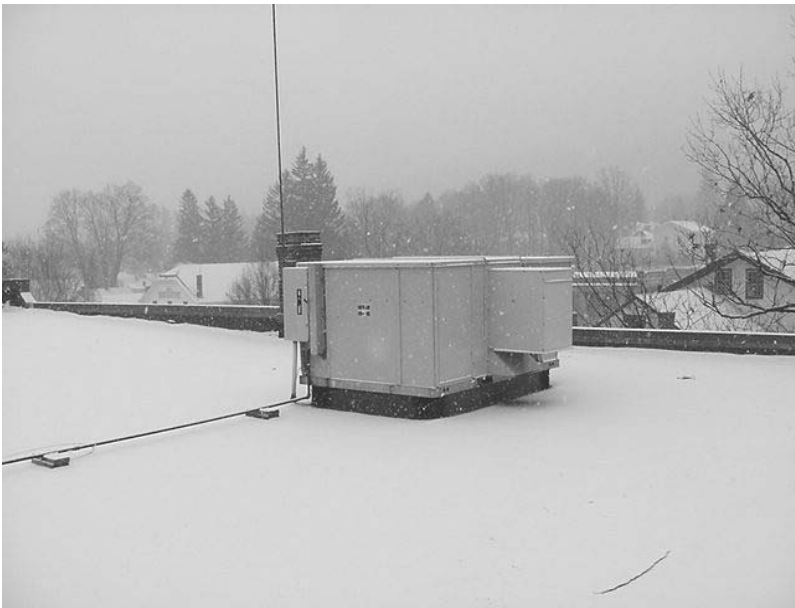
AHU for Auditorium
