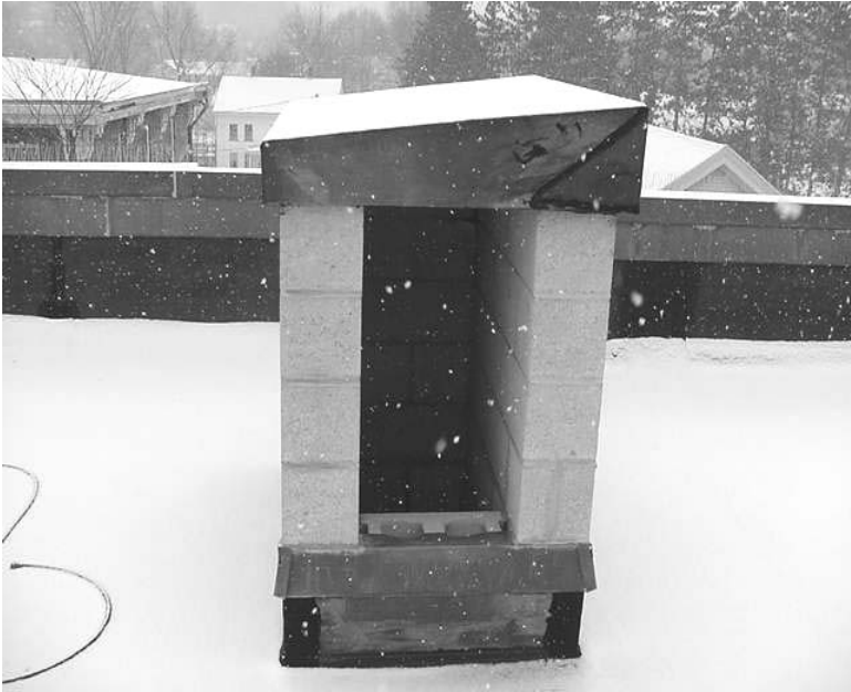
Elevator Shaft Pressure Equalization Vent, Note Lack of Bird Screen
