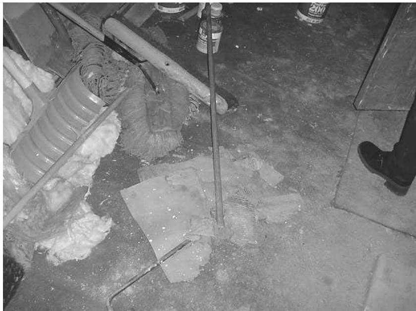
Materials Stored in Basement, Note Carpeting On Dirt Floor
