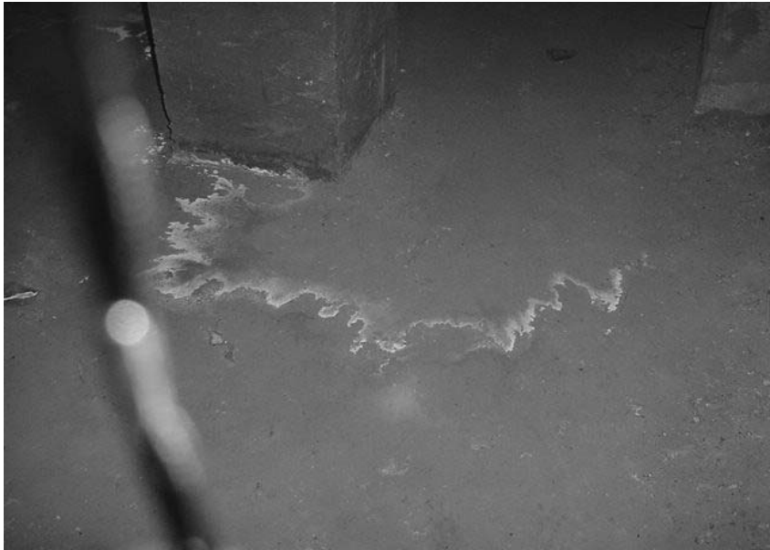
Basement Dirt Floor, Note Efflorescence
