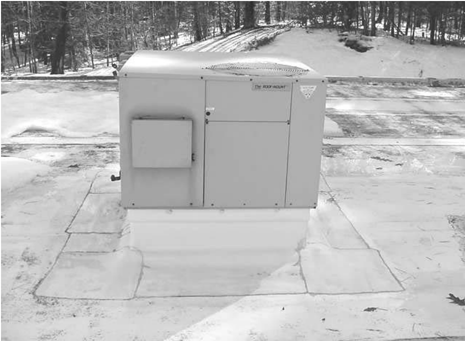
Modular Classroom AHU
