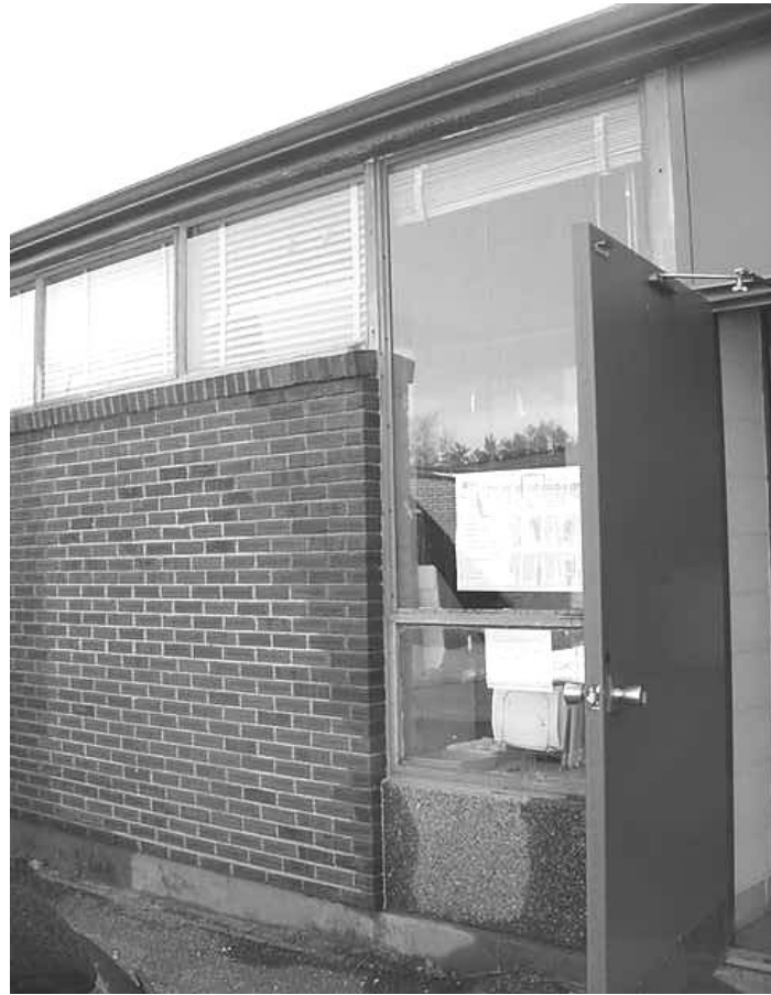
Water Dripping Through a Hole in the Gutter Wetting the Sill, Window Frame and Exterior Wall
