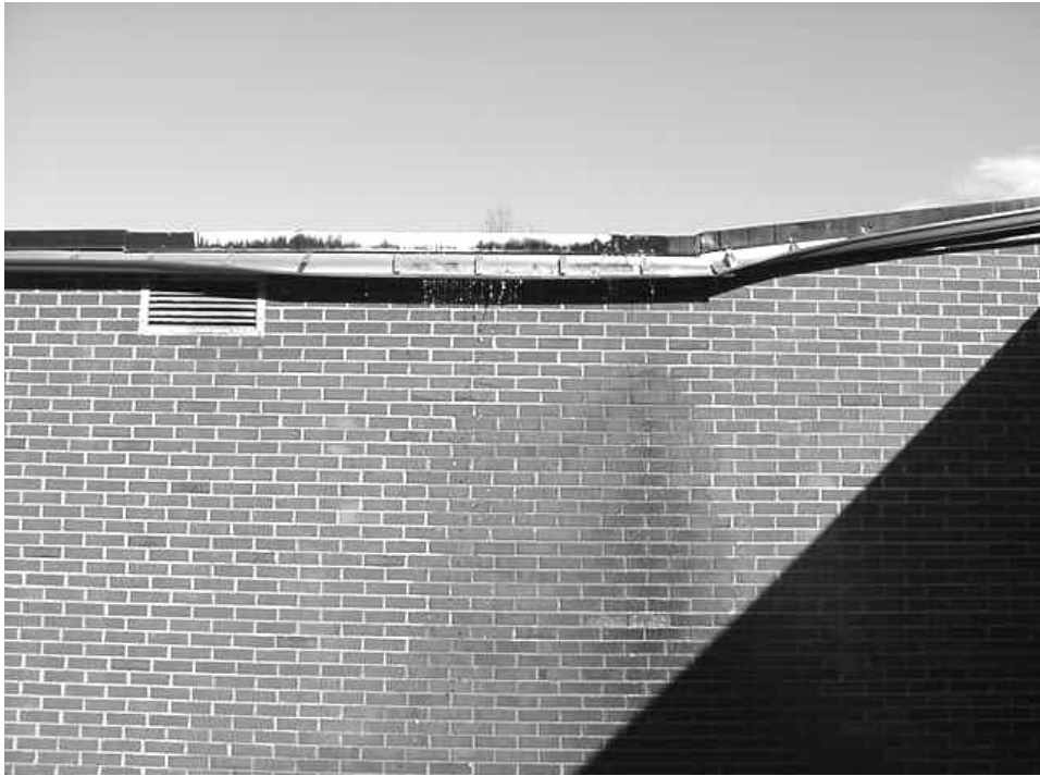
Damaged Gutter Wetting the Exterior Wall System
