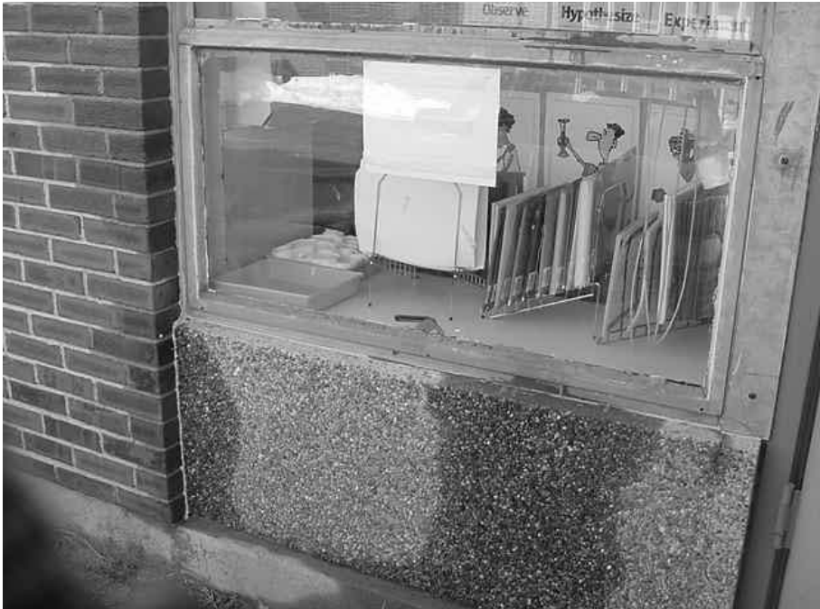
Close Up Of Water Damage in Picture 3
