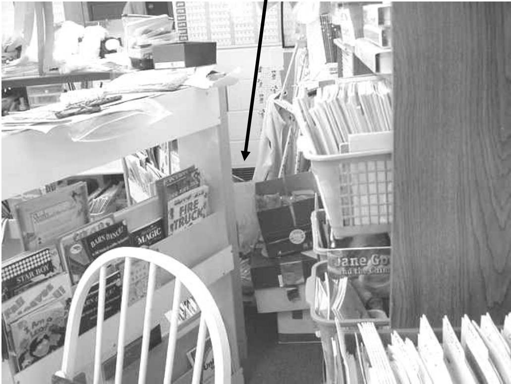
Classroom Exhaust Vent Blocked by Various Items
