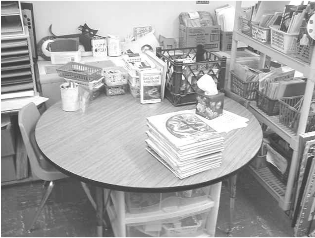
Univent Obstructed by Items on and in Front of Unit
