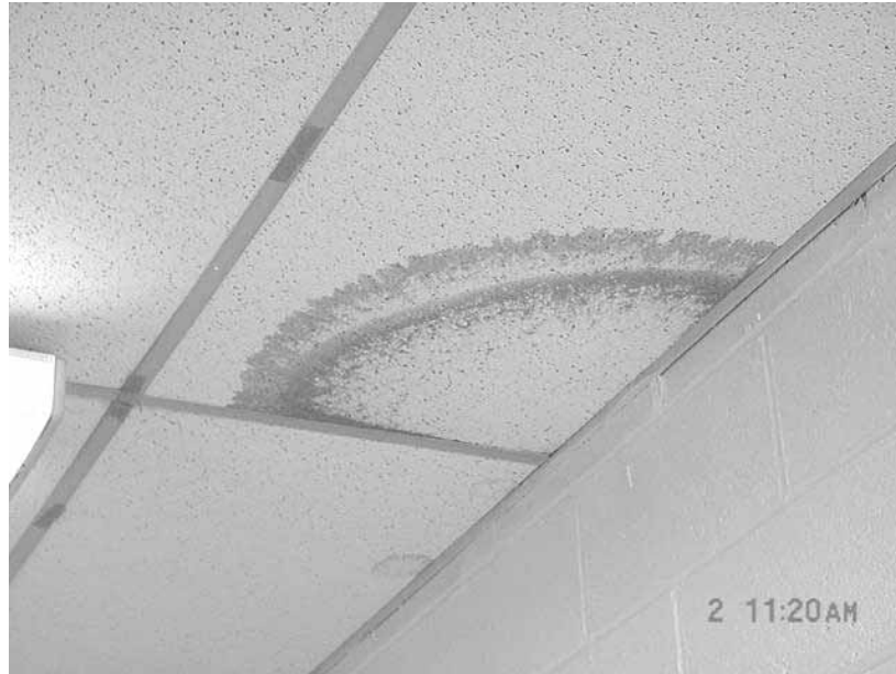
Water Damaged Ceiling Tile in Classroom
