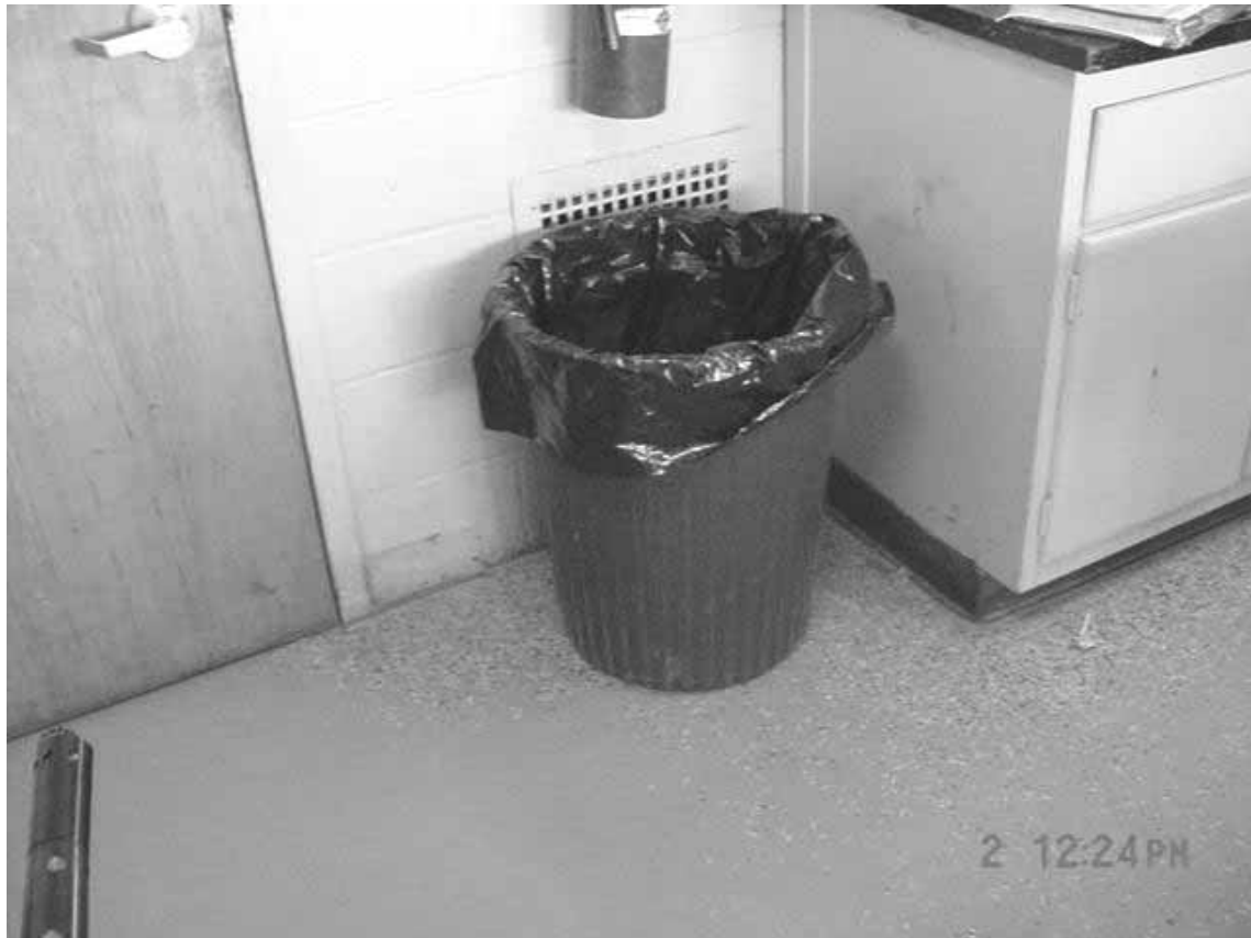
Classroom Exhaust Vent Obstructed by Trash Barrel
