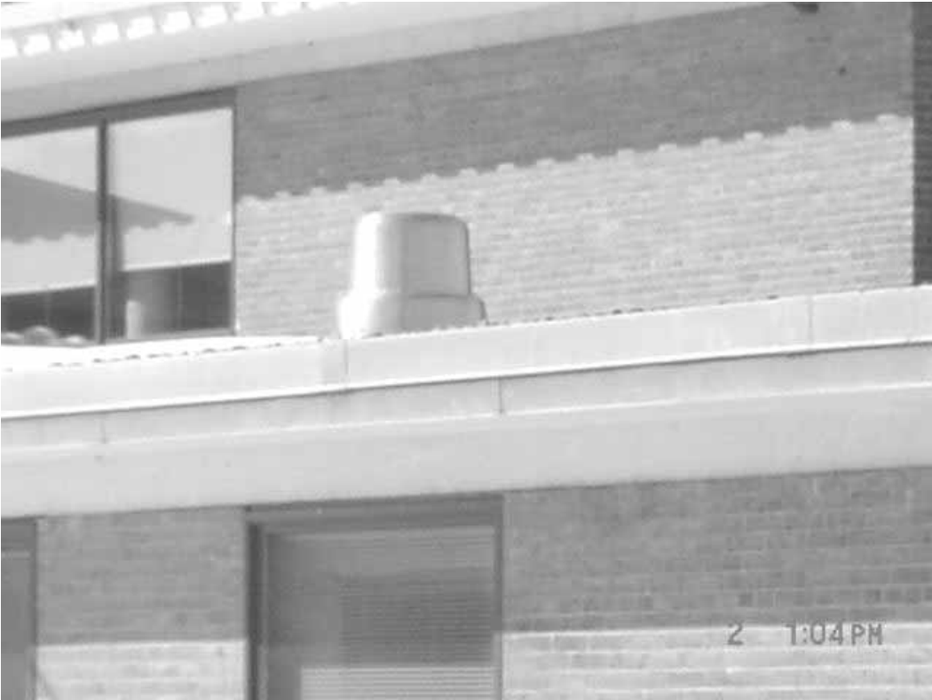
Rooftop Exhaust Motor
