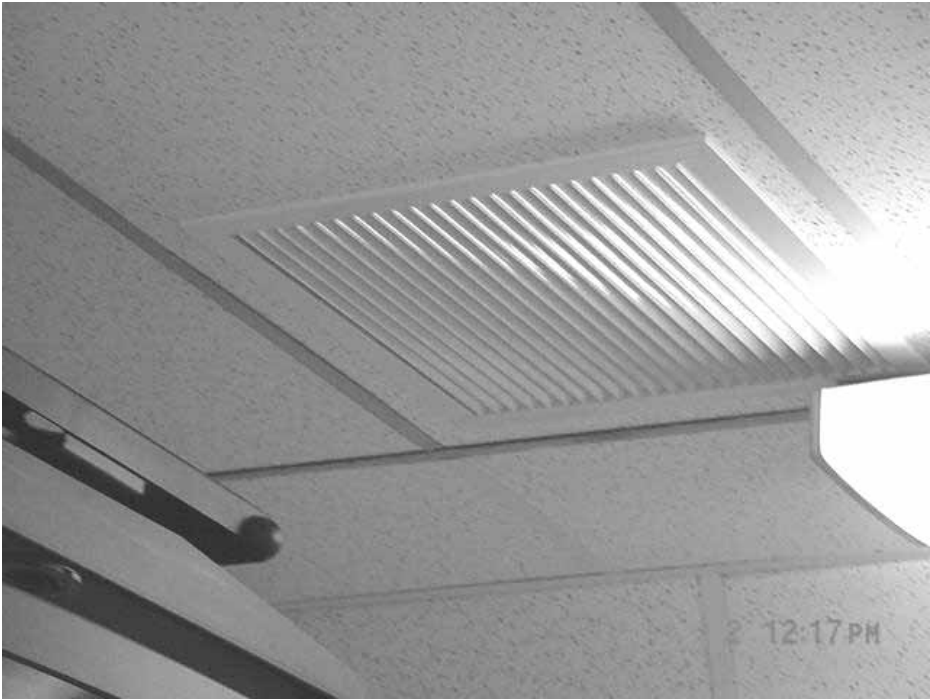
Ceiling-Mounted Return Vent
