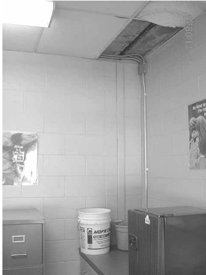
Active Roof Leak in Tutor's Room, Note Missing Tile and Bucket
