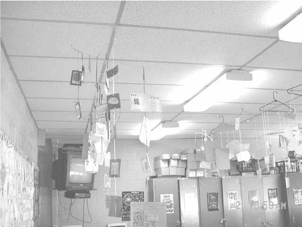
Items Hanging Form Ceiling Tiles in Classroom
