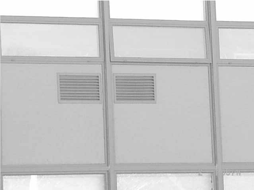
Univent Air Intakes
