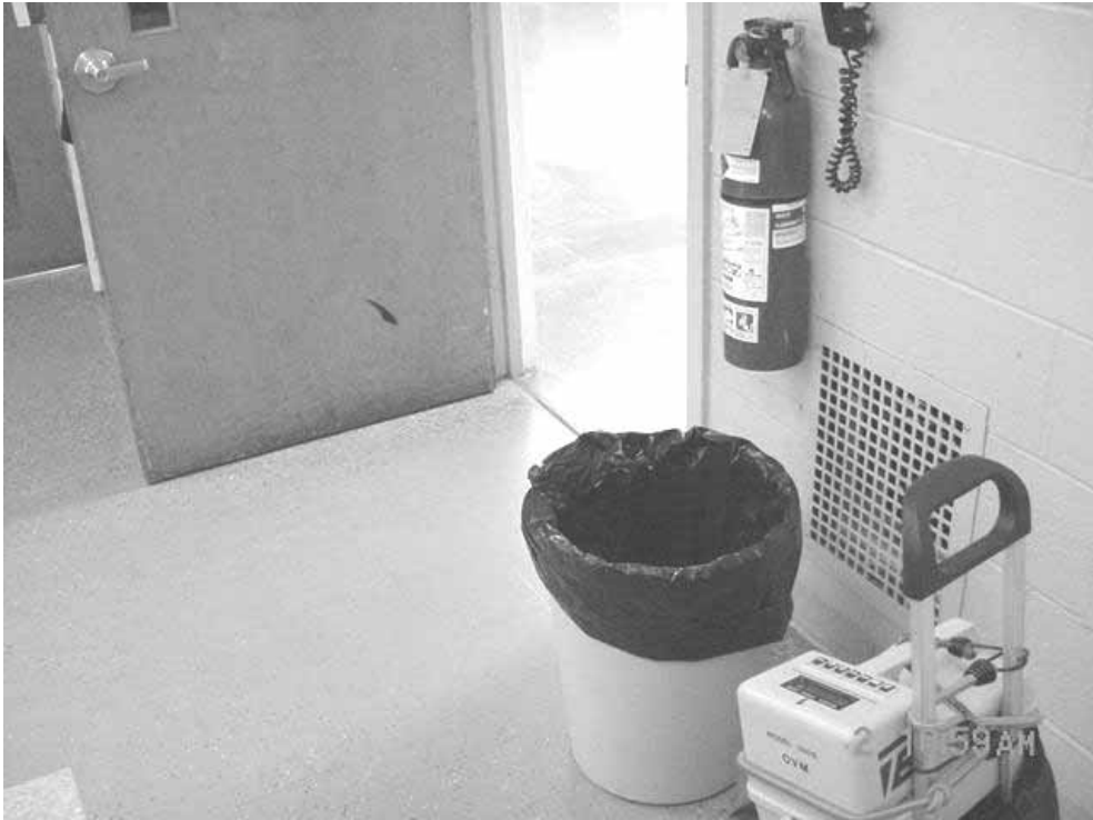
Classroom Exhaust Vent, Note Proximity to Open Hallway Door
