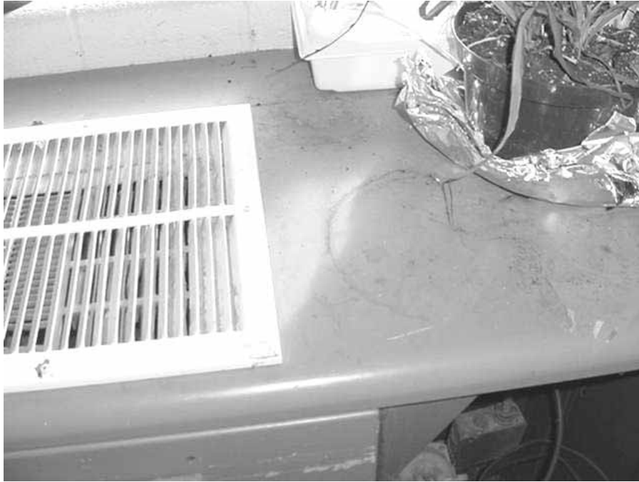
Plants placed near ventilation univent, note debris
