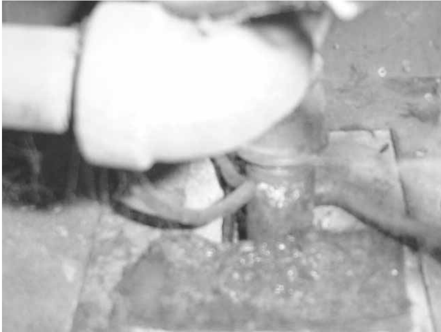
Spaces around pipes in univent air handling cabinet
