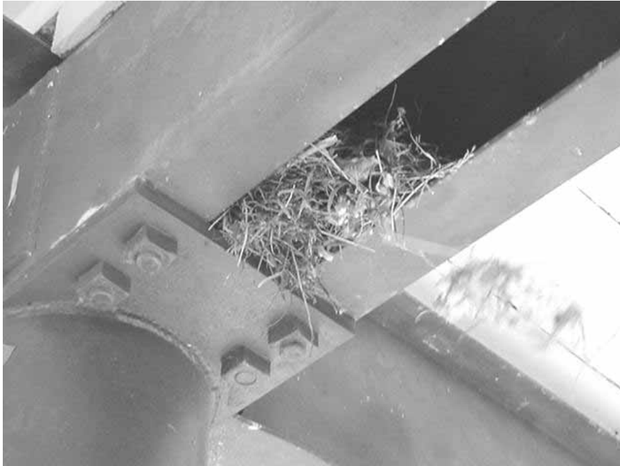
Bird's nest in support beam
