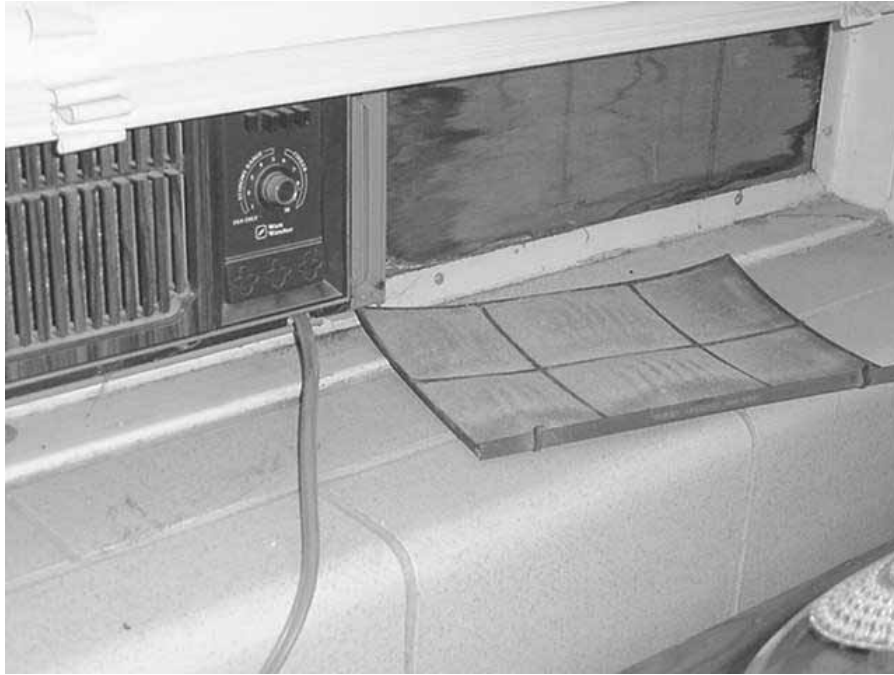
Air conditioner filter occluded with debris
