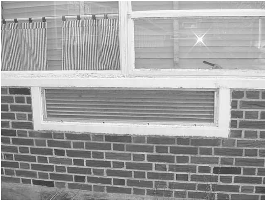
Univent fresh air intake
