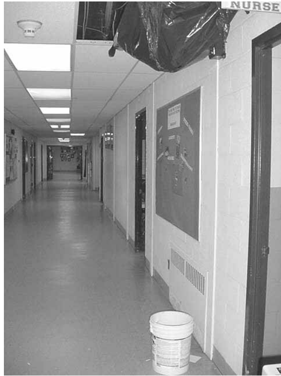
Missing ceiling tile for water drainage to bucket
