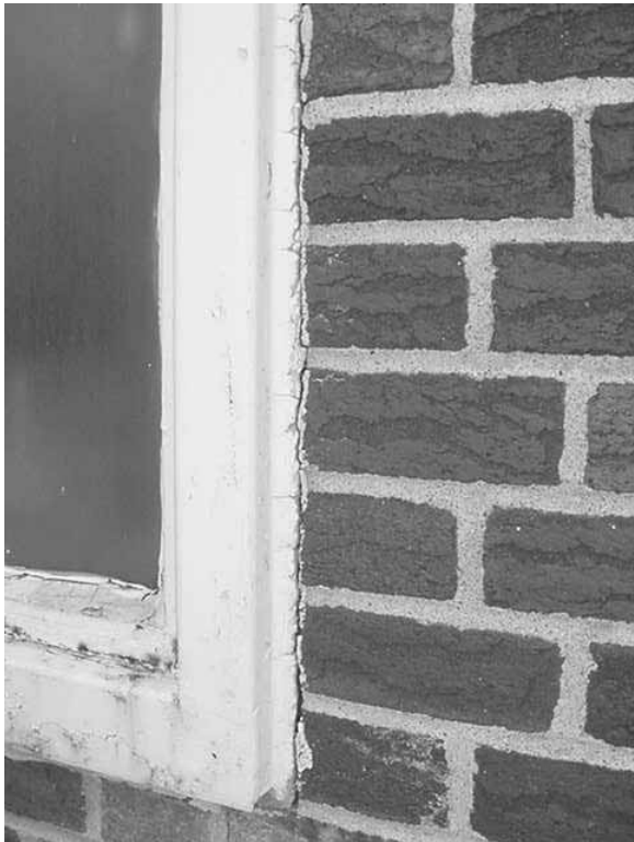
Spaces around window frame
