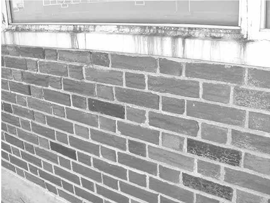
Water damage to exterior of window frame
