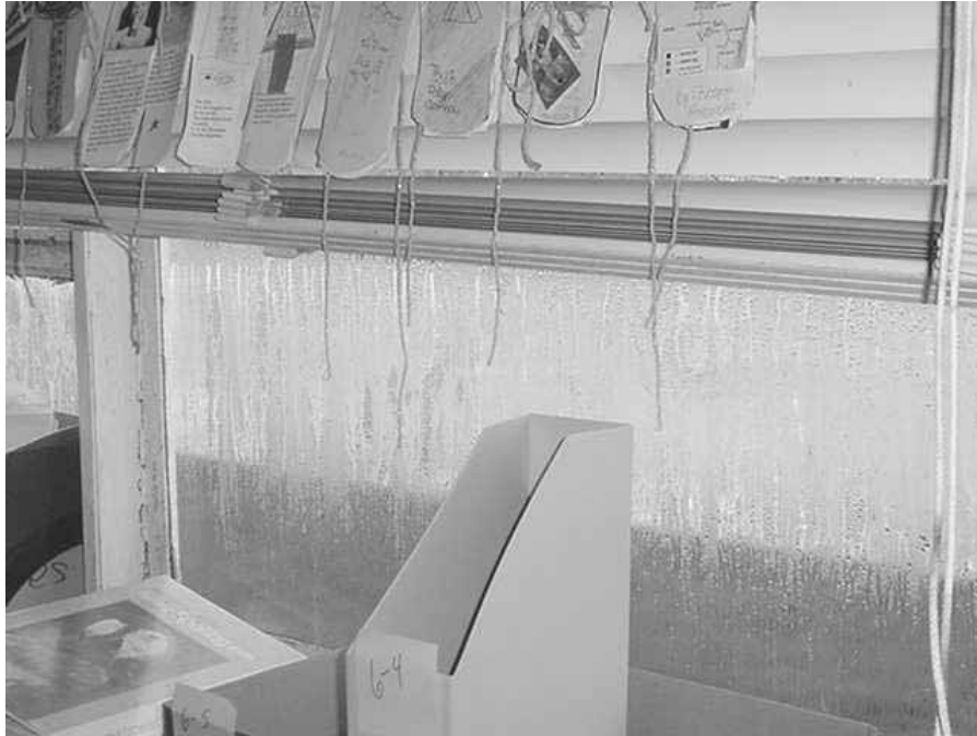
Interior view of condensation on classroom window
