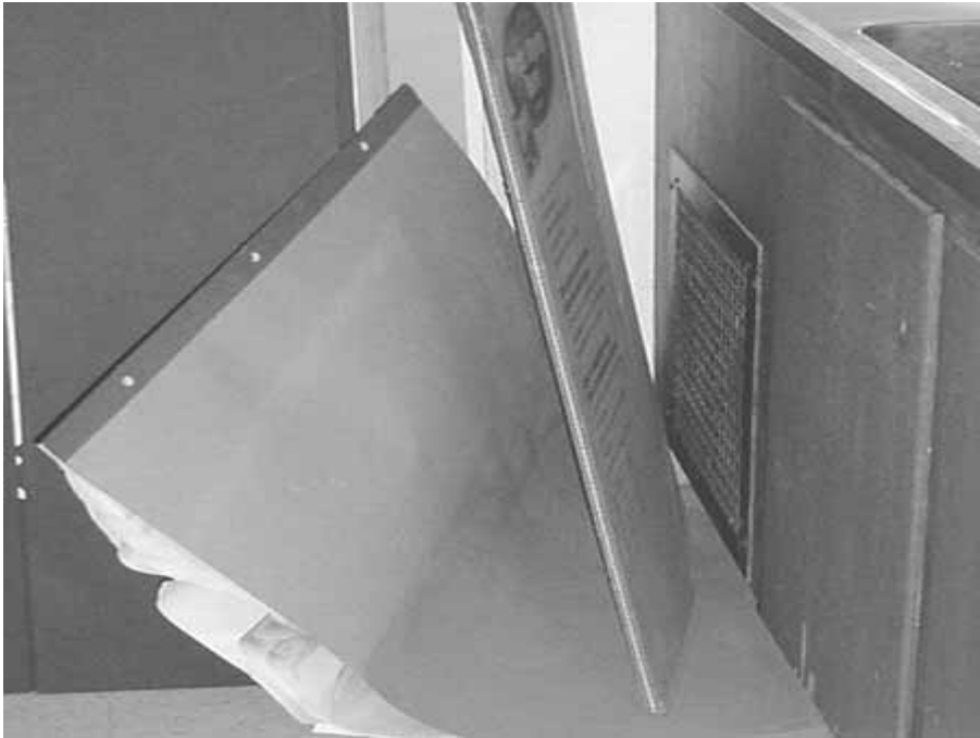
Blocked exhaust vent
