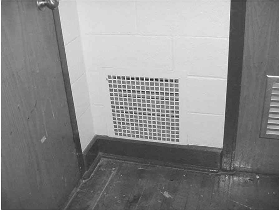
Exhaust vent proximity to door
