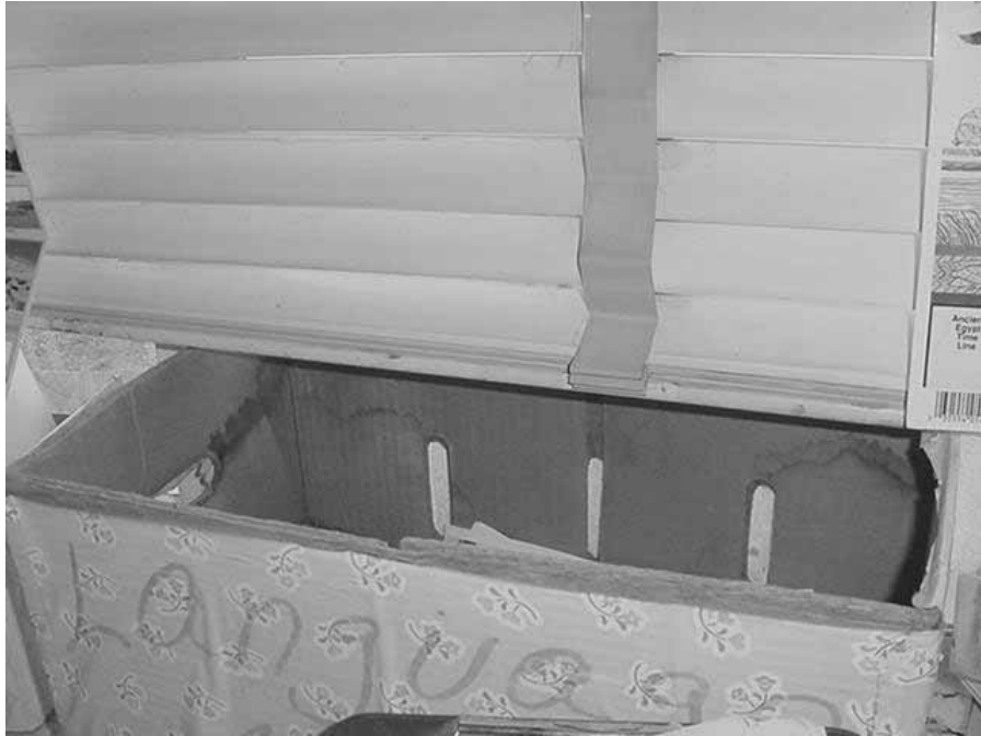
Water damaged materials
