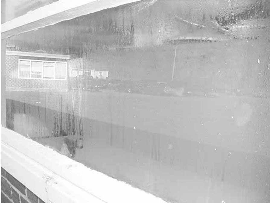
Exterior view of condensation on classroom window
