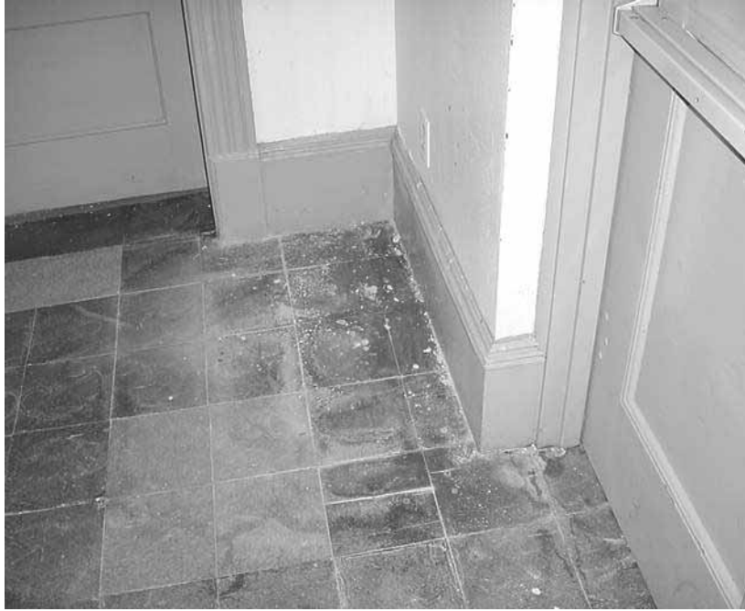
Water Damage Floor Tile in Hallway, Second Floor
