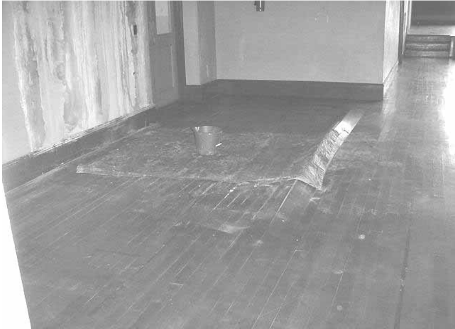
Water Damaged Floor, Third Floor
