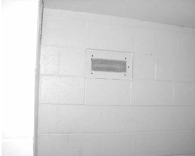
Exhaust Vent, Holding Cell
