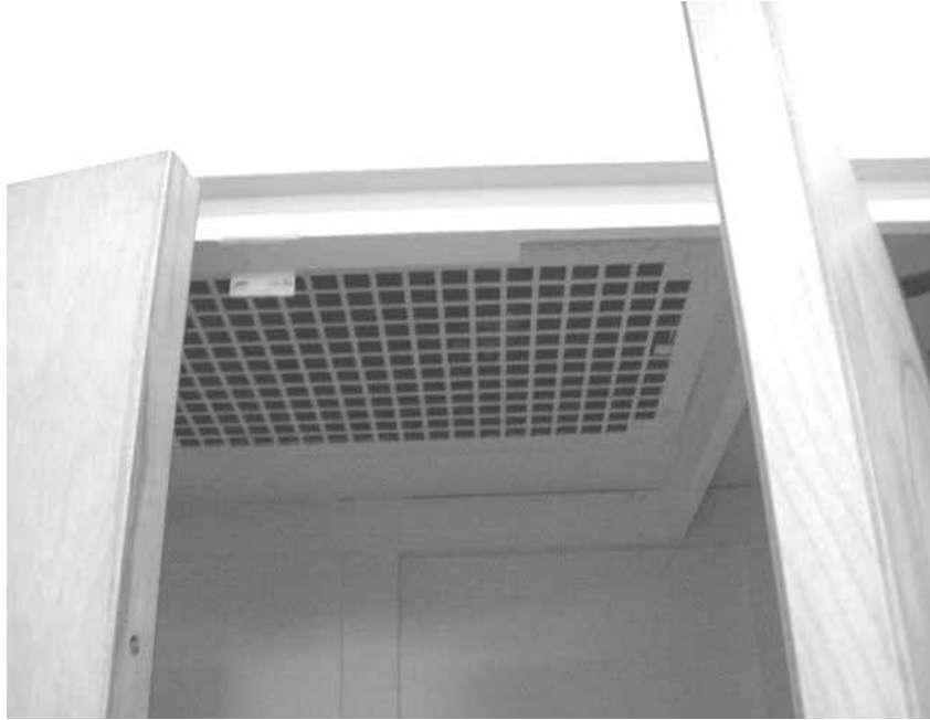
Original Exhaust Vent System in Closets
