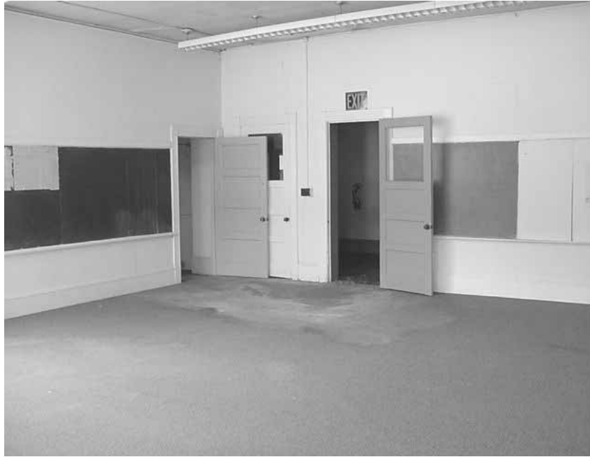
Water Damaged Carpet, Second Floor
