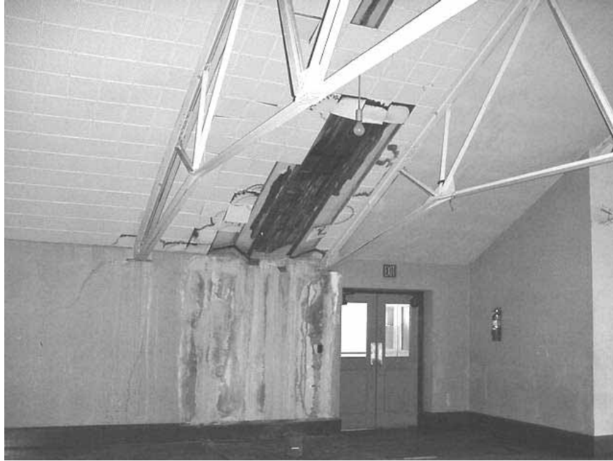
Water Damage to Ceiling, Third Floor
