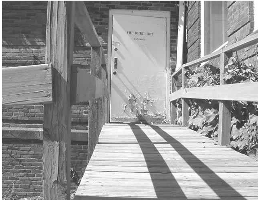
Water Damage to Access Ramp Door, Above the Holding Cell
