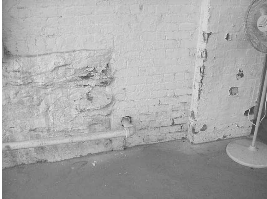
Water Damage to Holding Area Base of Wall, In an Area of the Foundation below Grade
