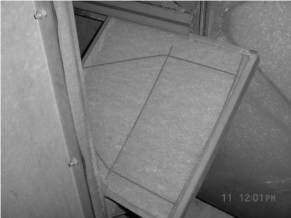
Fibrous Mesh Filters Installed in AHUs
