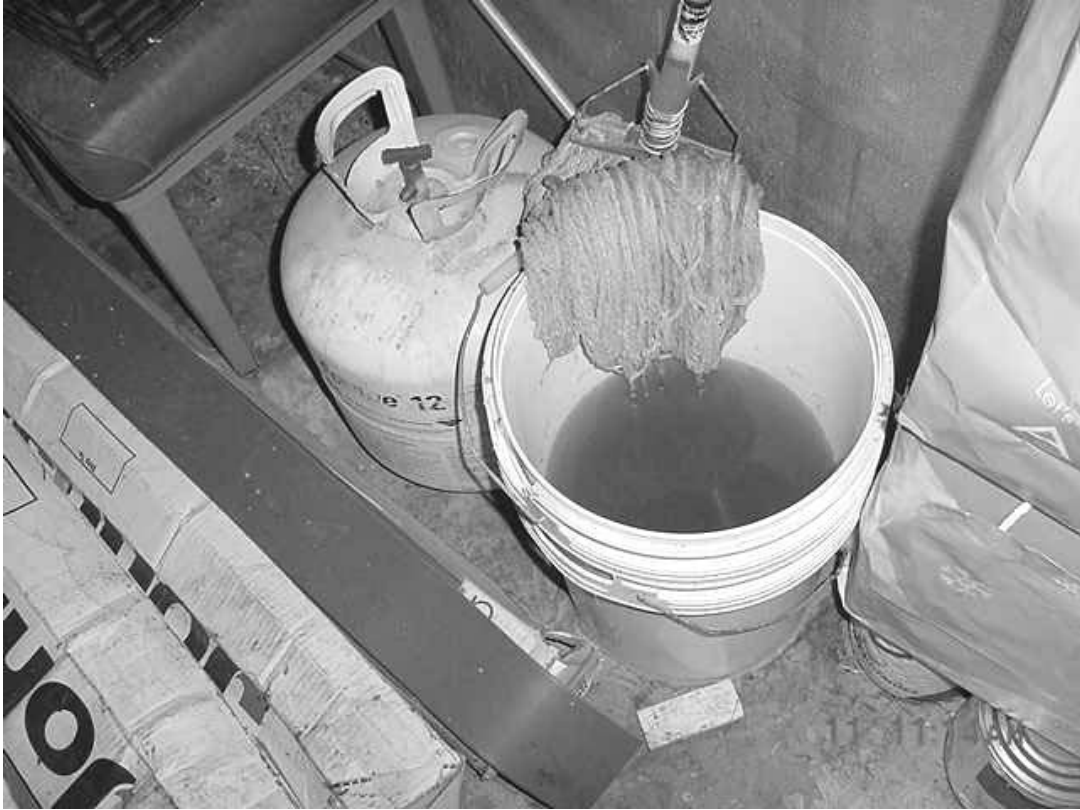
Mop and Buckets in Mechanical Room near Kitchen, also note Propane Tank
