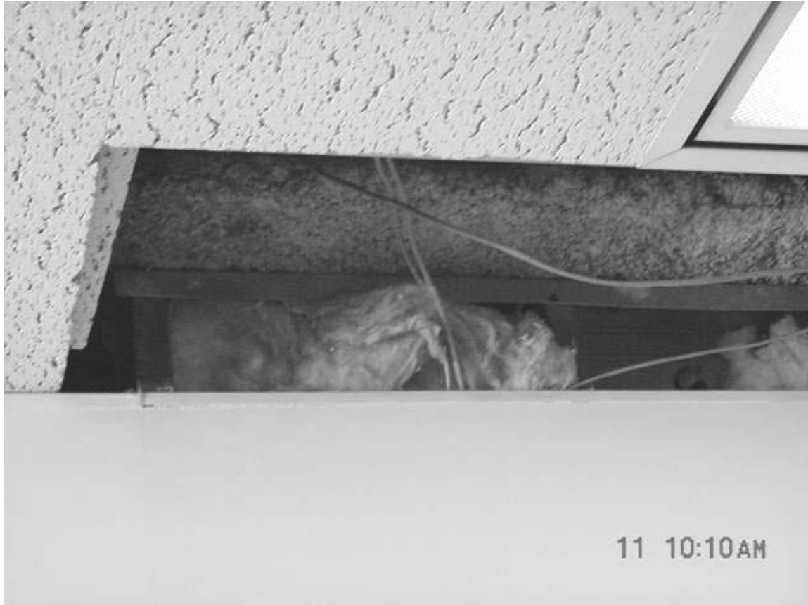
Missing Ceiling Tiles Exposing Fiberglass Insulation
