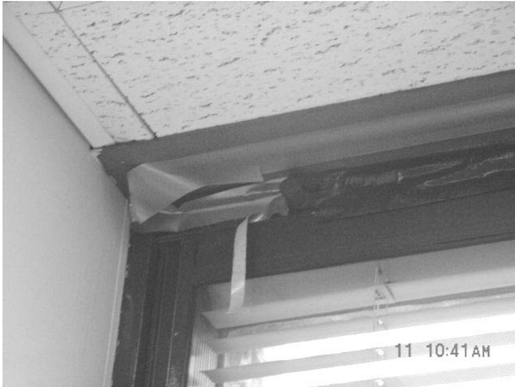
Duct Tape around Window Frames in Malden School Department
