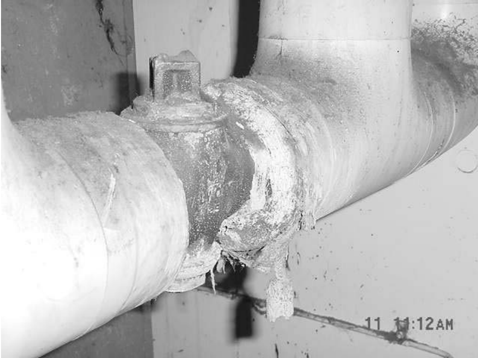
Exposed Insulation Material in Mechanical Room near Kitchen
