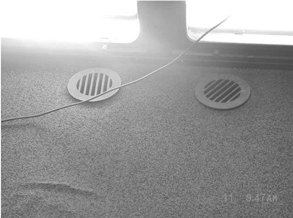
Floor Supply Vents
