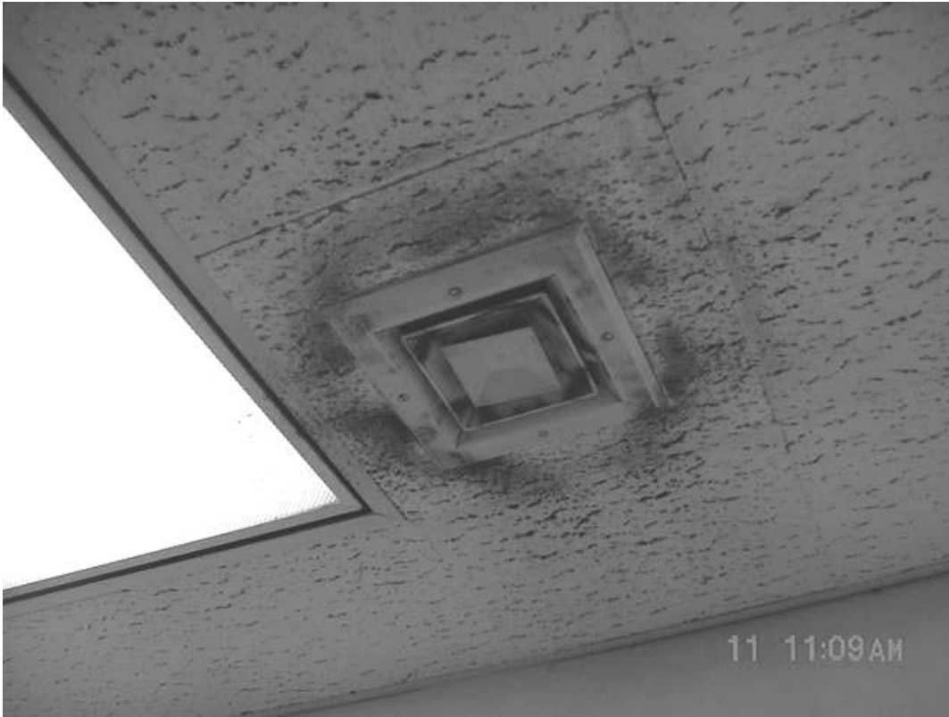
Dust/Debris Deposition around Supply Vent in Kitchen/Cafeteria
