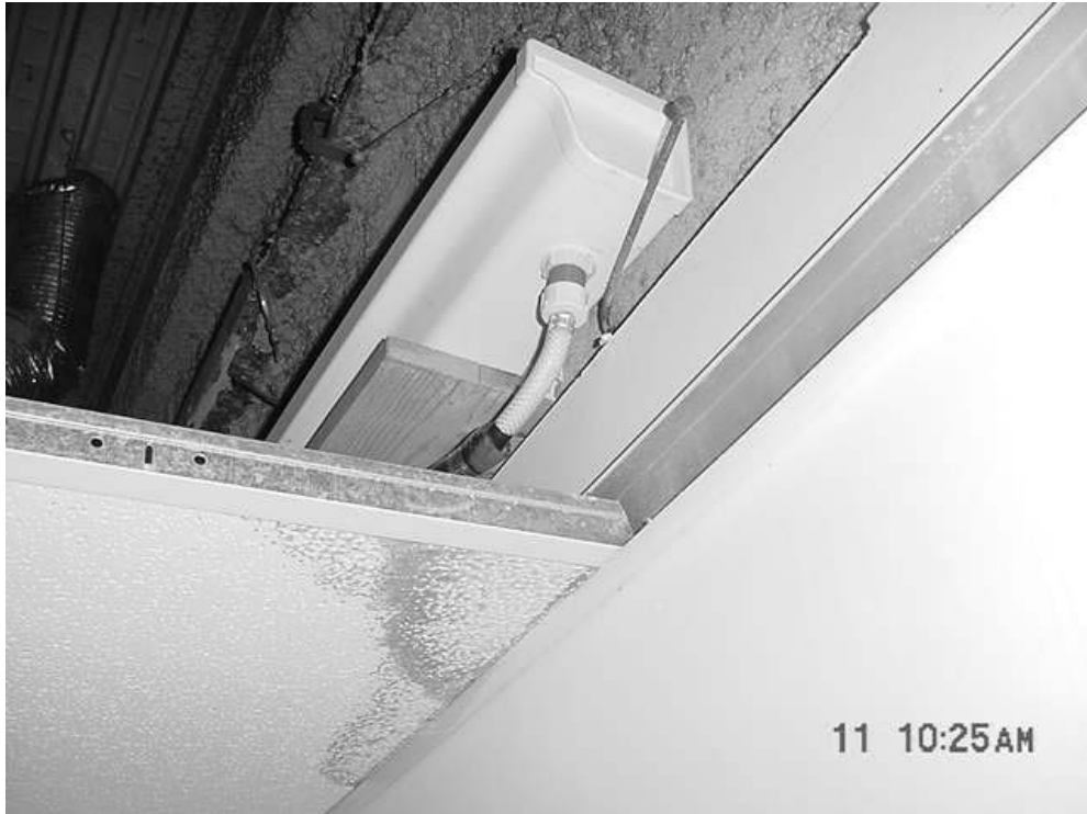
Temporary Drainage System above Ceiling Tiles in the Personnel/Retirement Area, Note Drain at Bottom of Gutter
