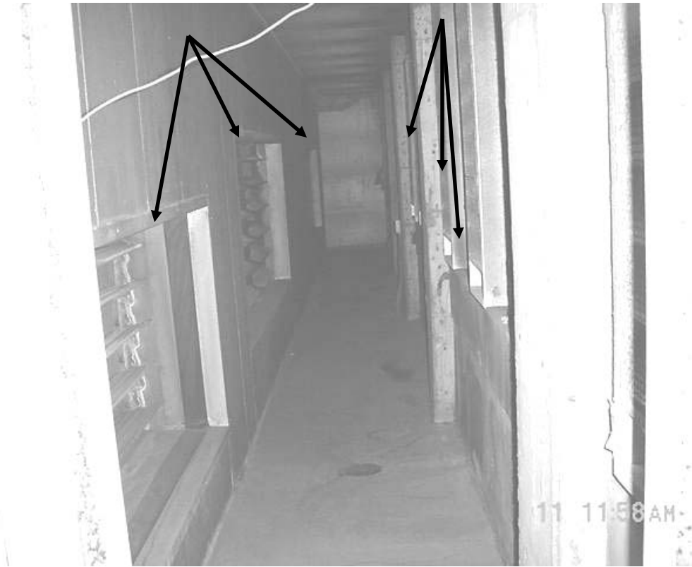
Fresh Air Ventilation Duct
