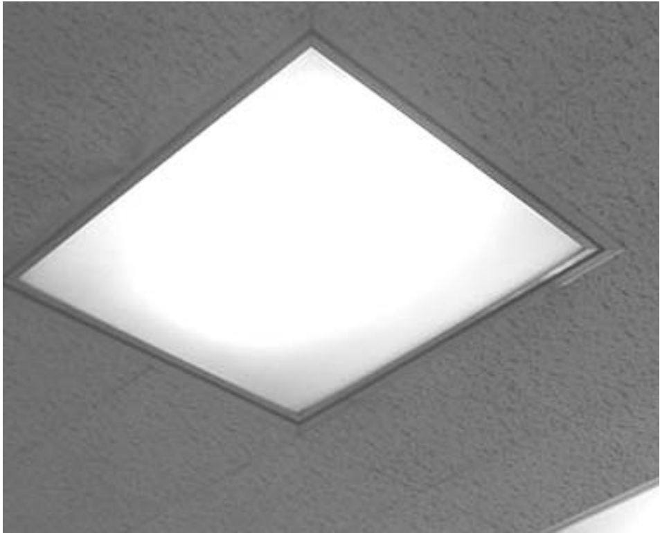
Slotted Vents around Light Fixtures
