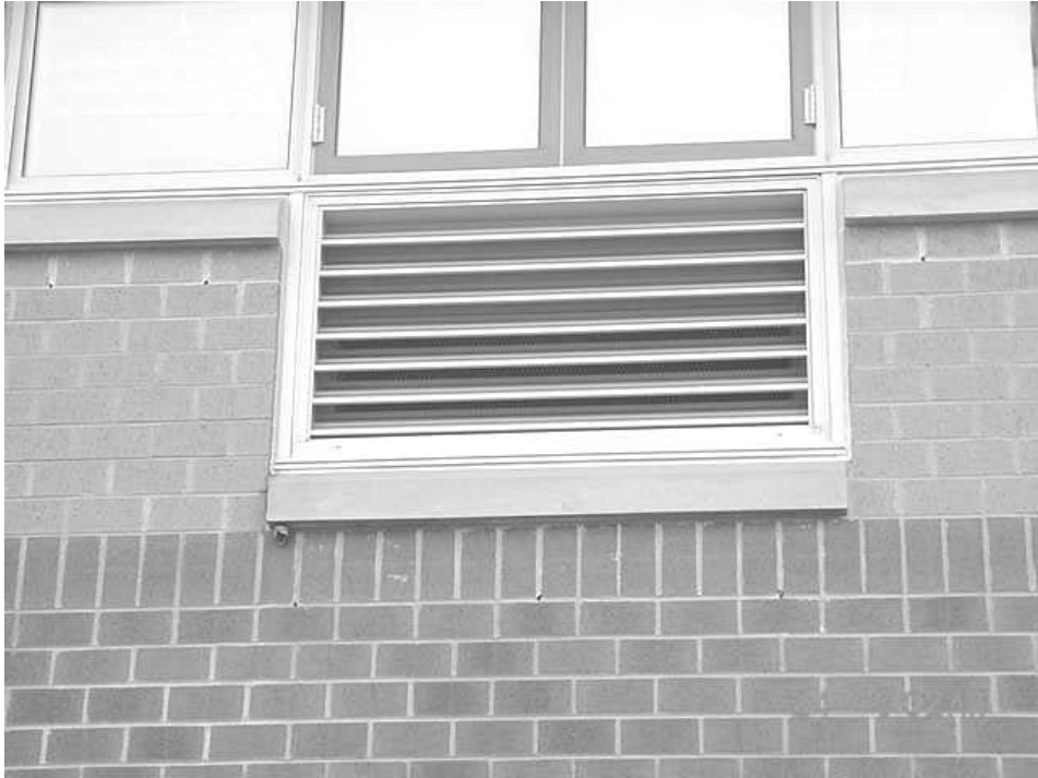
Univent Fresh Air Intake
