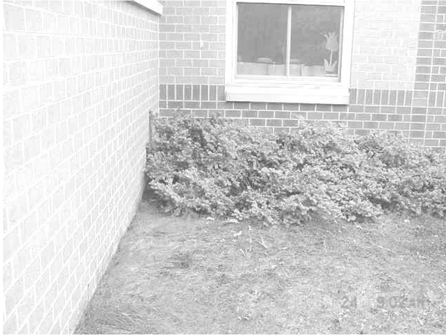
Plants/Shrubbery Growing against Exterior Walls
