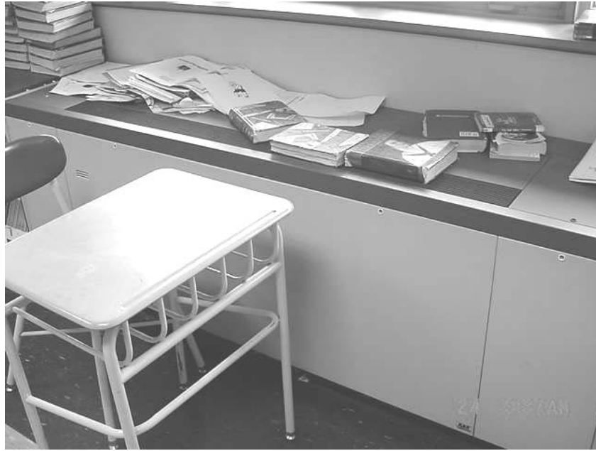
Classroom Univent, Note Books on Air Diffuser
