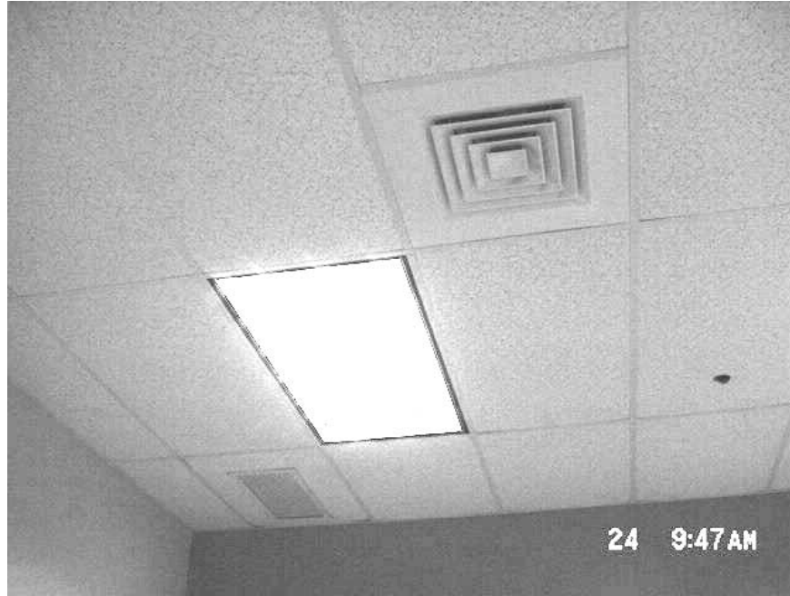
Supply and Return Vent Ducted to Rooftop AHU
