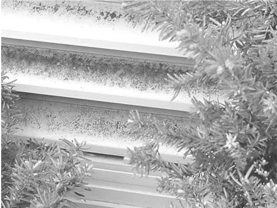
Plant Debris/Mold on Univent Fresh Air Intakes Louvers
