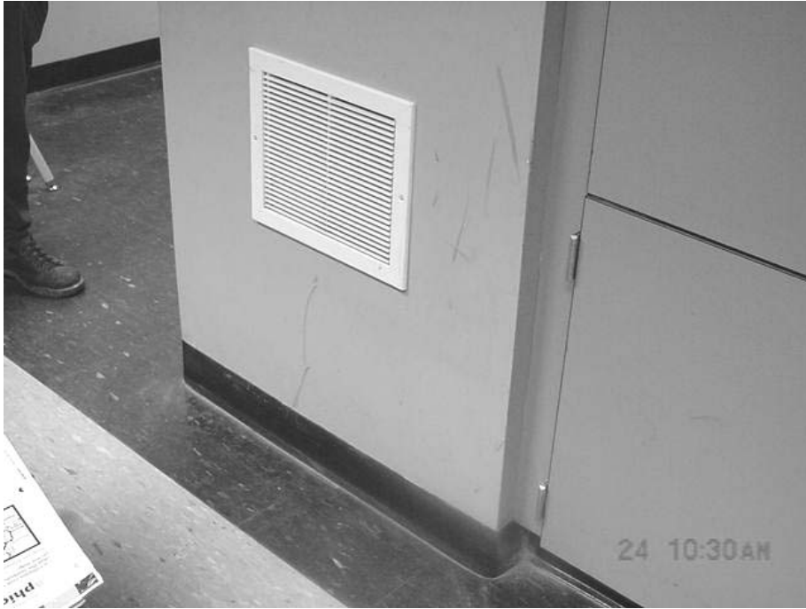
Wall-Mounted Exhaust Vent
