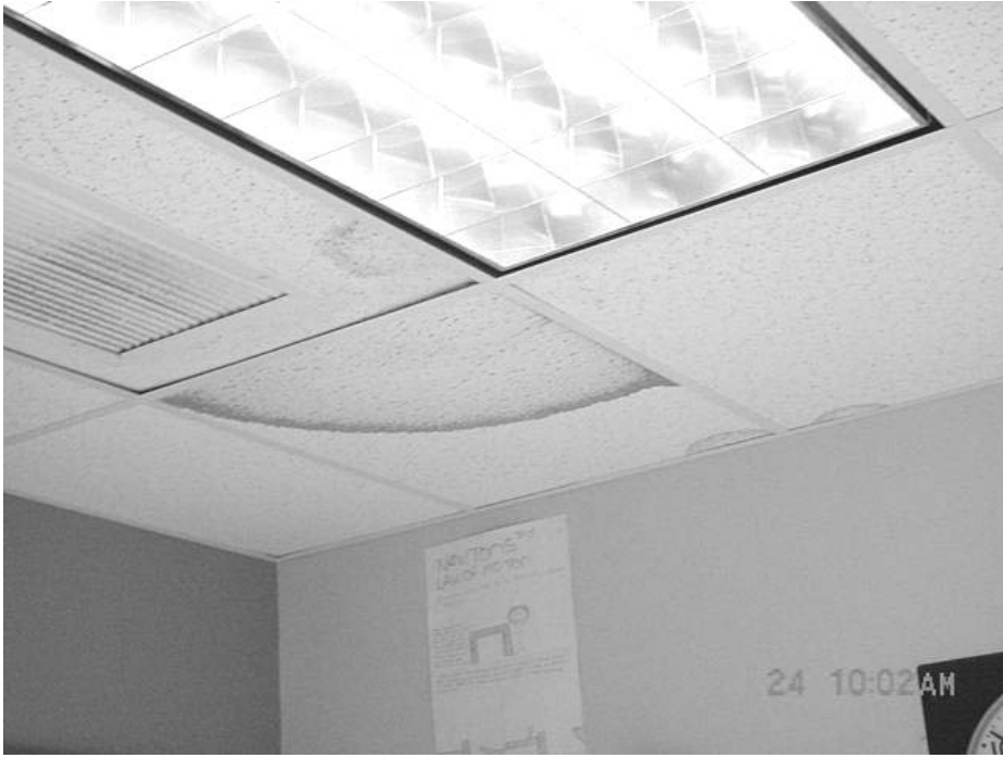
Water Damaged Ceiling Tiles in Classroom
