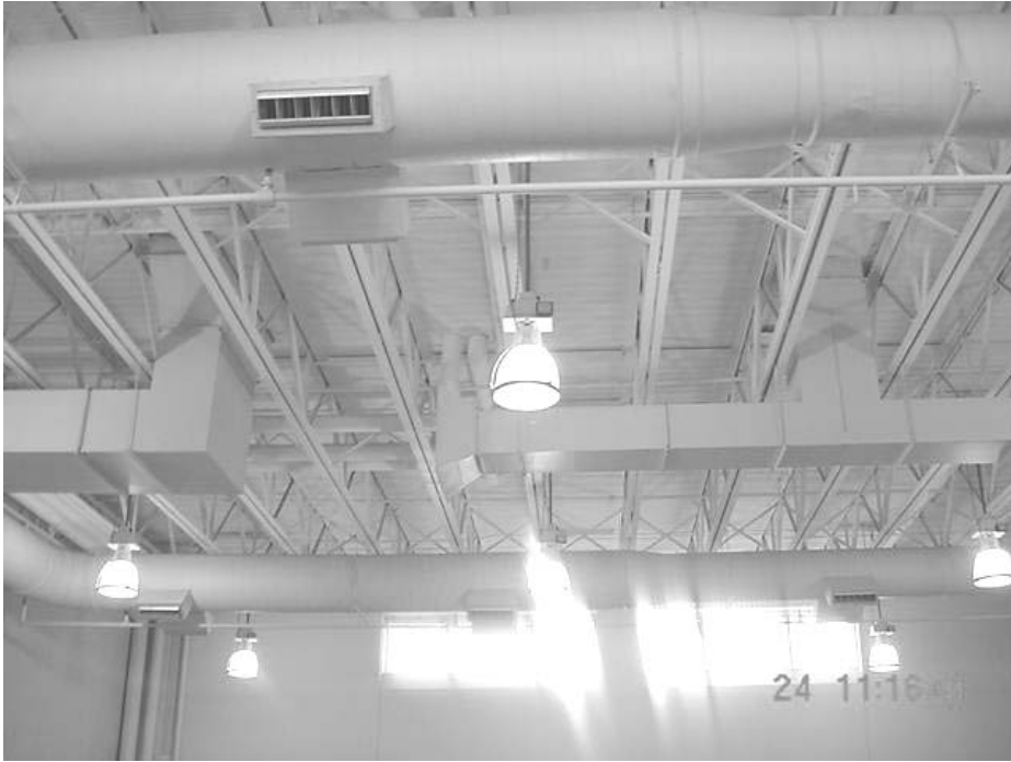
Ducted Supply and Return Vents in Gymnasium
