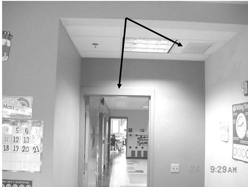
Ceiling-Mounted Exhaust Vent in Classroom, Note Proximity to Open Hallway Door
