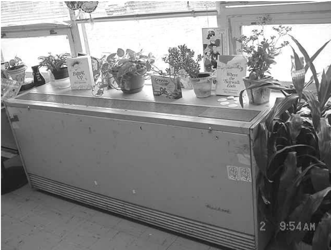
Classroom Univent, 1960s Vintage, Note Plants near Air Diffuser
