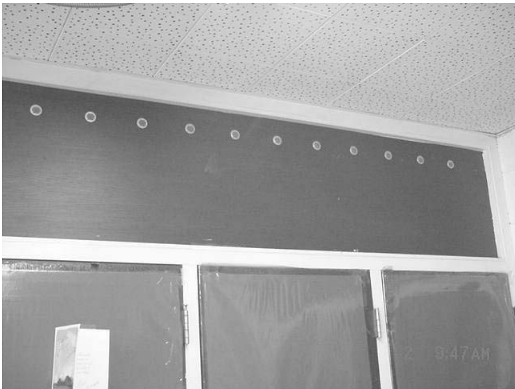
Small Round Vents Installed in an Attempt to Increase Airflow into Coat Closet Vents
