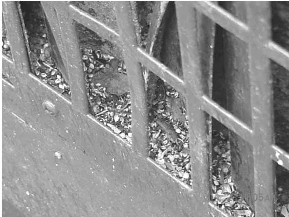
Plant Debris and Bird Seed in Univent Air Intake outside of Classroom 18
