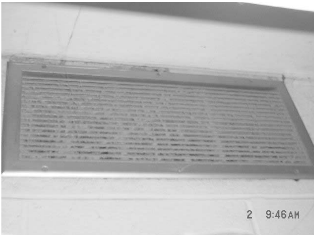
Exhaust Vent in Top of Classroom Coat Closet, Note Dust Build-Up
