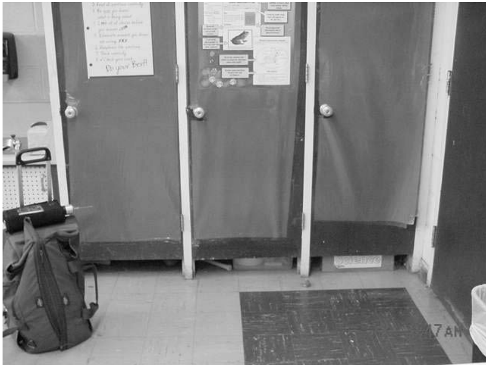
Long-View of Undercut Coat Closet, Note Materials at Bottom Obstructing Airflow
