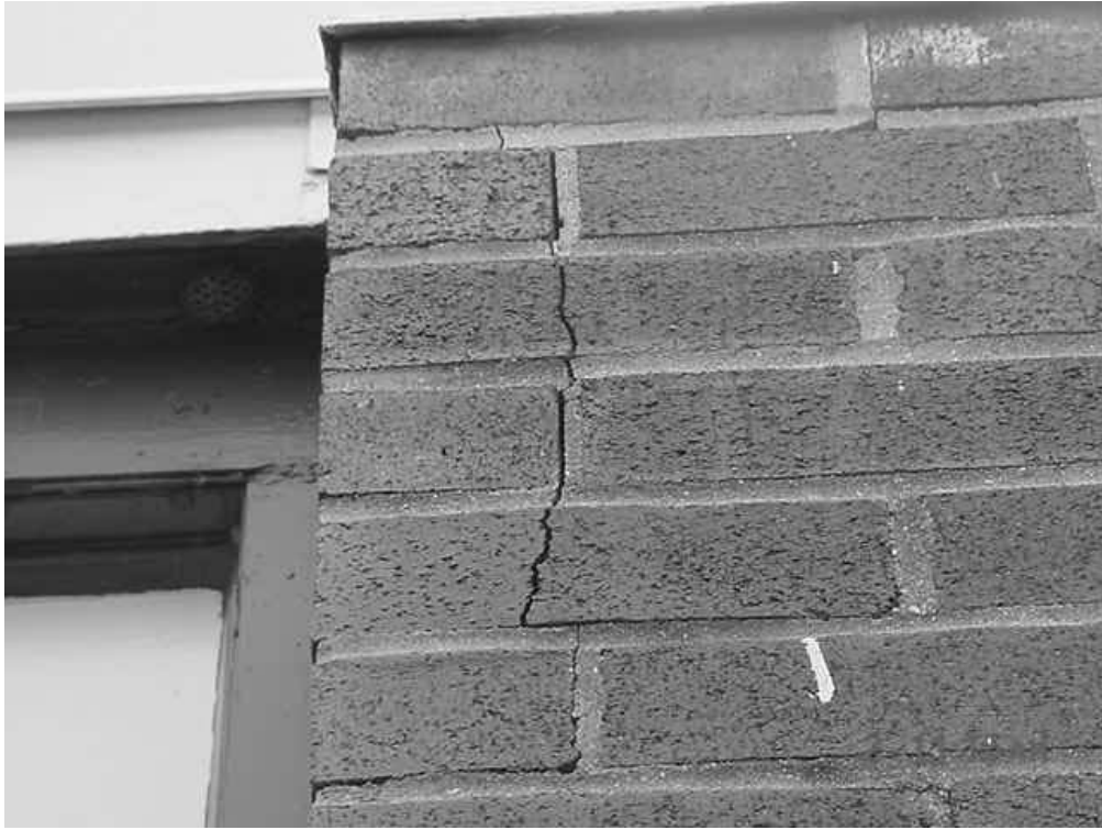
Exterior Wall Crack on Rear of Building
