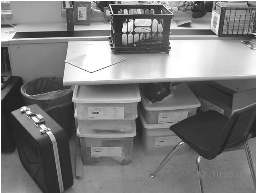
Obstructed Univent Return Vent (along front of unit)
