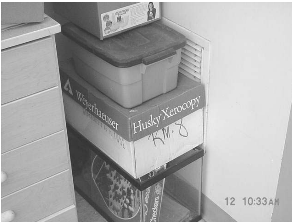
Classrooms Items Obstructing Exhaust Vent
