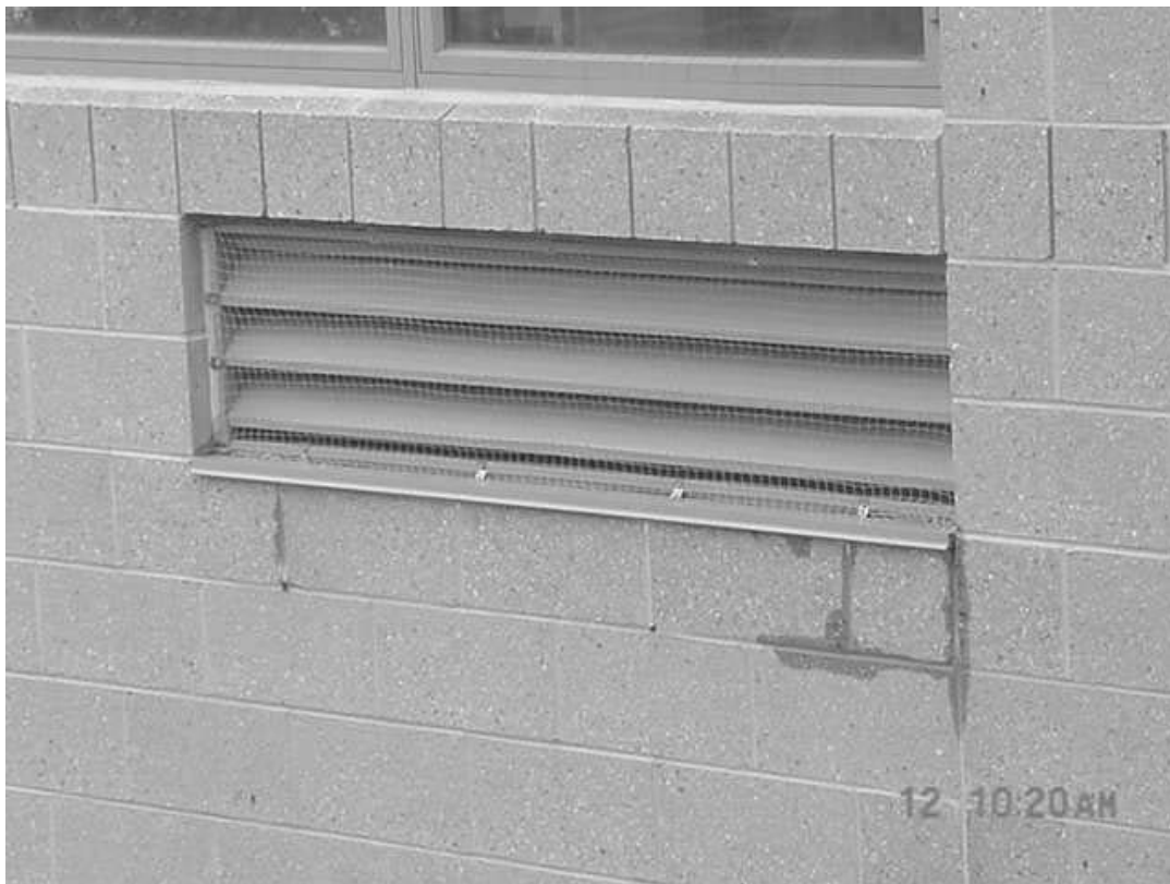
Univent Fresh Air Intake
