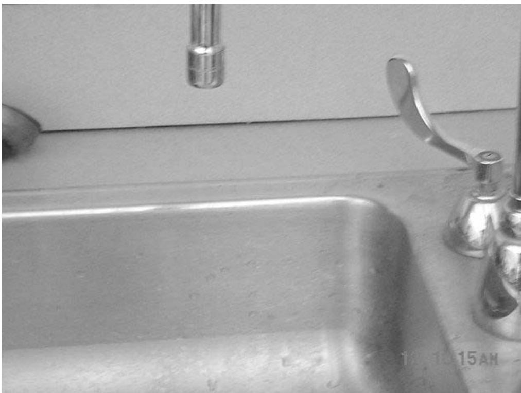
Space between Sink Countertop and Backsplash
