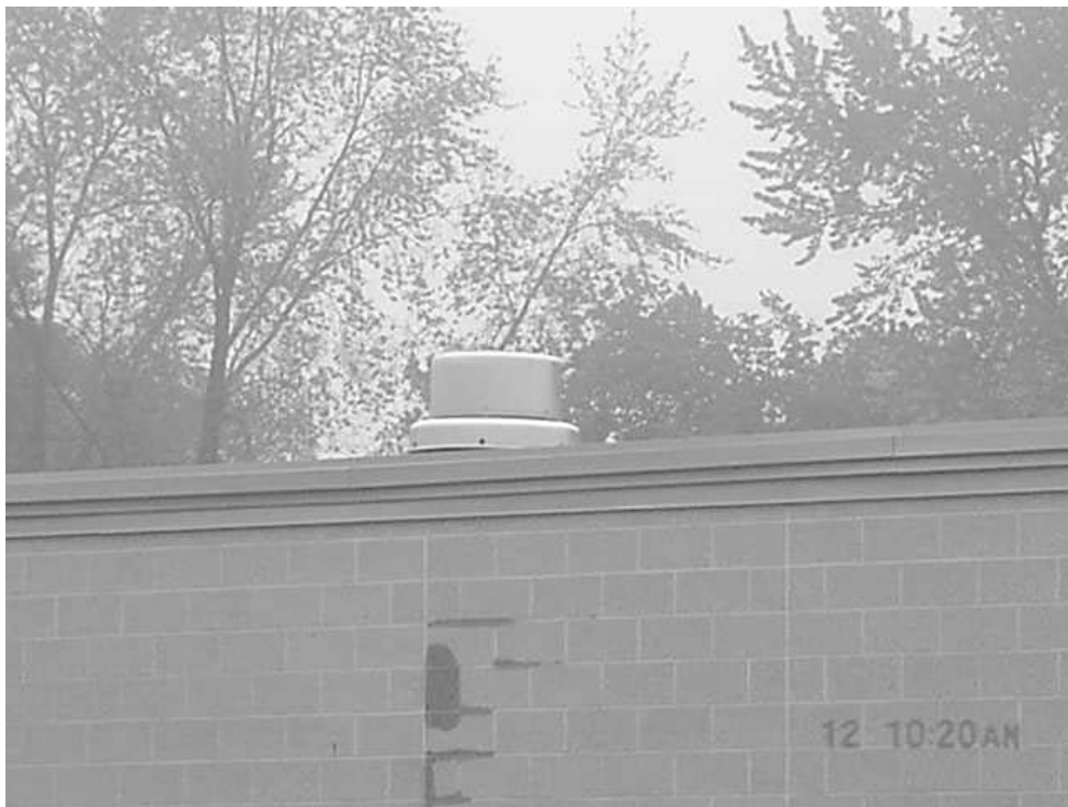
Rooftop Exhaust Motor
