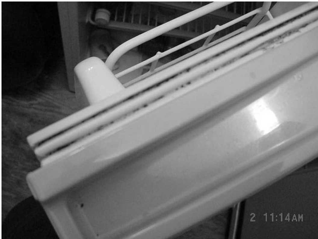
Mold Growth (as Indicated by Black Areas) along Refrigerator Gasket
