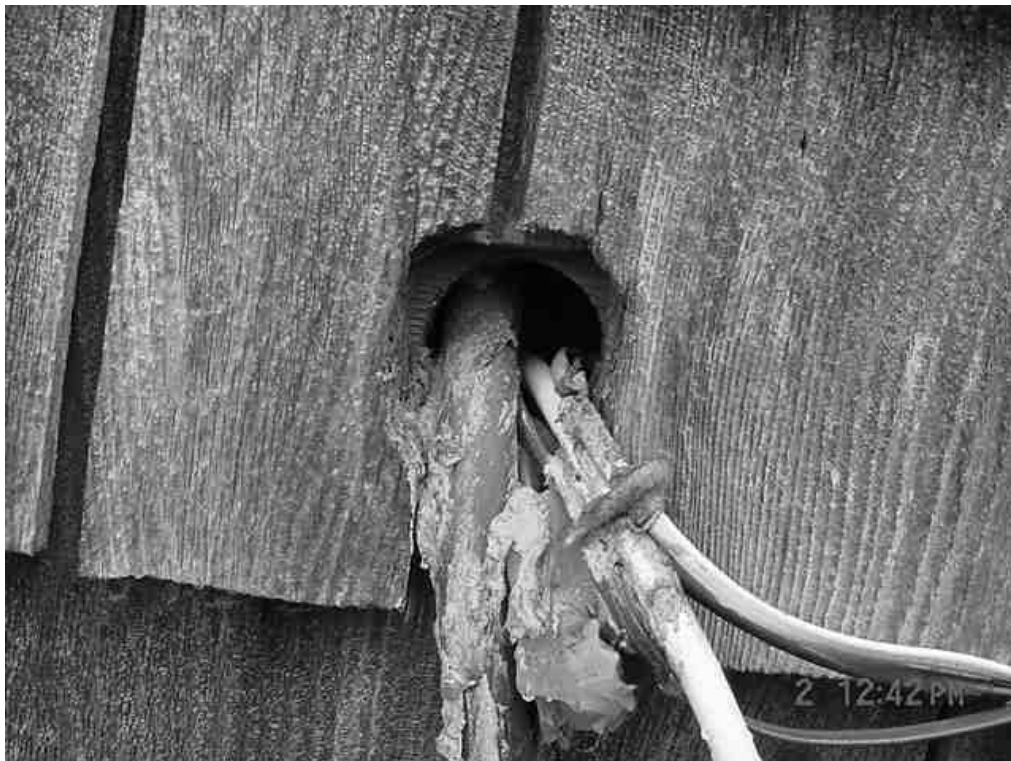
Open Utility Hole/Egress for Pests/Rodents into Building
