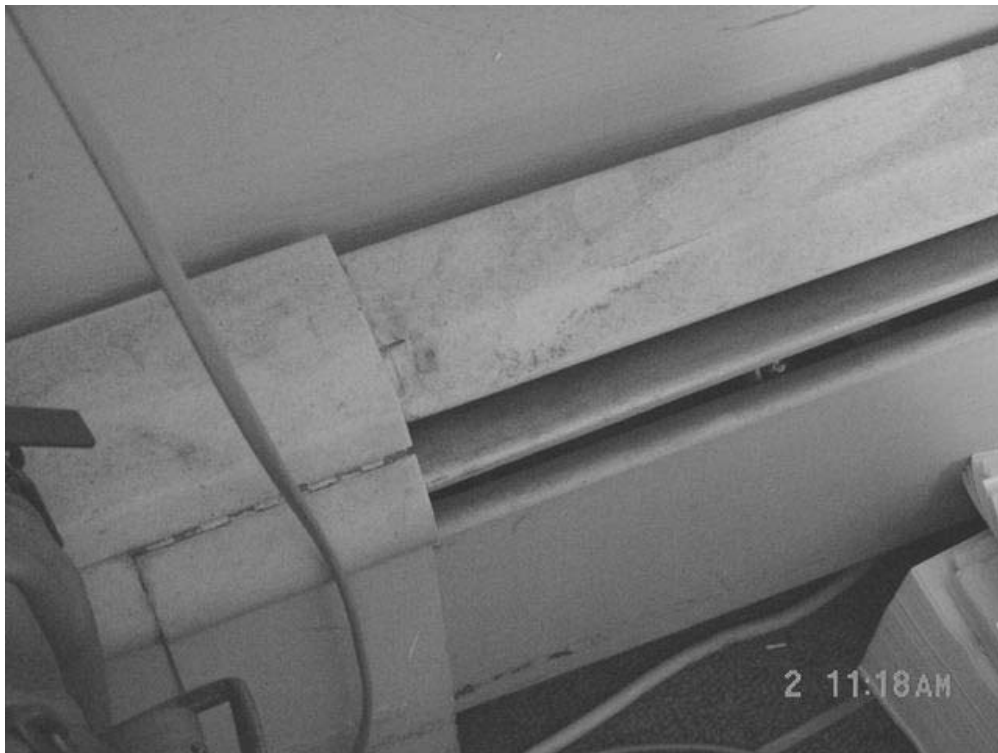
Dust Accumulation on Baseboard Heater
