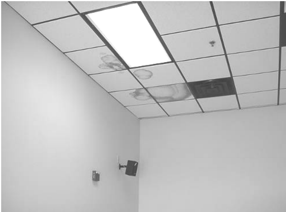
Water Damaged Ceiling Tiles in Room 210
