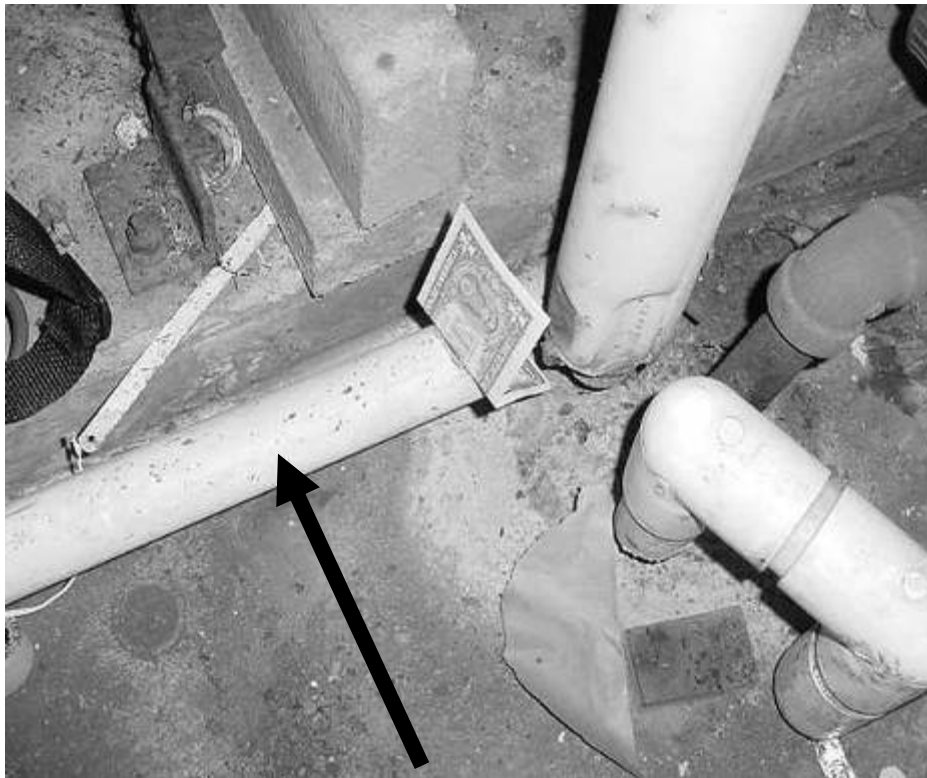
Condensation Drain Pipe
