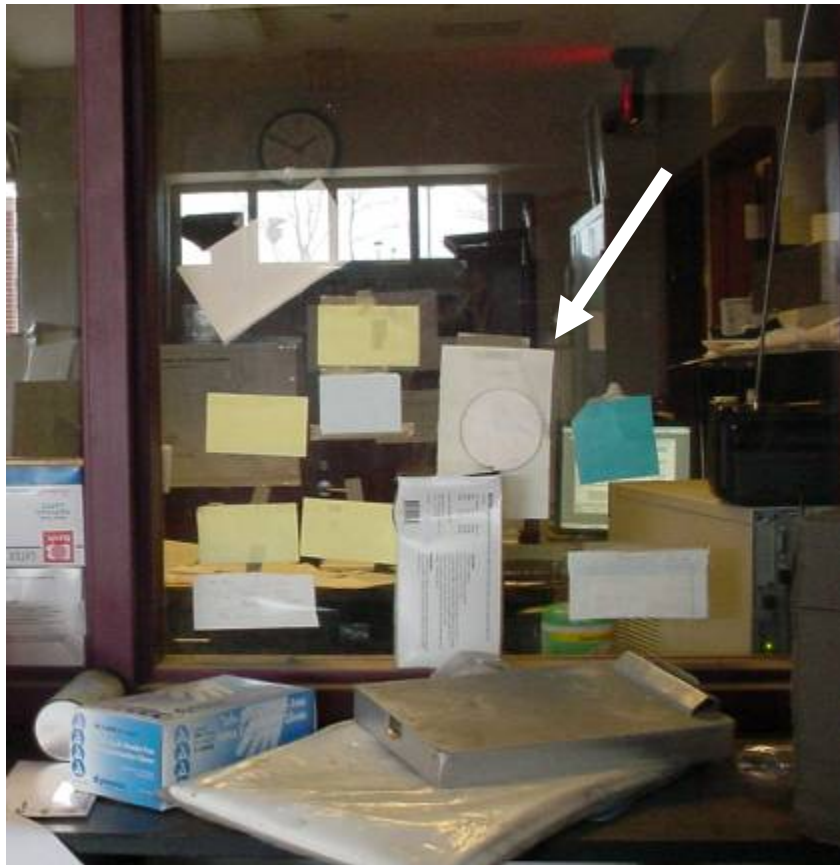
Former Check-in Window in Garage, Note Circular Opening Sealed with a Piece of Paper and Tape
