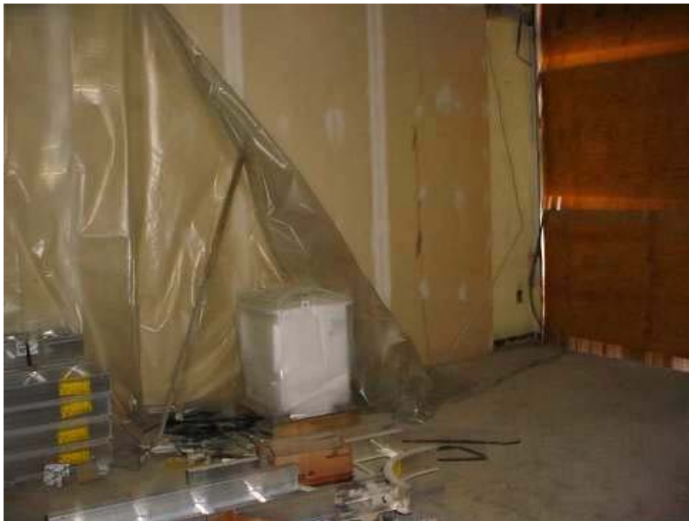
Failing Plastic Sheeting on Construction Side of Barriers
