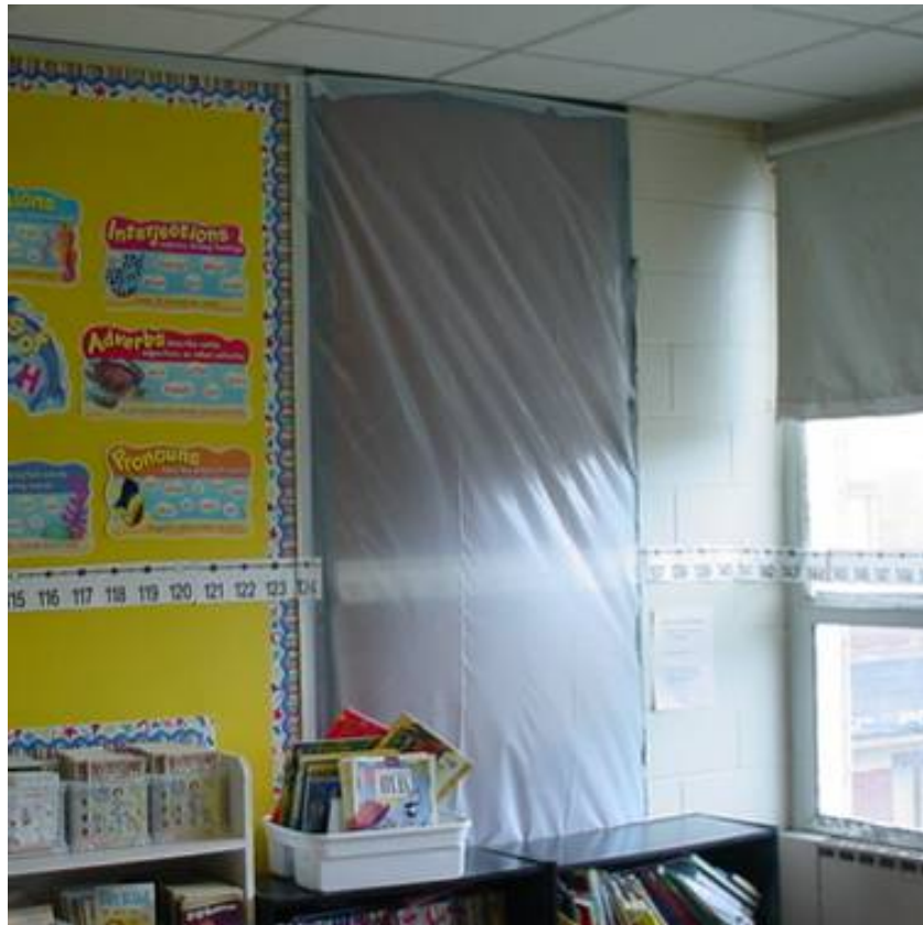
“Bowed” Plastic on Door in Classroom 33 Indicating that Construction area is Pressurized in Relation to Classroom
