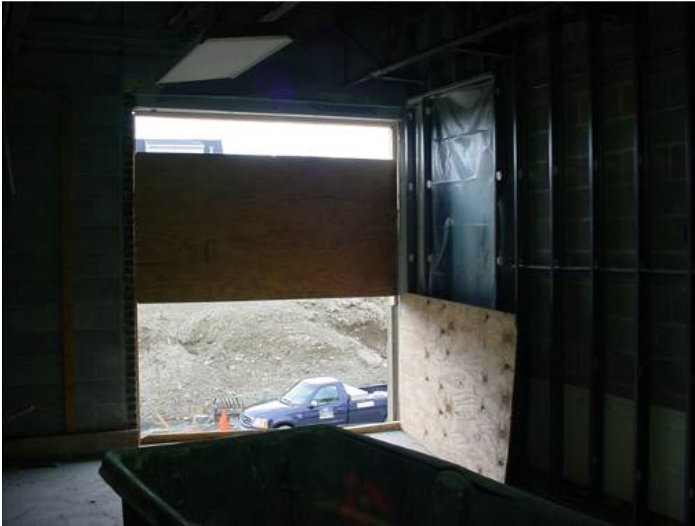
Section of Wall Removed in Construction Area Directly Adjacent to Classroom 33 Door Shown in Preceding Picture
