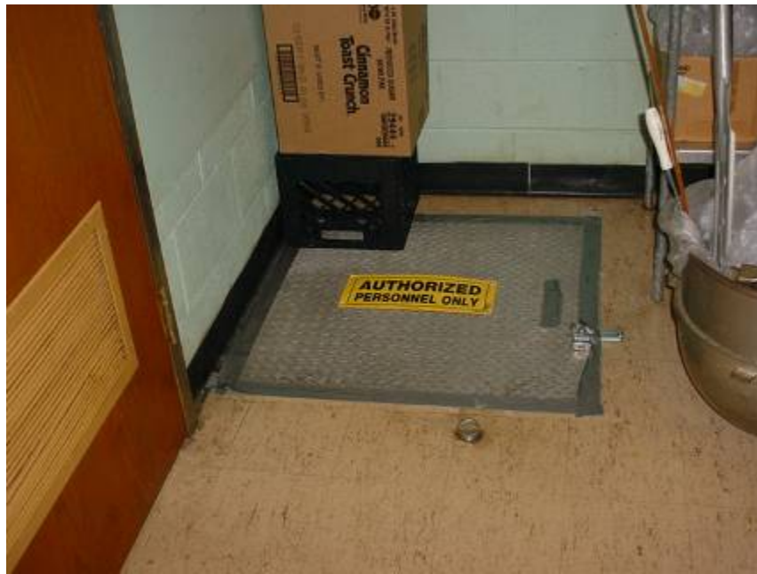
Crawlspace Access Hatch in Kitchen Sealed with Duct Tape
