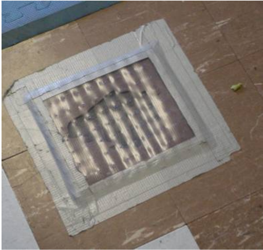
Damaged Asbestos-Containing Floor Tiles Sealed with Plastic and Duct Tape
