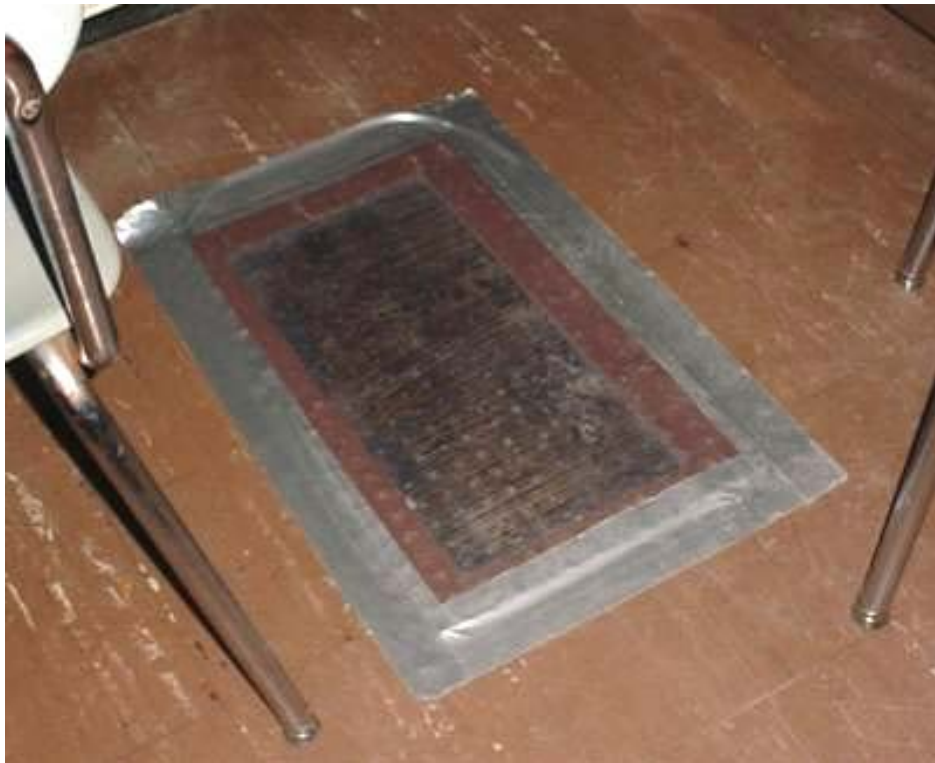
Damaged Asbestos-Containing Floor Tiles Sealed with Plastic and Duct Tape
