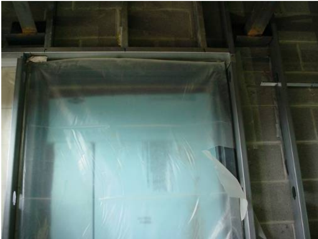
Torn Plastic Sheeting on Construction Side of Classroom Door
