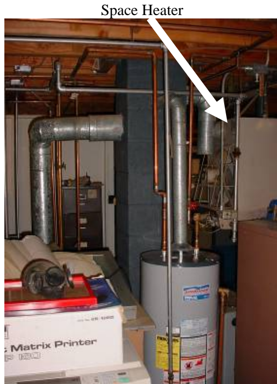
Gas Fired Water Heater, Note Space Heater Fan Location
