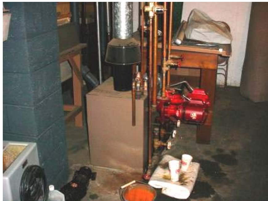
Gas Fired Furnace
