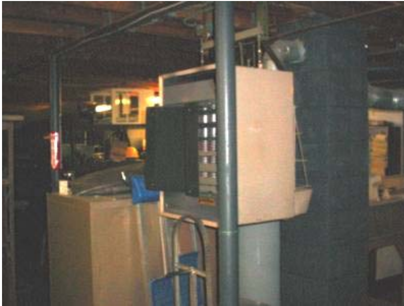
Space Heater near Furnace and Water Heater
