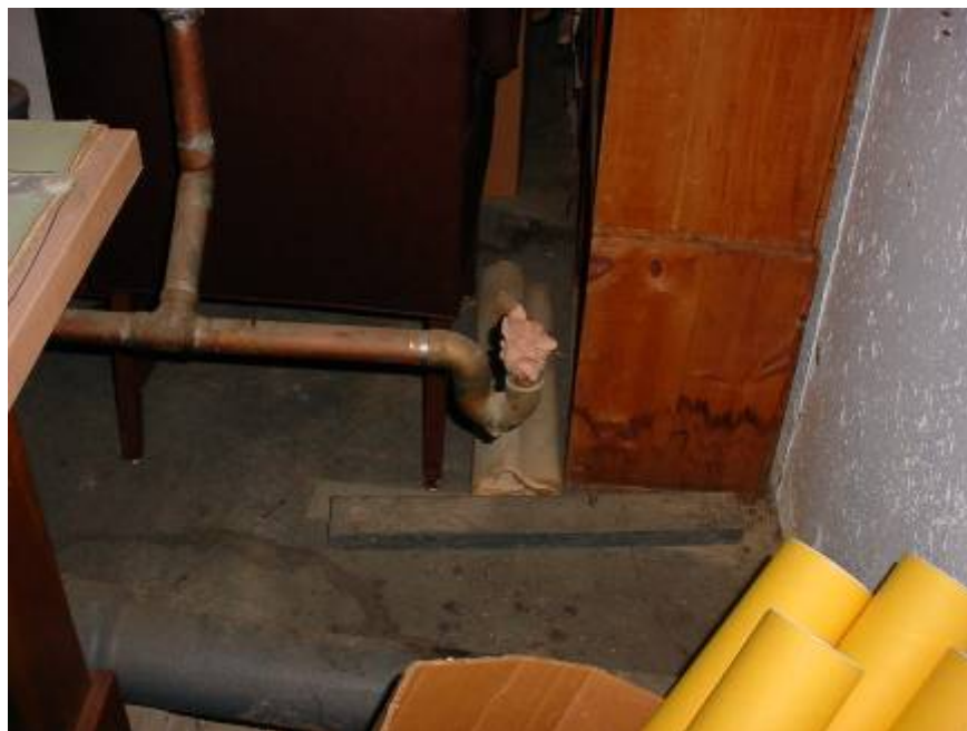
Drain Pipe Opening Sealed With Crumpled Paper
