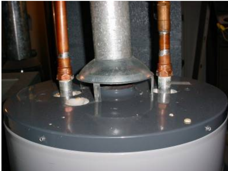
Water Heater Vent
