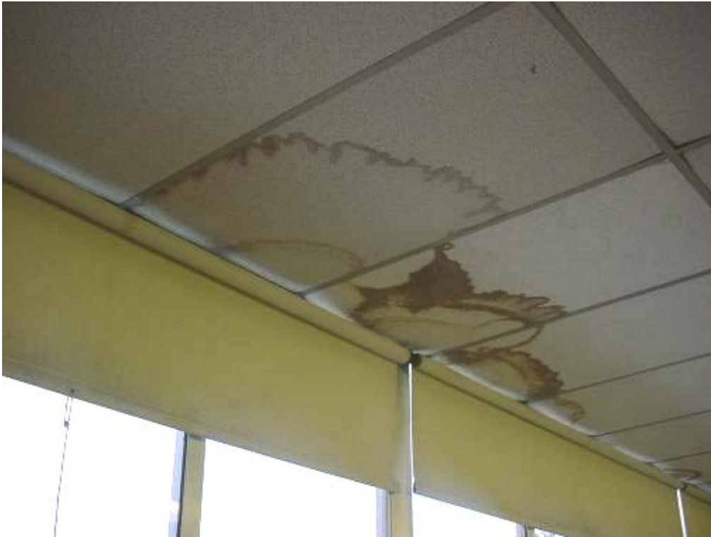
Water-damage to Ceiling Tiles along Window
