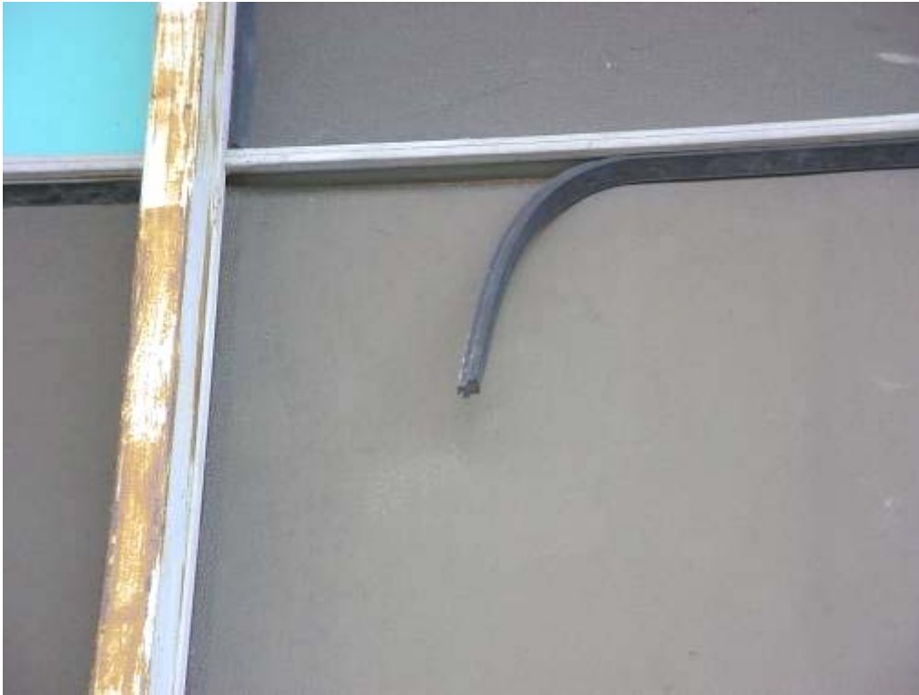
Loose/Damaged Strip Caulking
