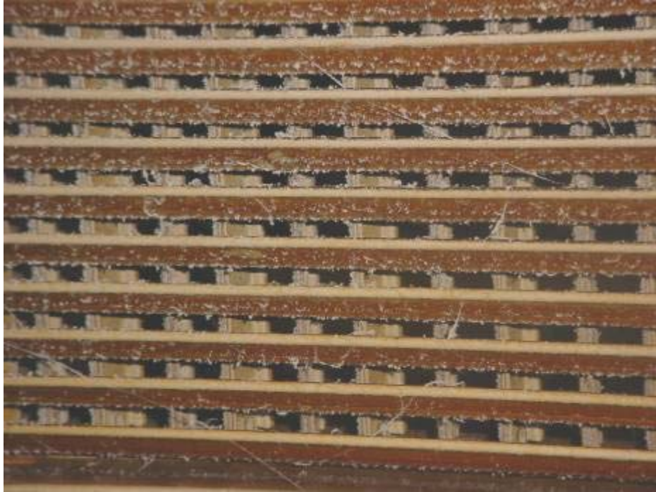
Dirty Exhaust Vent
