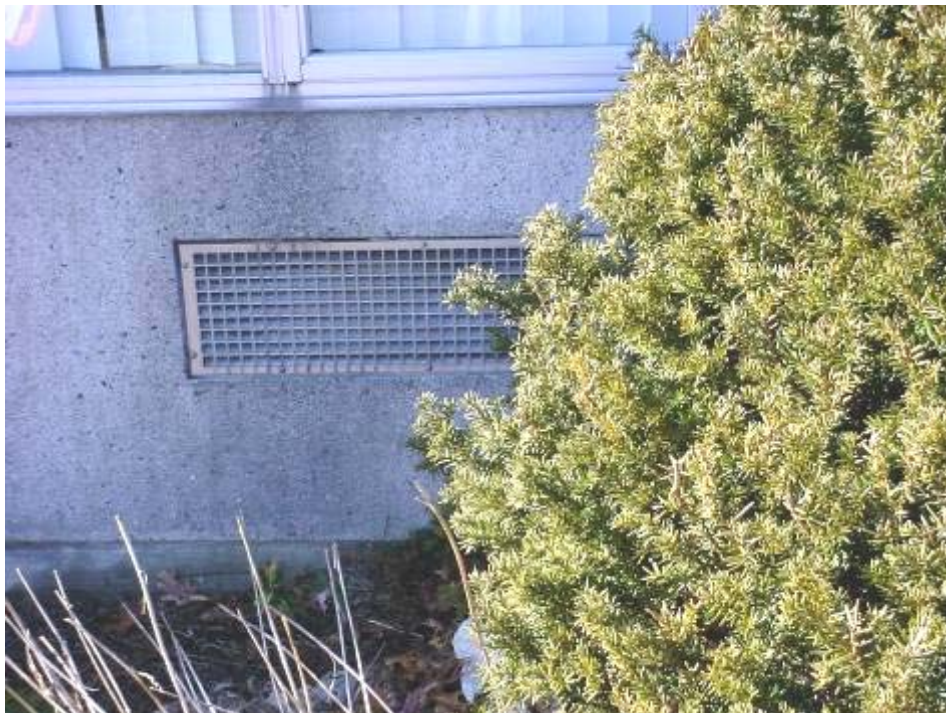
Fresh Air Intake, Note Bush Growing in Front of Intake
