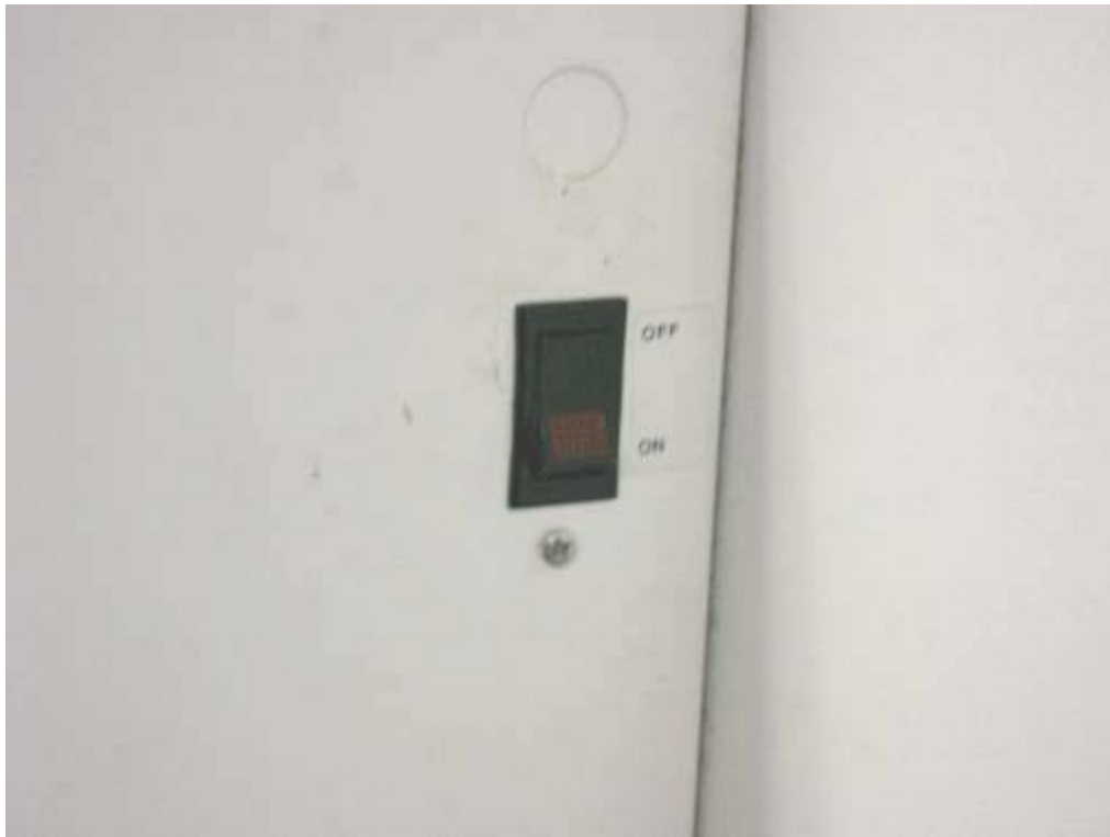
Air Handling Unit for Modular Classroom Switched to “Off”
