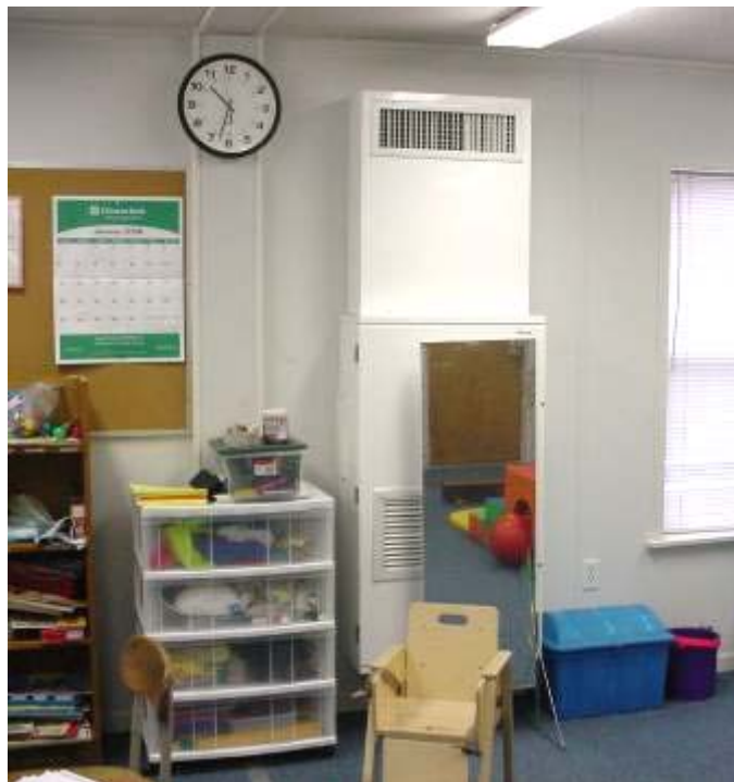
Wall-mounted Air Handling Unit, Note Mirror Blocking Vent
