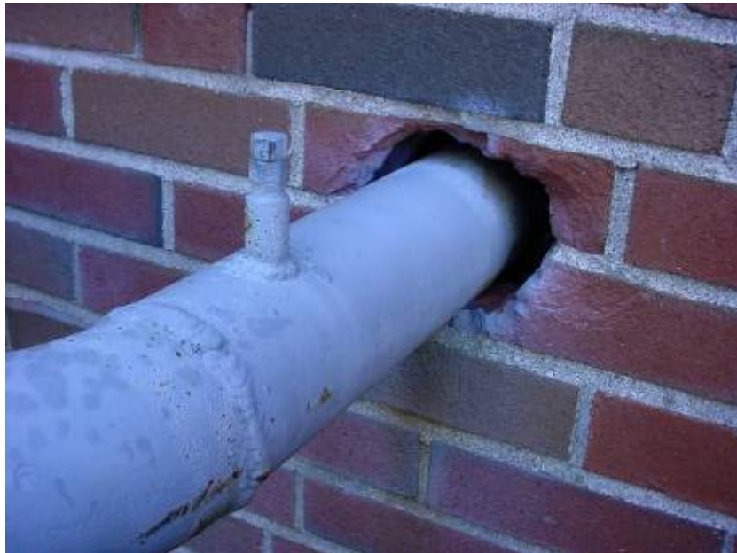
Open Utility Hole
