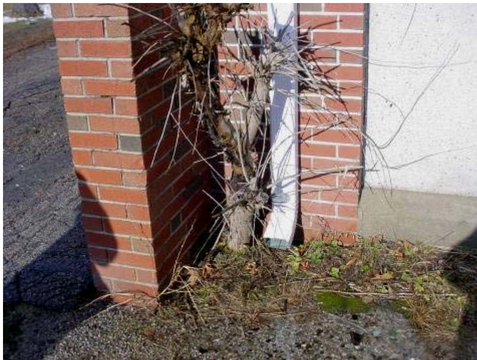
Tree Growing against Foundation/Exterior Walls
