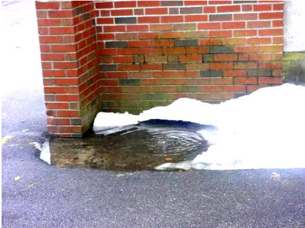
Water Pooling at Base of Building, Note Moss Growth on Exterior Wall (as Indicated by Dark Staining)
