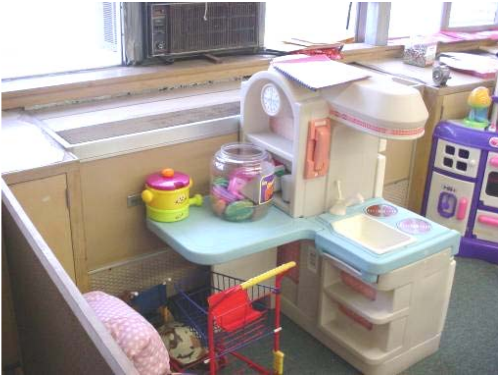
Items Obstructing Univent Return Vent (bottom front of unit)
