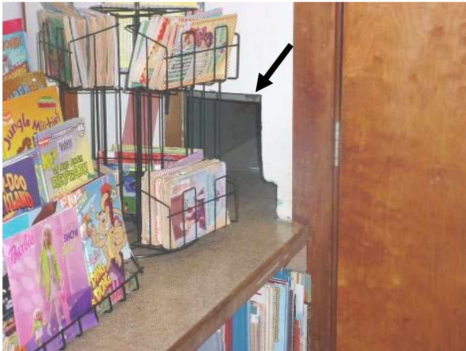
Air Supply Ducted into Library from Speech Room
