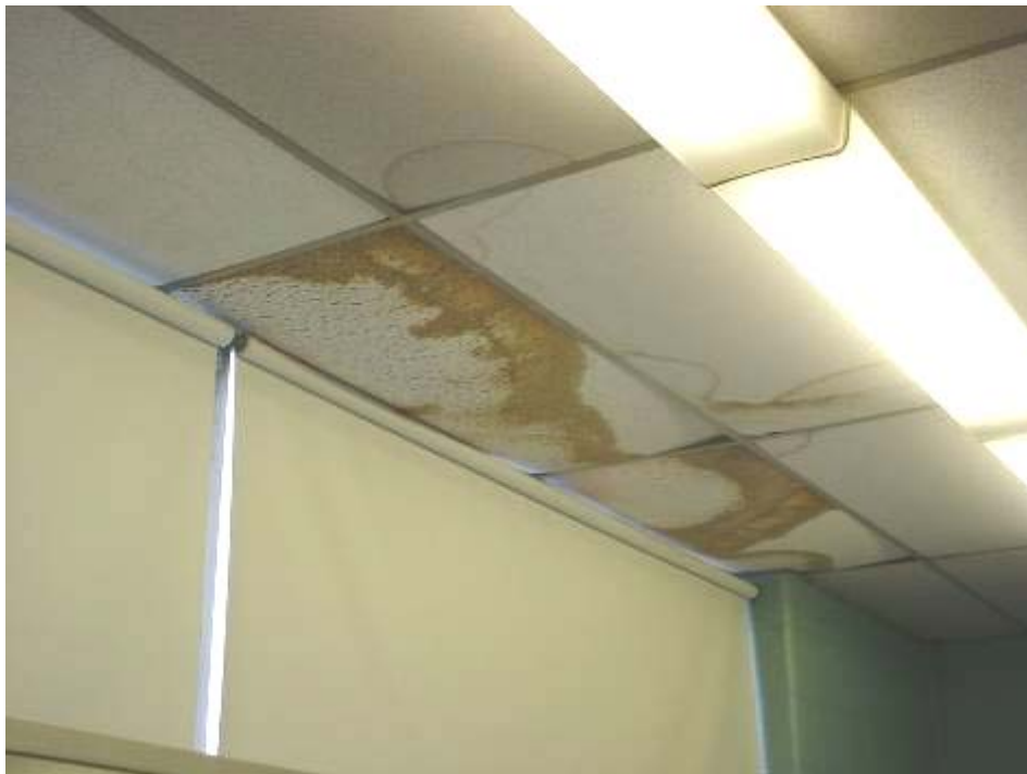
Water-damage to Ceiling Tiles along Windows
