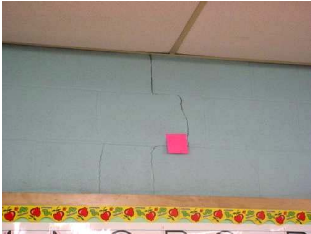
Interior Wall Crack
