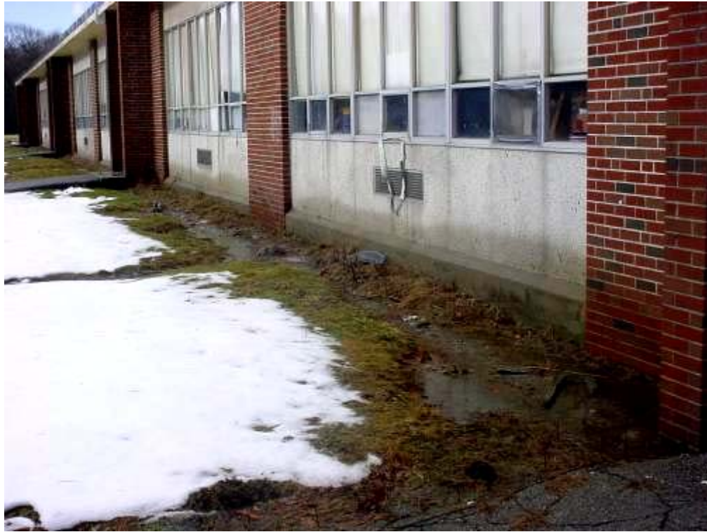
Water Pooling at the Base of Building against Exterior Wall Note Backsplash on Exterior Wall (as Indicated by Dark Staining)
