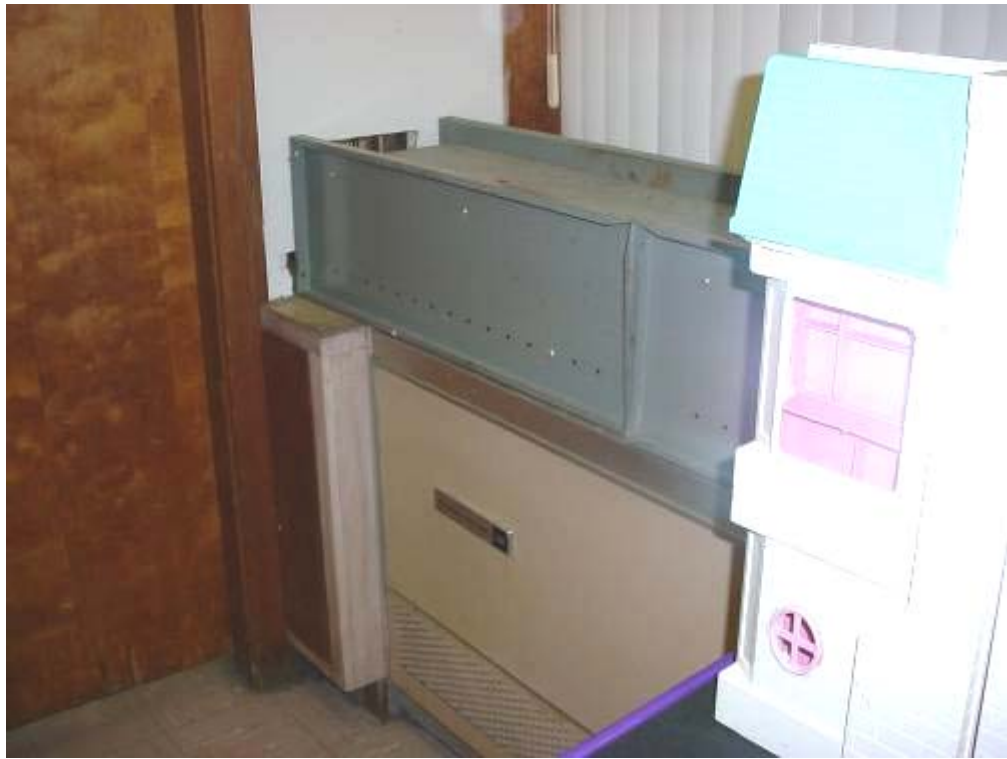
Ducted Univent Leading to Library (From Speech Room)
