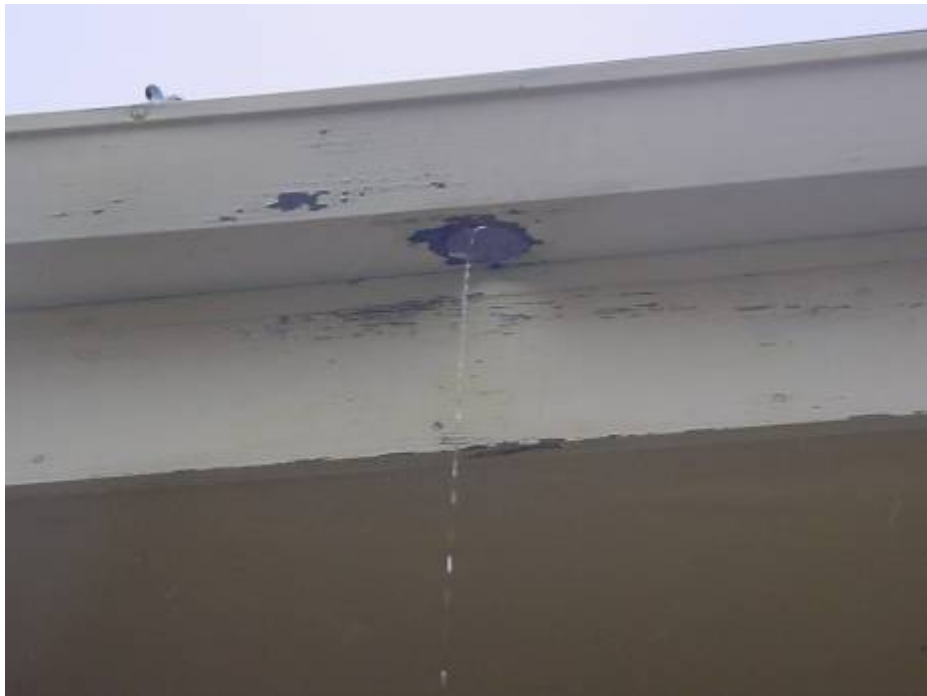
Water Emptying Against Building Hole in Gutter/Missing Downspout
