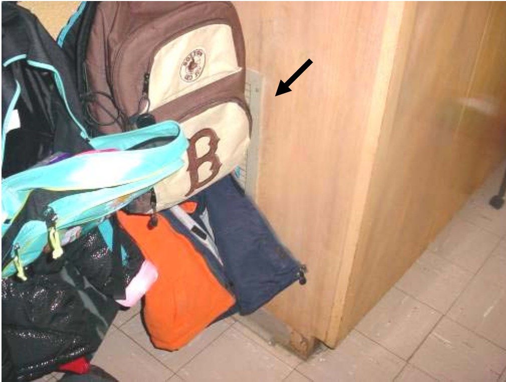
Exhaust Vent Obstructed by Coats and Bags
